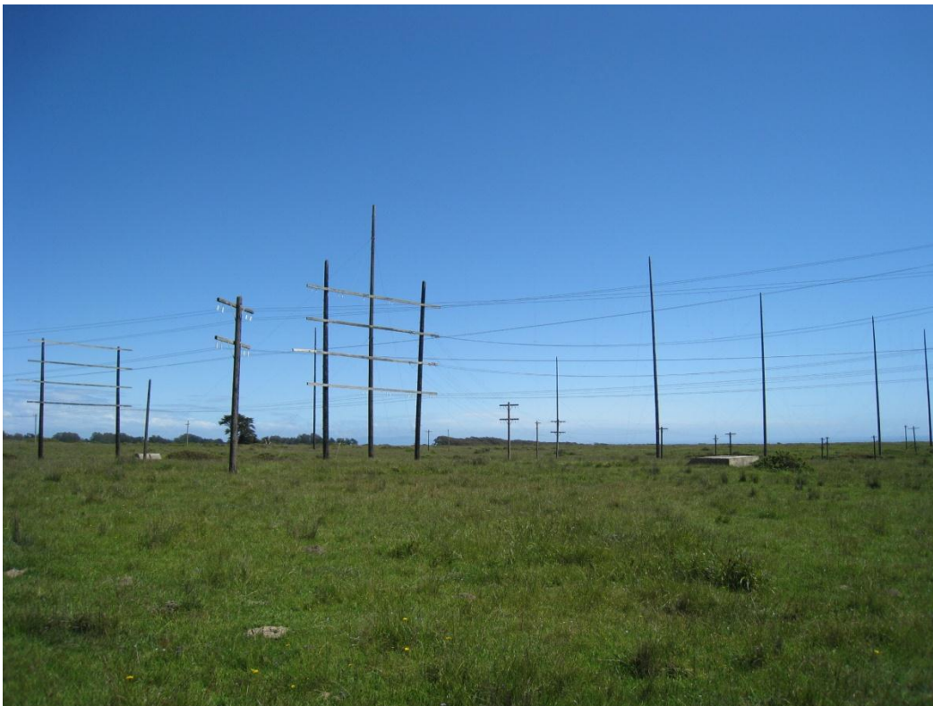
H-frames, T-poles, and various other poles and concrete bases located within the antenna field. (PWRO 2010)
