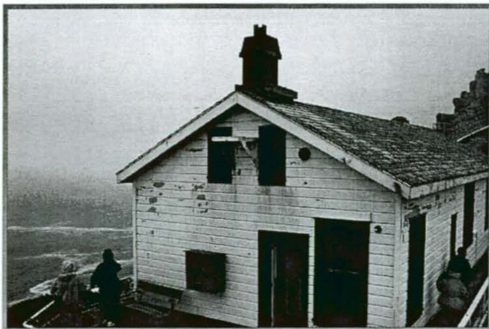
Figure 11. The west elevation of the Equipment building showing coating failure.
