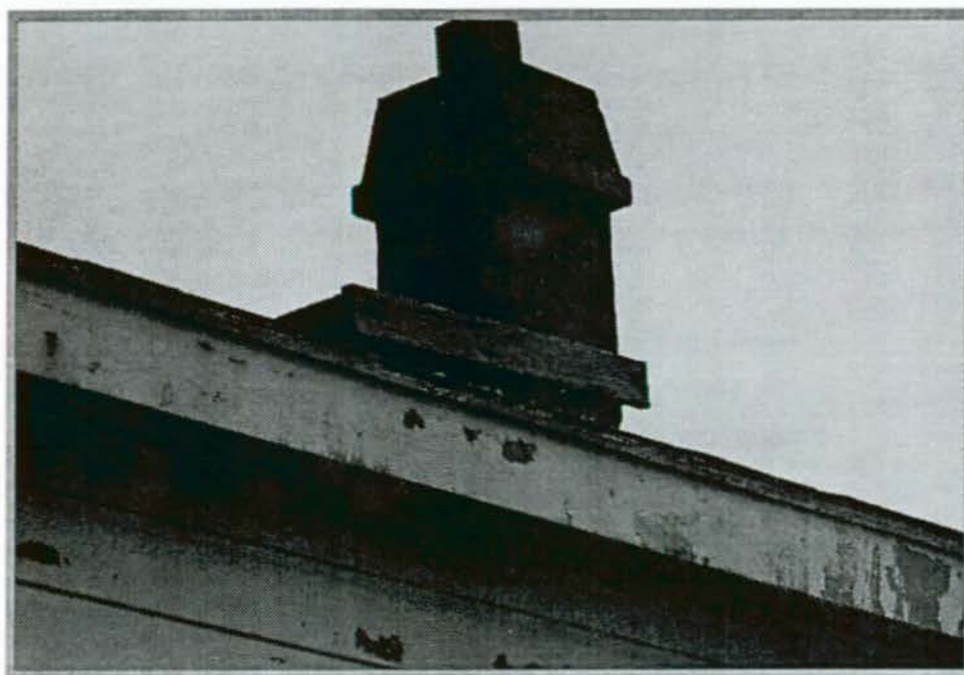
Figure 12. Coating failure at the gutters on the Equipment building.
