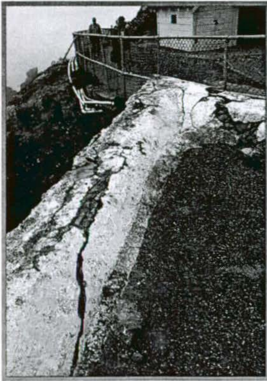
Figure 21. Crack on the top at the watershed and cistern where water is infiltrating from behind.
