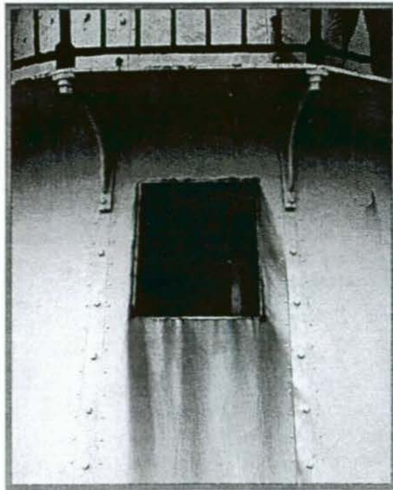
Figure 1. Rust staining under the ground level windows.
