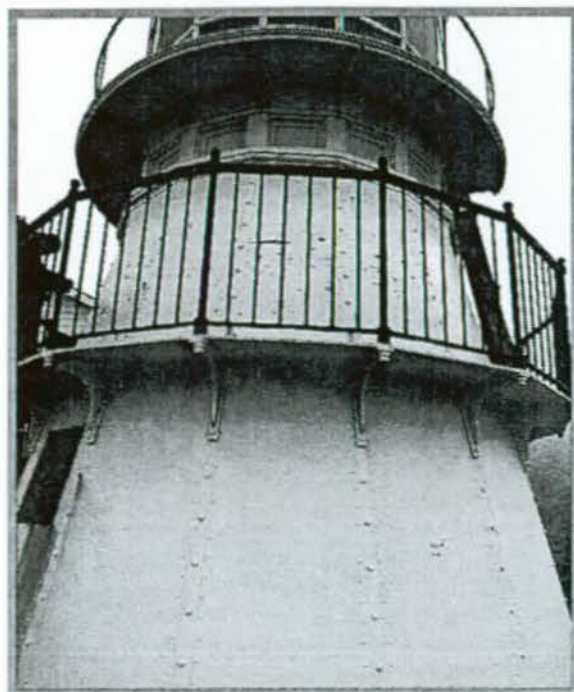
Figure 2. Through the railing, the 4'-0" and lower areas of paint loss are evident.
