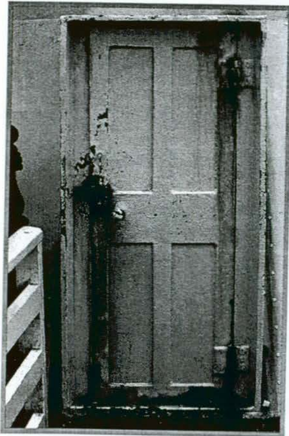
Figure 9. Signs of corrosion on the hinges, edges, and locking mechanism on the first gallery level entry door.
