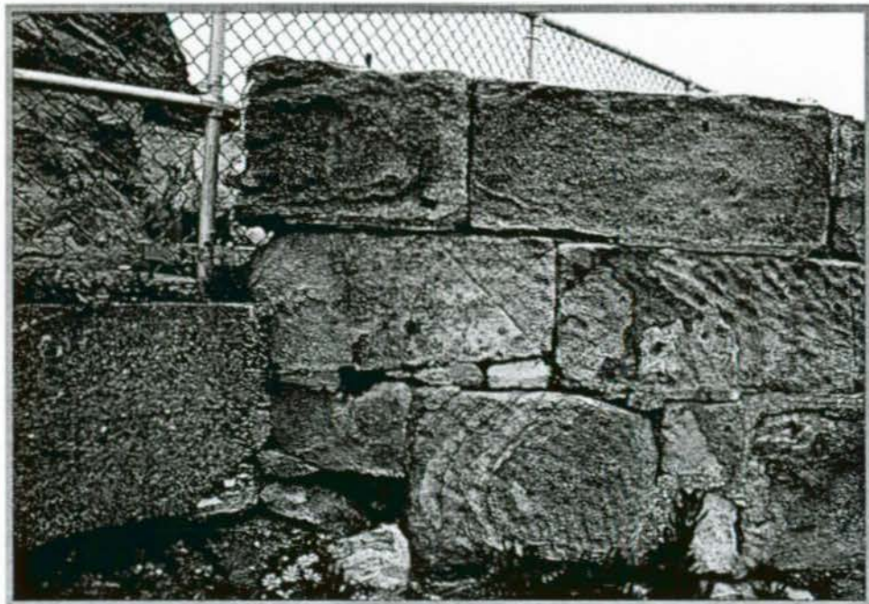
Figure 20. Far north edge of the wall illustrating where water is draining from behind and eroding edge.
