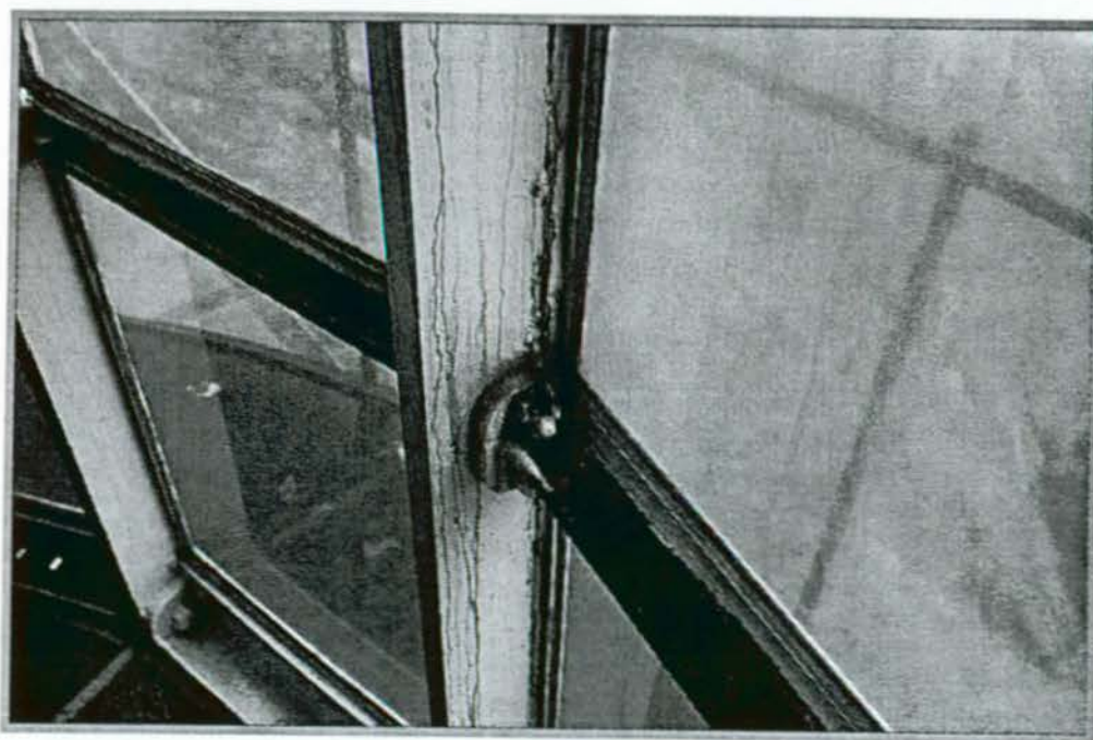
Figure 4. Rust stains and collected water on interior astragal and water trough.
