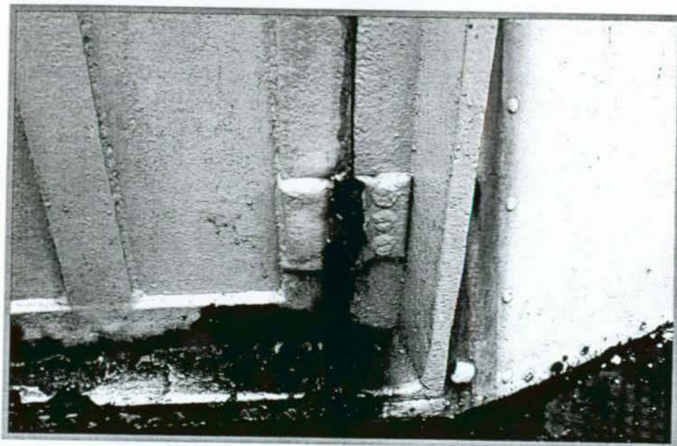
Figure 10. Rust on the bottom hinge of the first gallery entry door.
