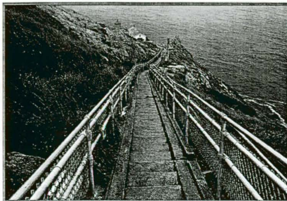
Figure 16. A missing curb section on the right side of the stairway.
