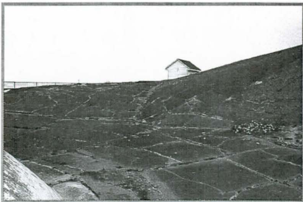
Figure 23. View of cistern, in lower left, and watershed showing severe cracking, elastomeric joints, and plant invasions.
