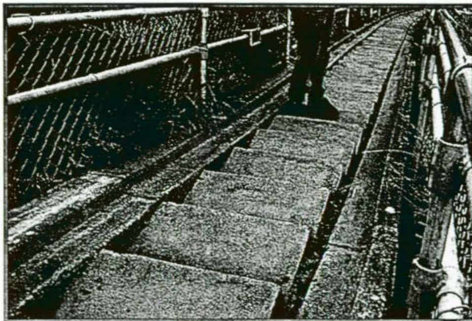
Figure 15. A greater than 3/8" separation between the stair and curb.
