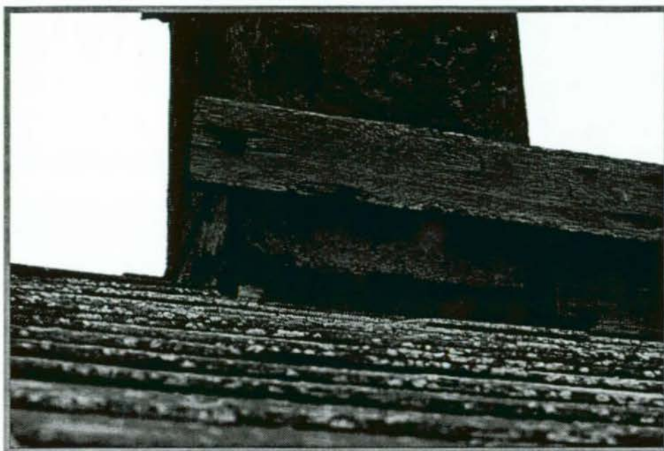
Figure 13. Joint at chimney where water flashing has fallen away.
