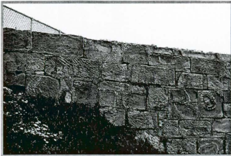
Figure 22. Previous patches are spalling along with original stone face.
