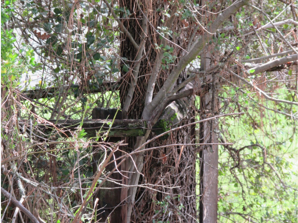
Buildings and Structures #3 Close-up of the damaged Horace Bacon Commemorative Tree Enclosure. (NPS, March 2020)
