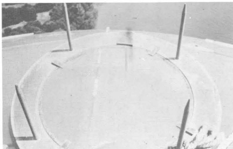
ILLUSTRATION 243. Lightning points on top of lantern hatch.
