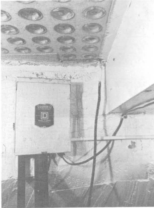
ILLUSTRATION 239. Lantern lighting panel at elevator machine platform.
