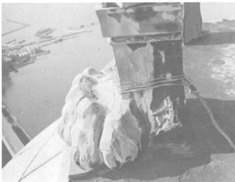
ILLUSTRATION 244. Typical (unacceptable) grounding of lantern base.
