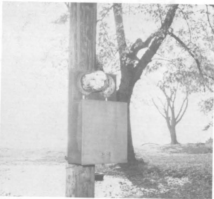
ILLUSTRATION 220. Ohio Edison Company Electric Meter.
