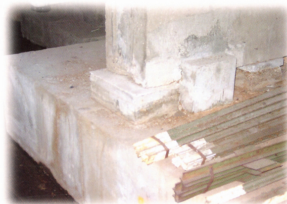
Photo of a concrete block used to jack up the structure, which is settling into the landfill.
