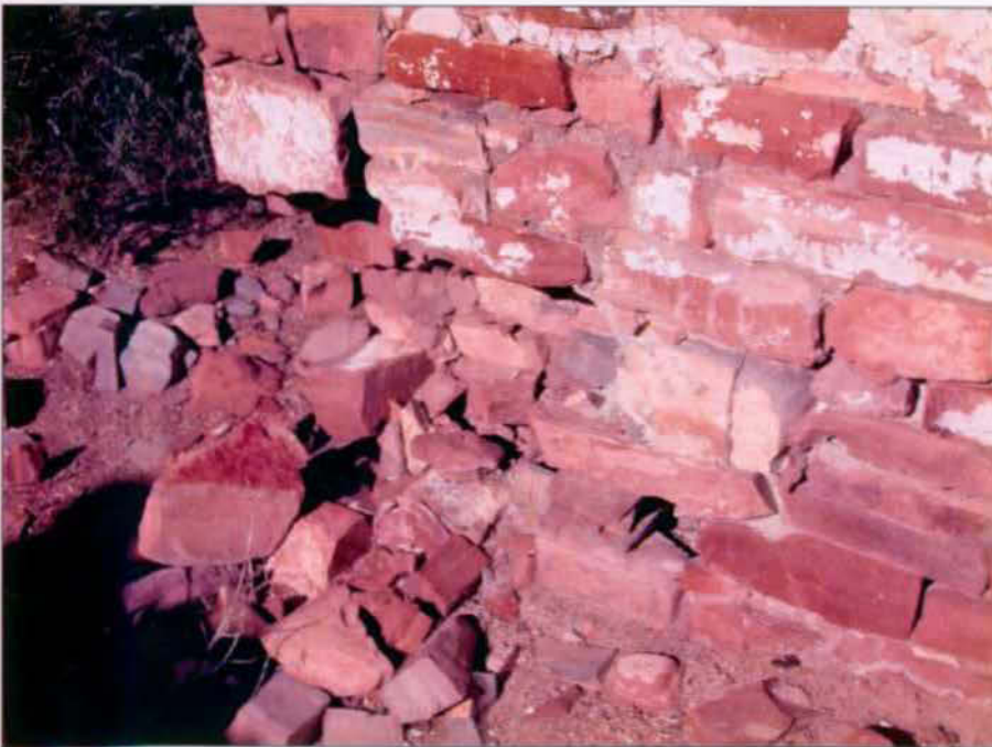
Detail at collapse of base of wall below arched opening.
