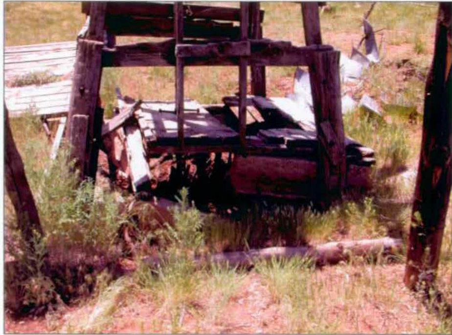
Detail of well below windmill. Note deteriorated concrete enclosure and deteriorated wood cover.
