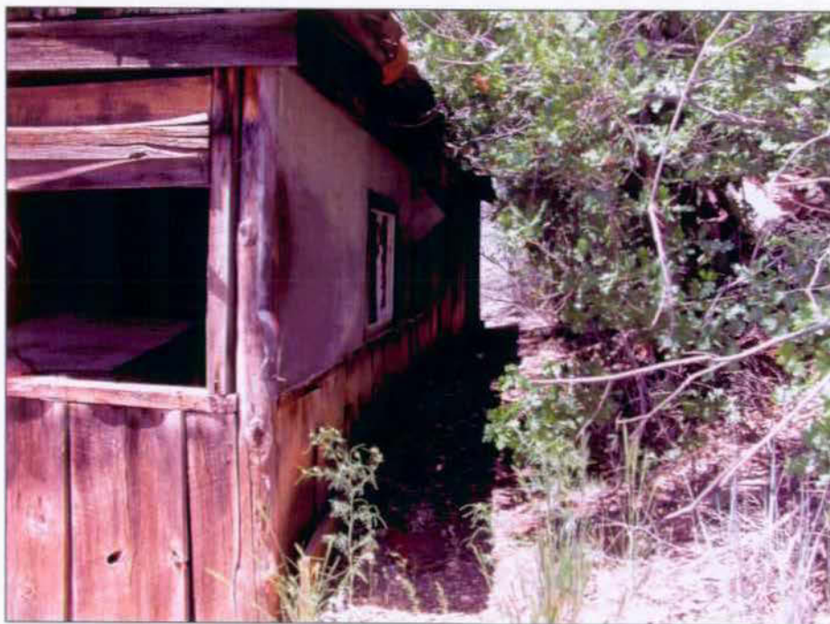
Detail of northeast corner. Note sedimentation along north wall.
