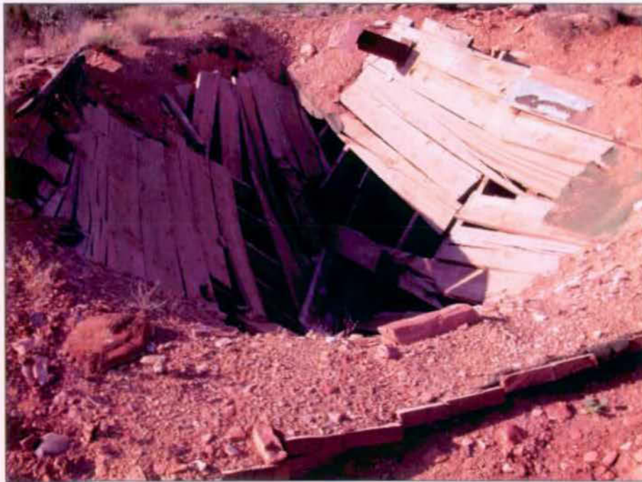
View from northwest. Note collapsed roof.
