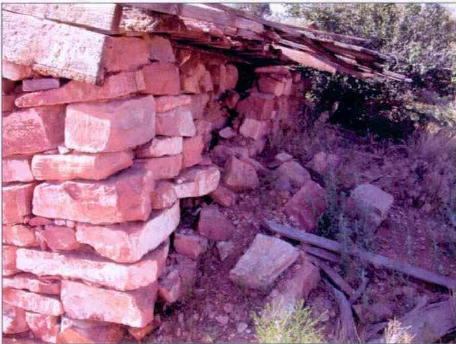
Detail of northwest corner of building. Note erosion and collapsing wall (outer wythe”).
