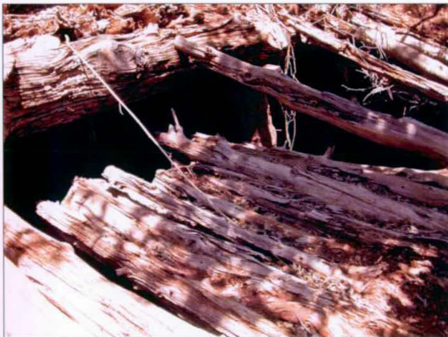
Detail of roof. Note center beam and collapsed roof poles.
