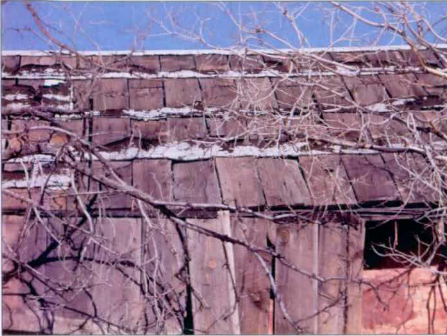
Detail of roof covering, sheathing, and collapsed porch roof.
