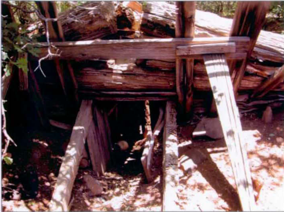
View from south. Note bracing holding up south wall.
