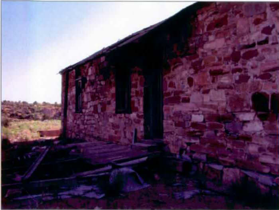
Detail of west wall and partially collapsed roof and porch floor.
