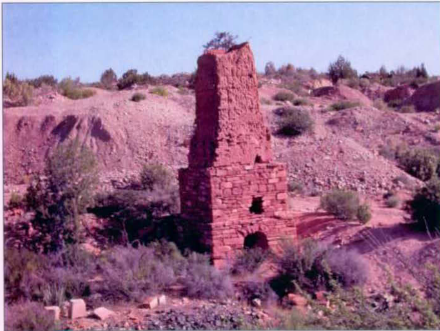
View from southwest. Note holes in masonry above arch and in adobe above stone base, and erosion of step in adobe chimney.
