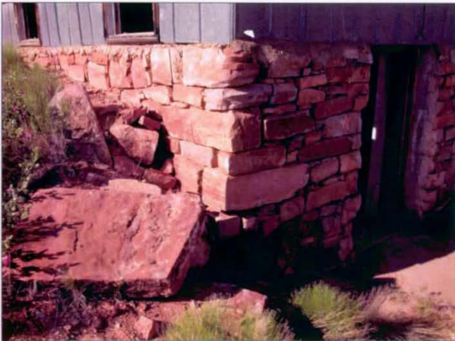
Detail of northeast corner of building. Note eroded wall at lower corner.
