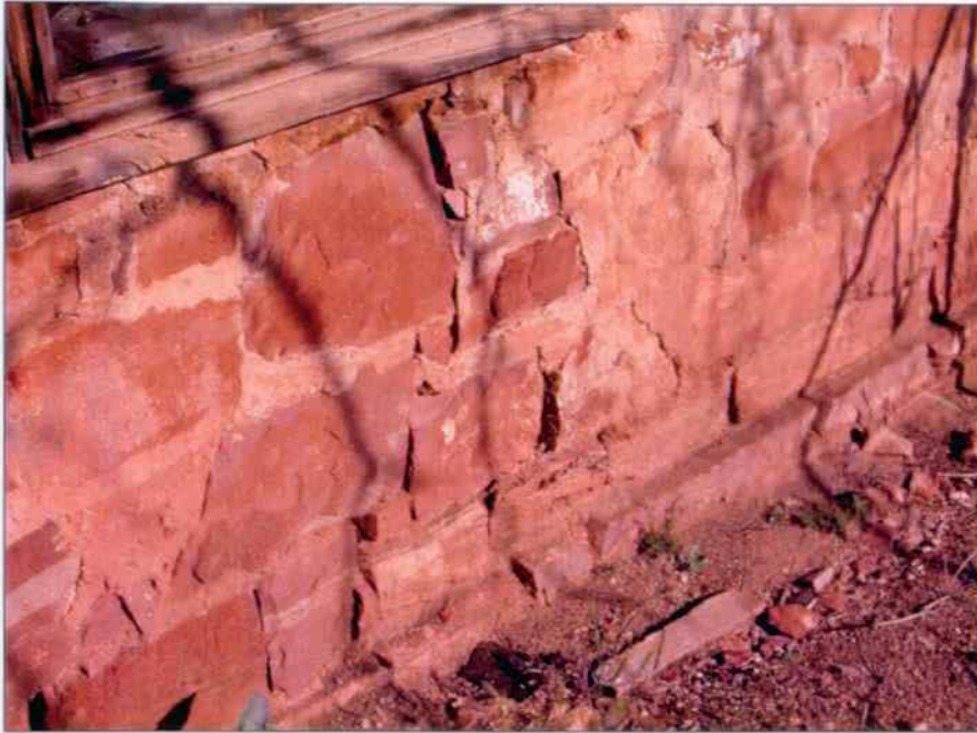
Detail of mortar joints in east wall. Note eroded and re-pointed mortar joints.
