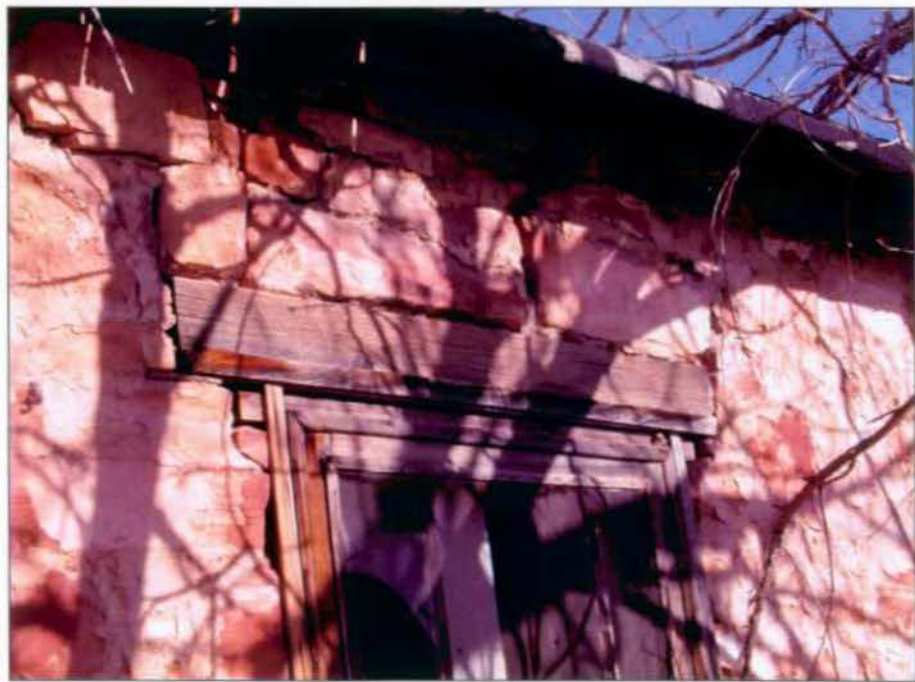
Detail of cracking and eroded mortar joints in east wall.
