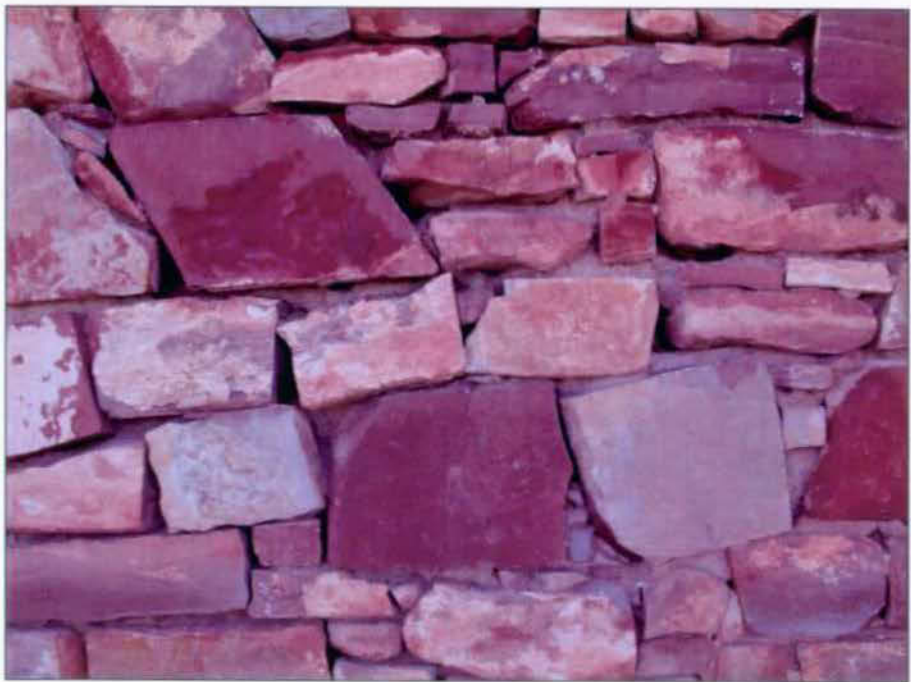
Detail of eroded mortar joints in east wall.
