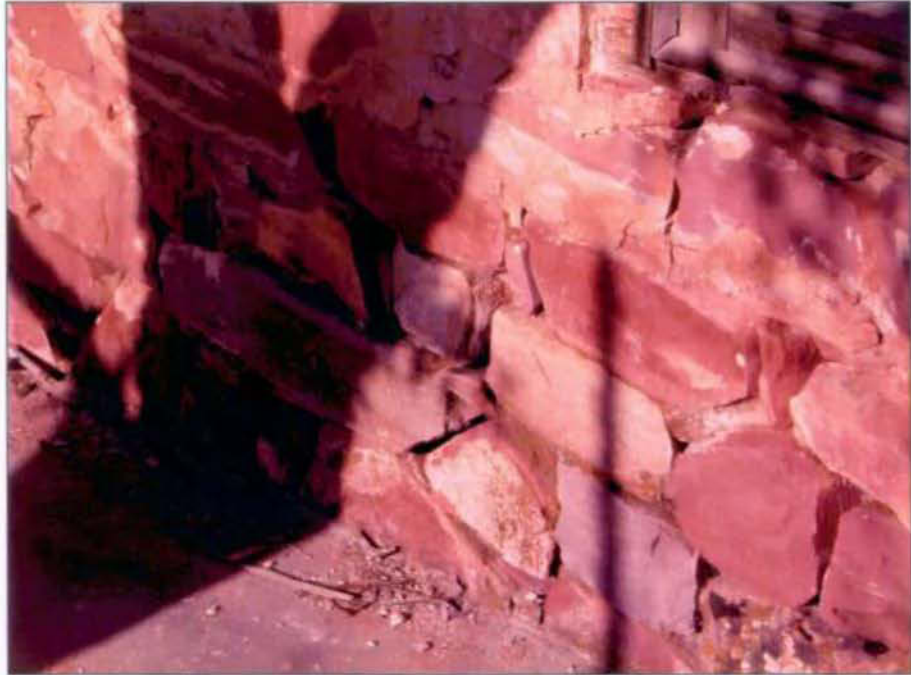
Detail of east wall. Note eroded mortar joints.
