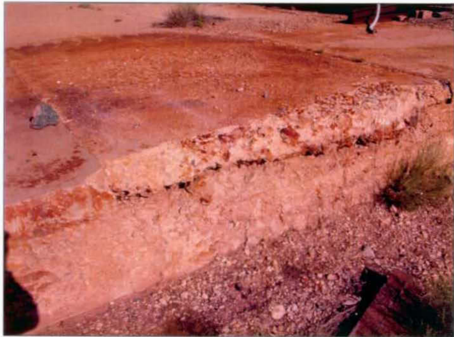
Detail of east edge. Note deterioration of concrete at edge.
