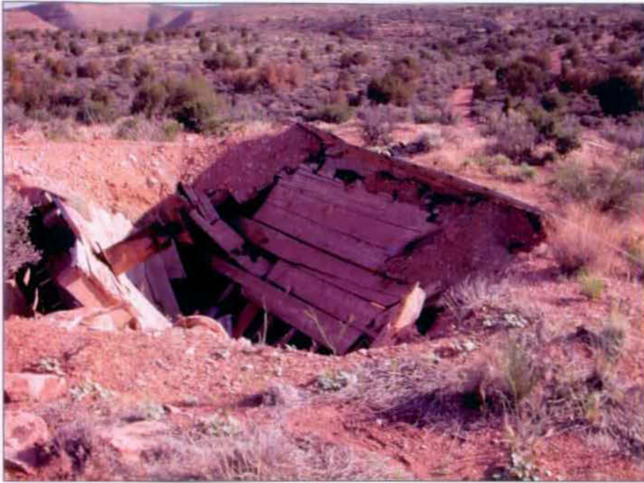
View from southeast. Note collapsed roof
