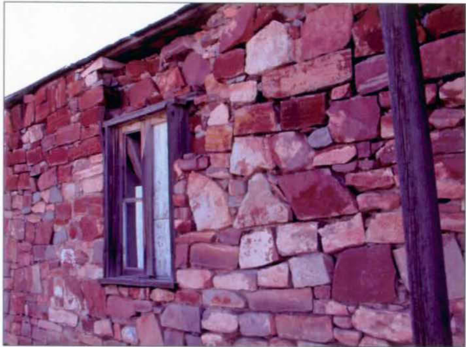
Detail of east wall. Note eroded mortar joints and missing stones over window.
