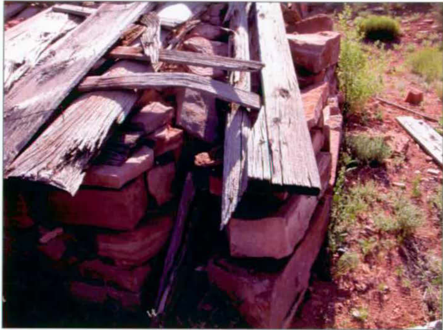
Detail of southwest corner. Note corner separation, collapsed roof structure, and "orrilas" in roof below.
