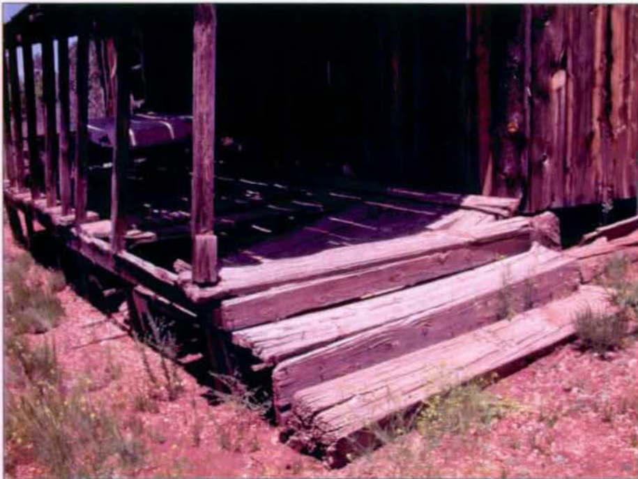
Detail of west end of porch. Note deteriorated steps and flooring, and displaced framing.
