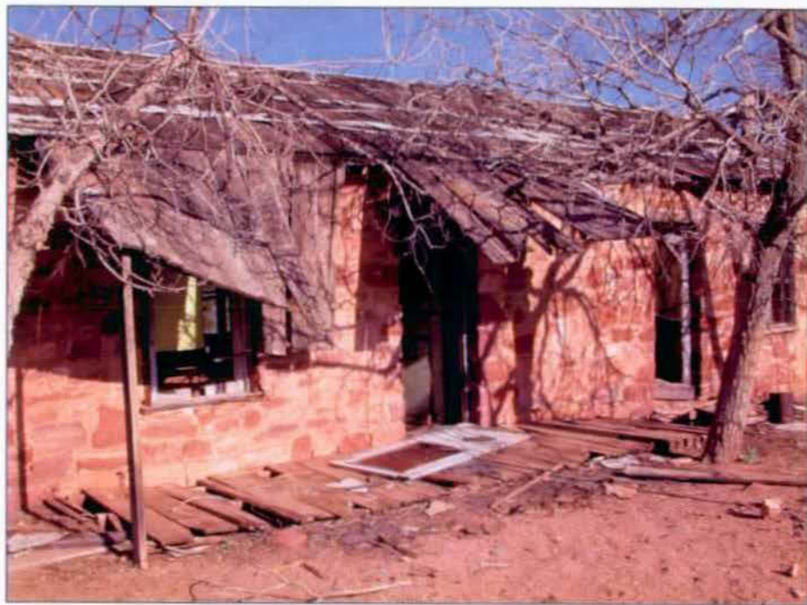
Close-up of east elevation. Note partially collapsed porch roof, and deteriorated porch floor.
