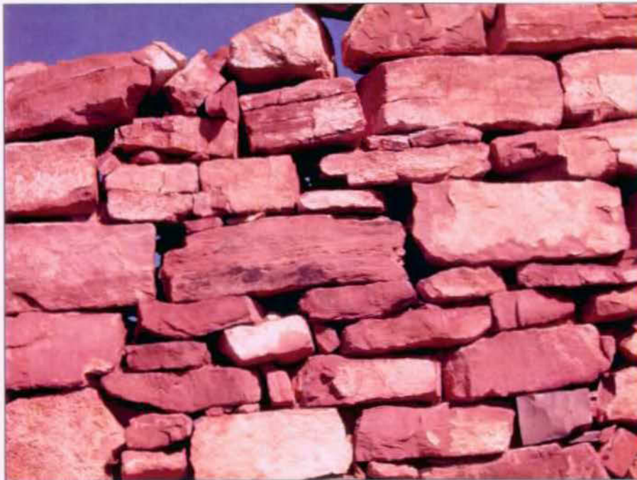
Detail of cracked wall at southeast corner.
