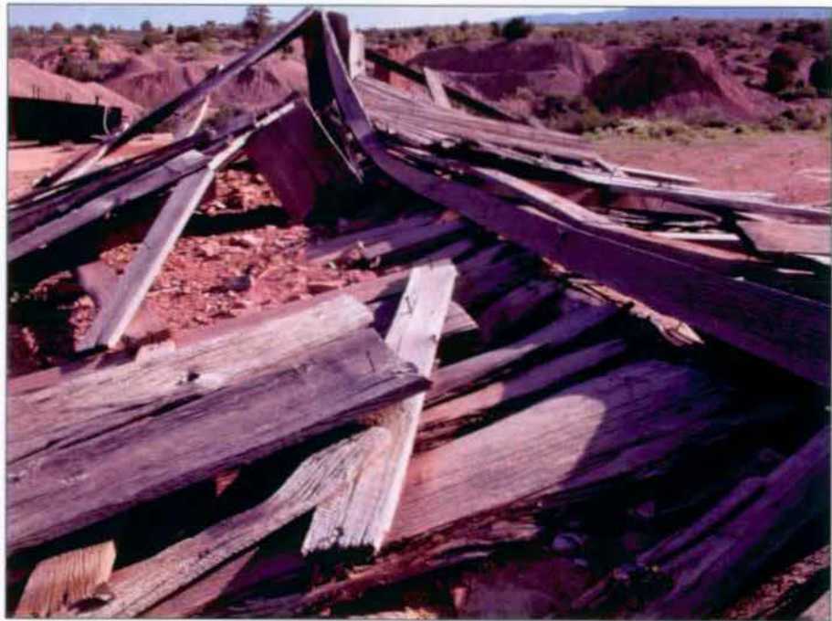
Detail of roof. Note original roof under collapsed secondary roof and earth covering.
