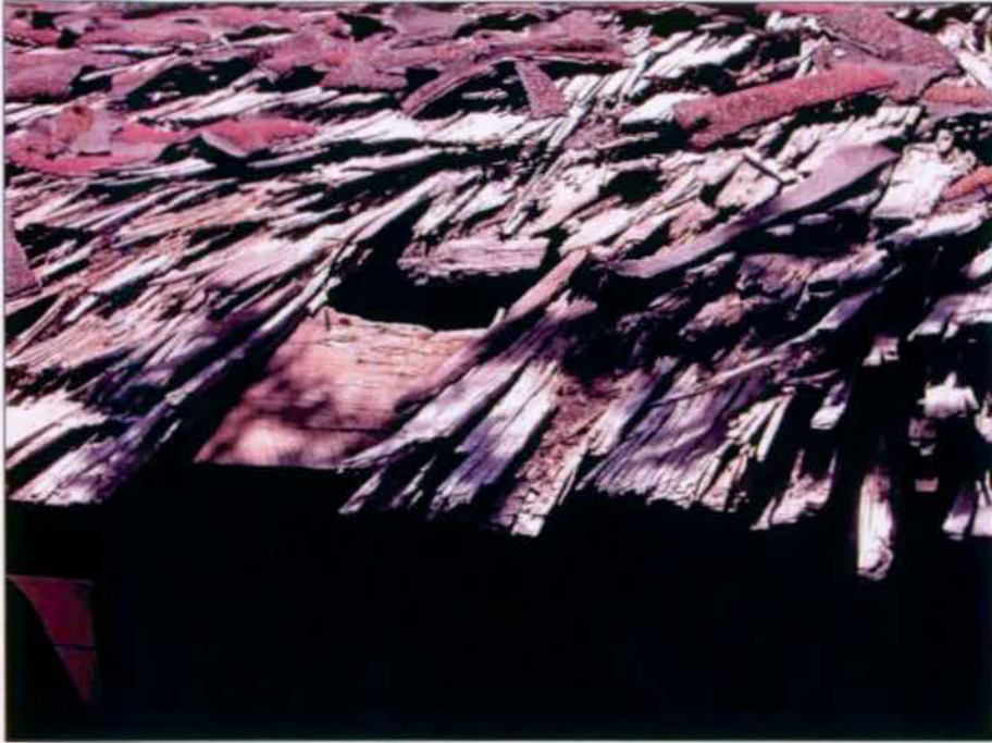
Detail of deteriorated roofing.
