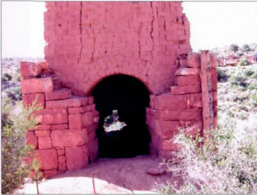
Detail of north elevation. Note adobe arch and missing stone arch.
