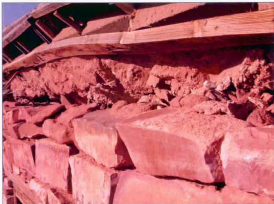
Detail of east wall. Note how roof collapse has rotated framing and associated construction up off of top of wall.
