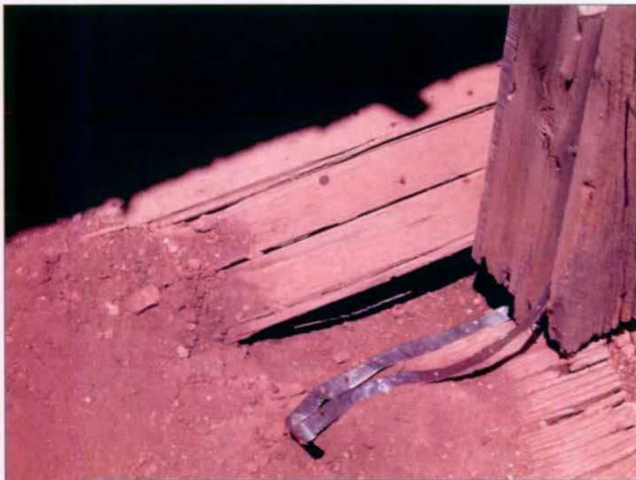
Detail of deteriorated flooring and door sill at north end of east elevation.
