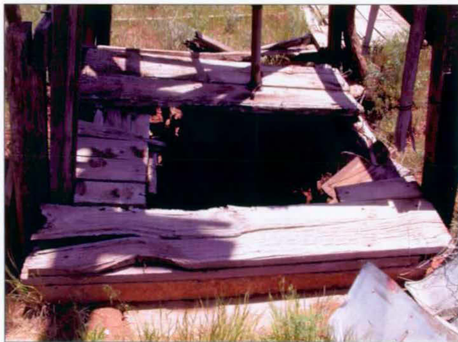
Detail of well below windmill. Note concrete enclosure and deteriorated wood cover.
