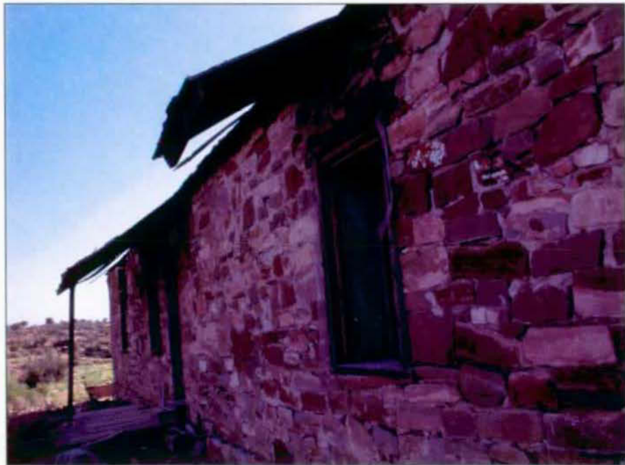
View of west wall. Note unsupported roof over window, and partially collapsed roof over porch.
