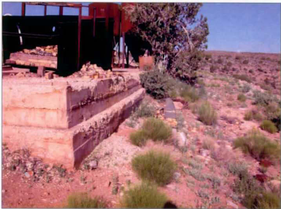
Detail of northeast corner. Note deterioration of concrete at edge.
