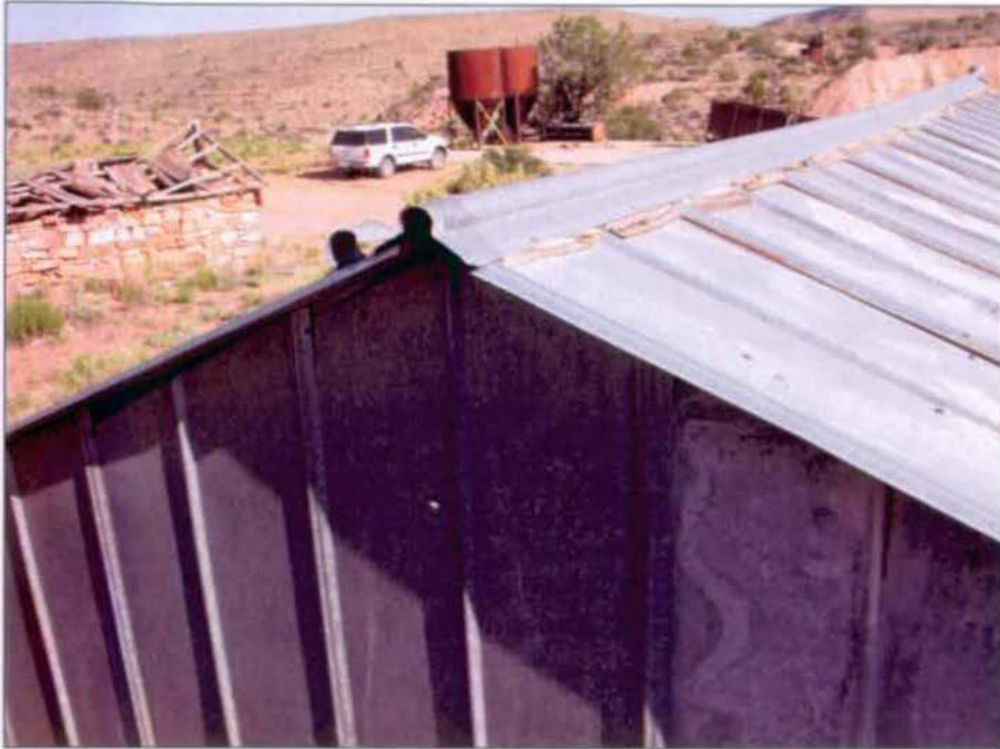
Detail of south end of roof. Note missing end trim piece, and pieces of wood boards jammed under ridge cap.
