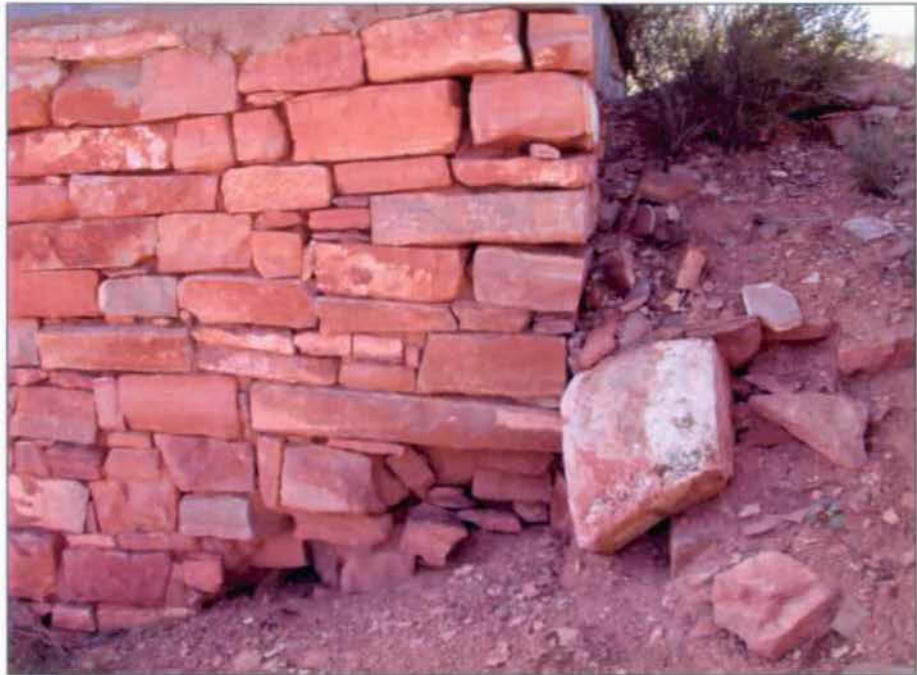
Detail of northwest corner of building. Note eroded wall, and missing stones.
