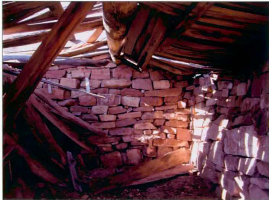
Detail of interior. Note collapsing roof and walls.
