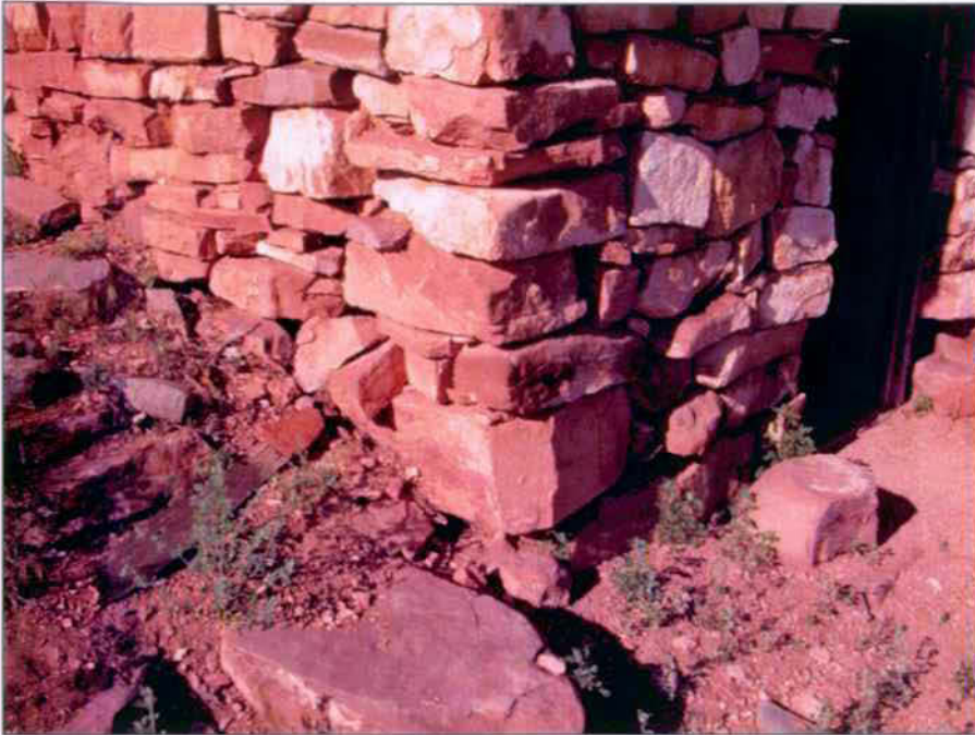
Detail of northeast corner of building. Note erosion and missing stones.
