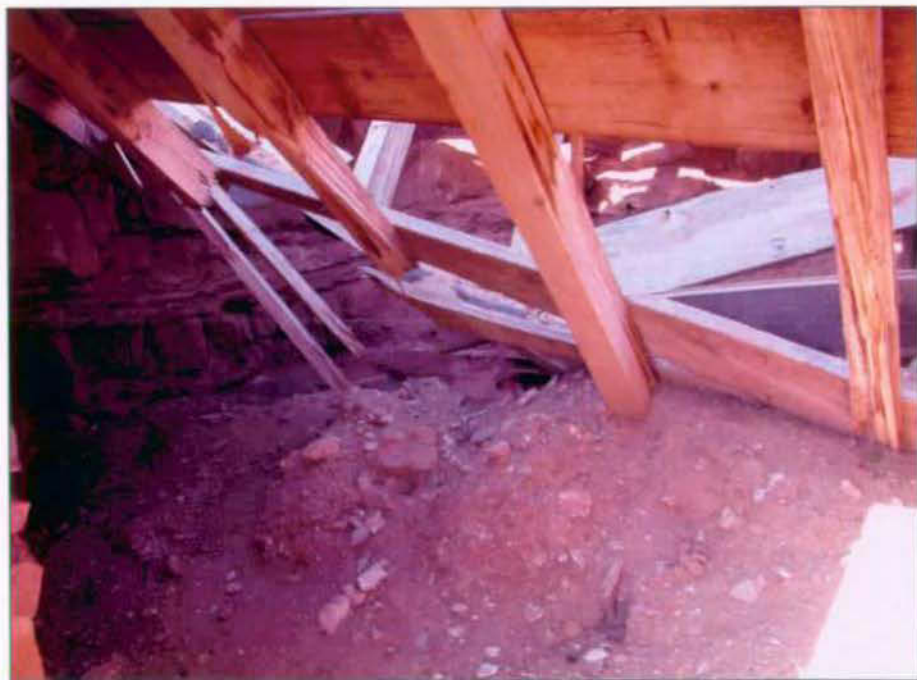
View if interior. Note collapsed roof and sediment on floor.
