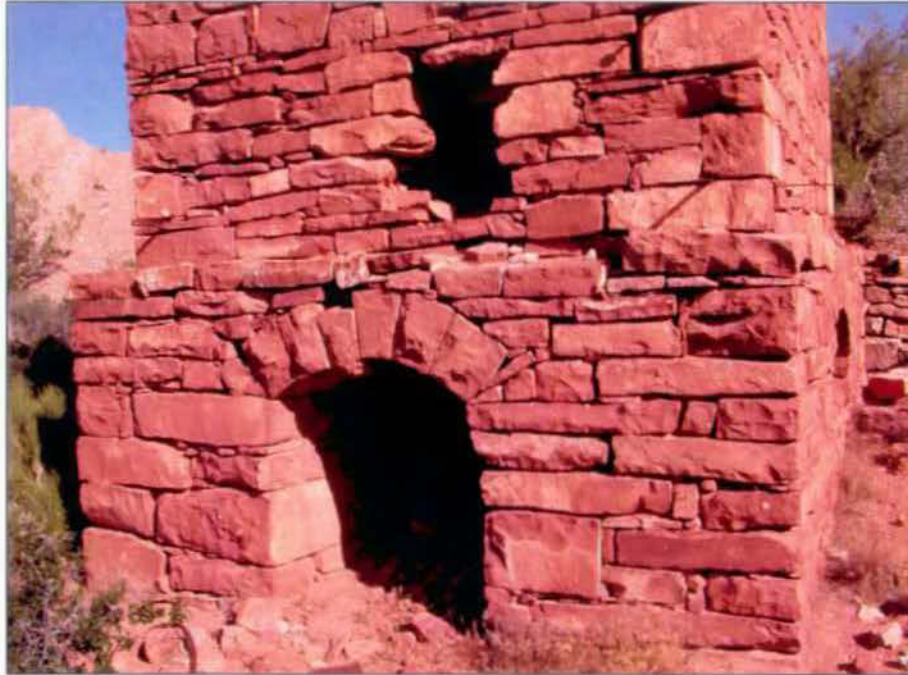
Detail of south elevation. Note hole in masonry above arch, deterioration at top of first tier, and loose stone in arch.
