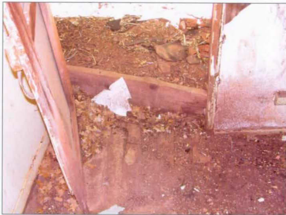
Detail of door sill at north wall (room 3). Note sedimentation, and board to prevent sediment from entering building.
