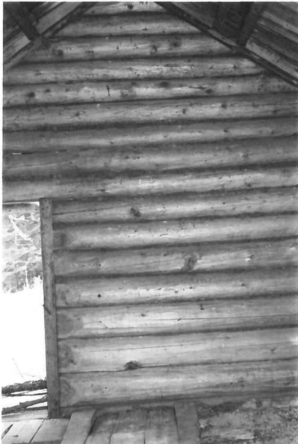
Illustration No. 12: View of interior toward front entrance. Note decay of floor construction from contact with earth.
