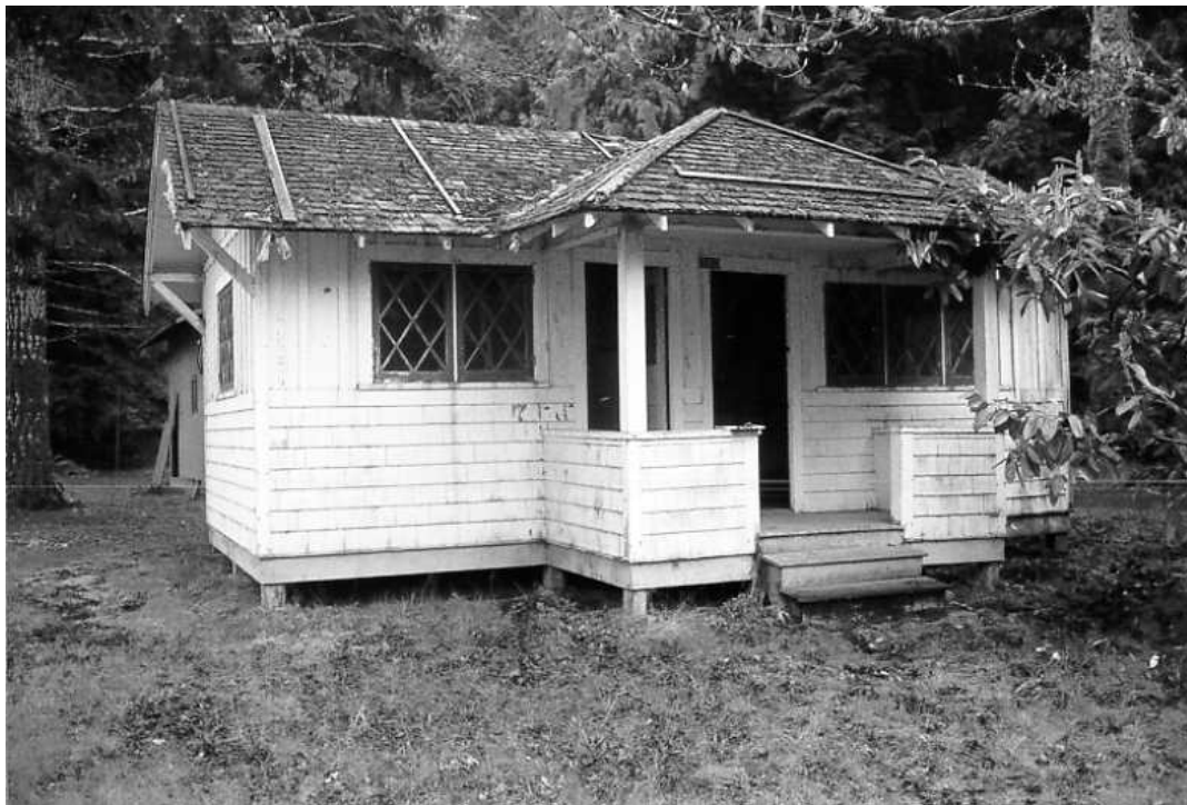
Contemporary photograph of Red Wing, one of the guest cabins at Rosemary Inn, built before 1926. This cabin has not been reconstructed and is in poor condition. (CCSO, 1999.)
