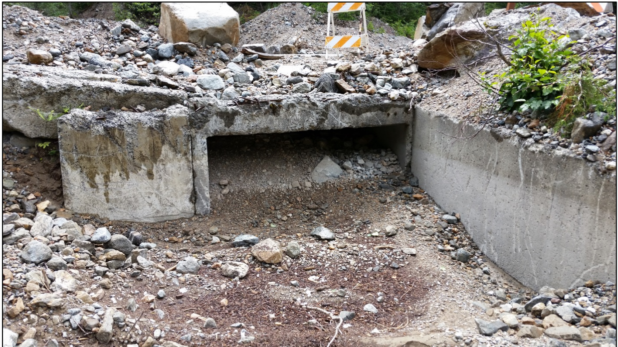
Figure 9. Debris flow from Rhode Creek clogging a culvert and spilling over the access road at Colonial Creek Campground, November, 2015.
