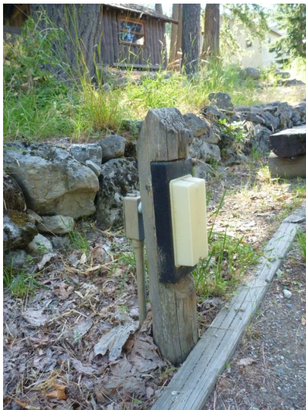
Small Scale Features #12: Lighting along main path, looking southeast. (PWR, June 2013)
