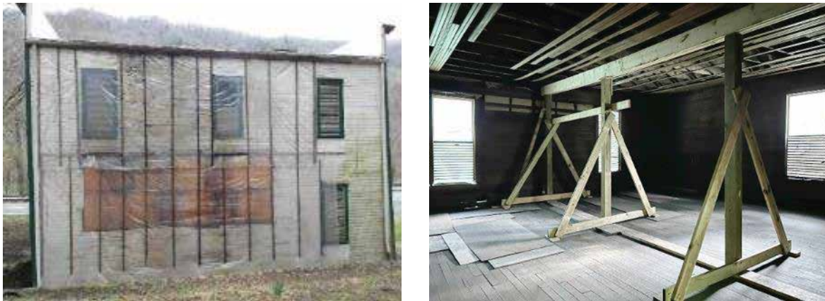
Figure 12. The Prince Brothers General Store has suffered extensive water damage, resulting in an unstable structure and collapsing rear wall (left) that continues to degrade over time. An interior beam truss system (right) was installed in 2021 as an extreme stabilization measure.
