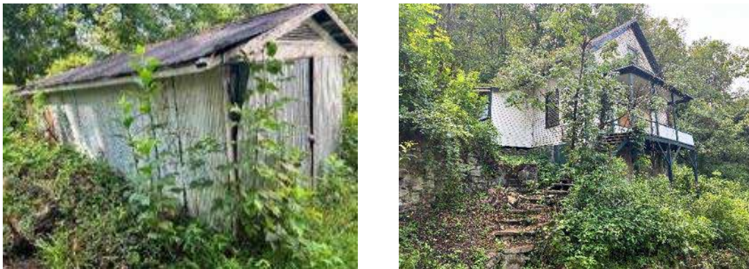
Figure 9. The McGuffin Garage (left) and the Wedzel Young House (right) are examples of overgrown, unsafe, deteriorated historic structures within the Thurmond Historic District that are proposed for demolition.
