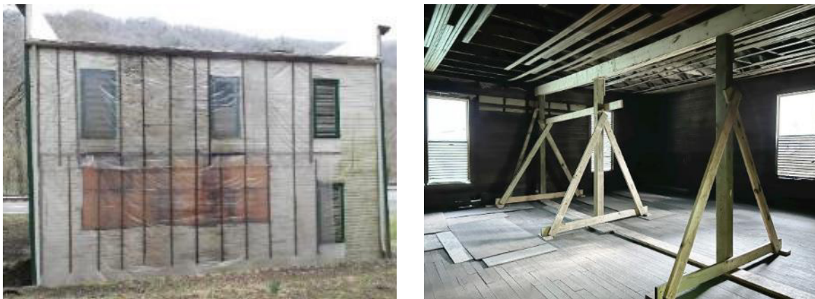
Figure 11. The Prince Brothers General Store has suffered extensive water damage, resulting in an unstable structure and collapsing rear wall (left) that continues to degrade over time. An interior beam truss system (right) was installed in 2021 as an extreme stabilization measure.
