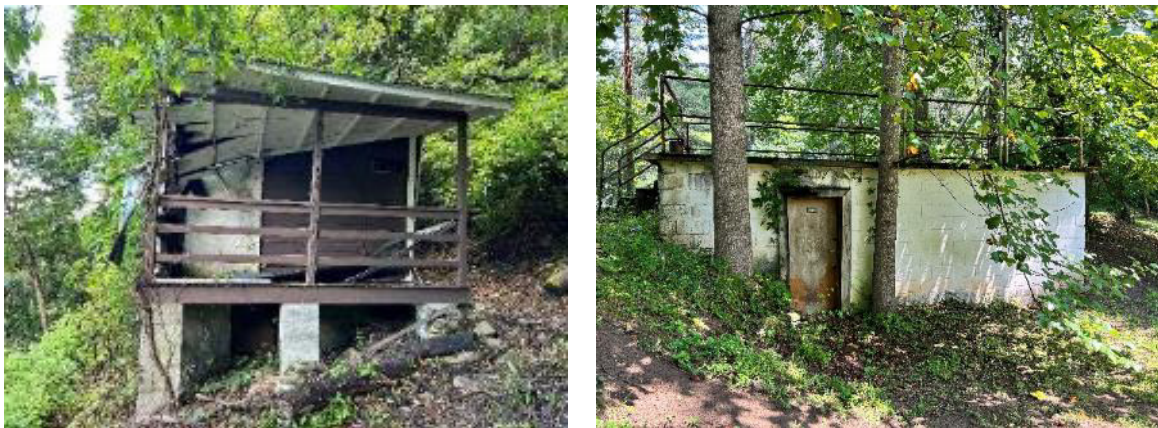
Figure 8. The Erskine Pugh Rental House (left) and the Camp Brookside Pool Chemical Treatment Building (right) are examples of the overgrown, deteriorated, unused structures within the park.
