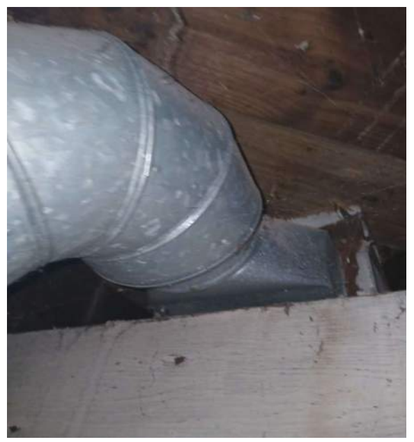
Photograph 18: Asbestos insulation on ductwork in basement (Note: Present behind walls on first and second floors, and wall and grates).
