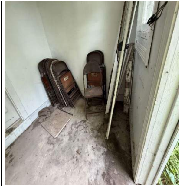
Photograph 35: Exterior rear porch LBP door frame.
