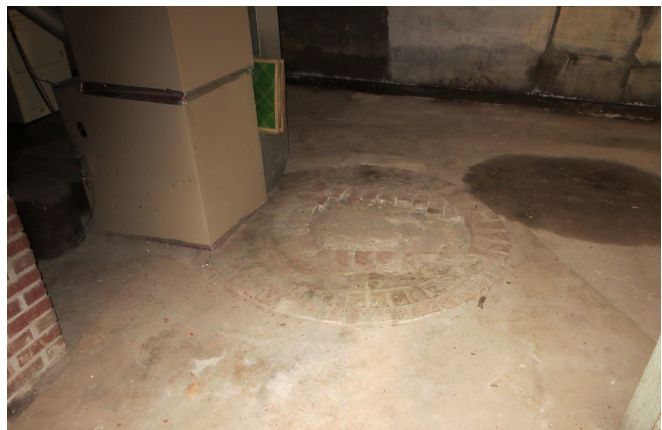
Figure 57. Basement, Looking East at Brick Cistern at Floor Behind Furnace. (source: Alvine, 2025)
