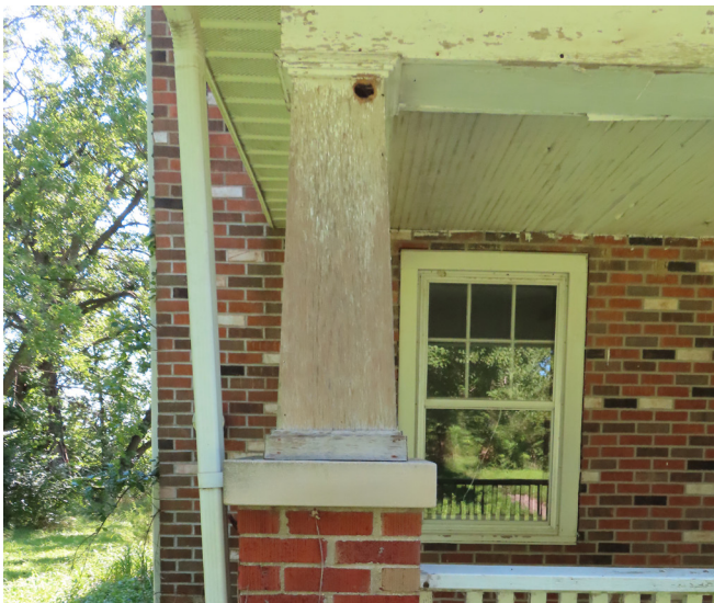
Figure 30. Northwest porch column with weathered paint and large pest hole at top.
