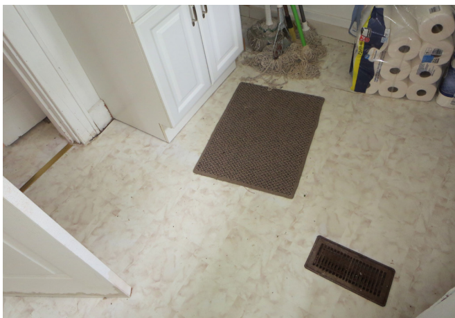
Figure 105. First Level, Looking South at Floor Supply Air Register at Restroom. (source: Alvine, 2025)
