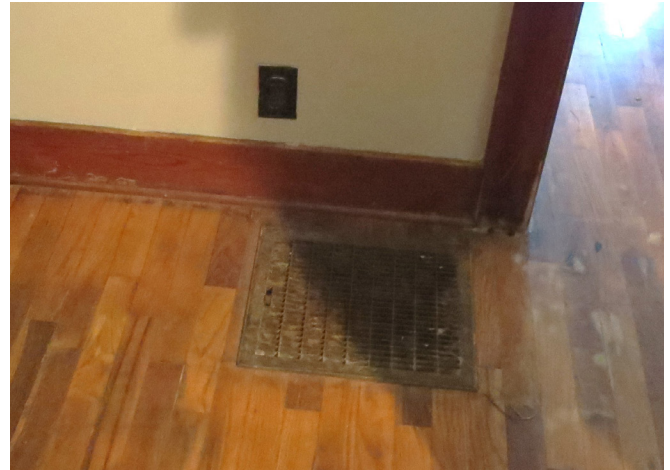
Figure 101. First Level, Looking North at Floor Located Supply Air Register. (source: Alvine, 2025)
