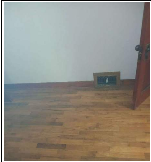
Photograph 25: Typical view of wall grates on first and second floor (Note; Asbestos insulation wrapped around ductwork behind wall to second floor).
