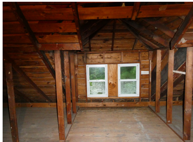
Figure 51. Roof framing at west dormer with inappropriate load path. (source: RRJ, 2025)
