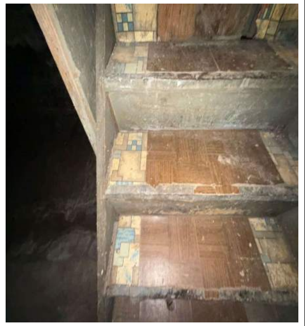
Photograph 34: Basement stairway asbestos beige floor tile assumed beneath brown and yellow green floor sheeting.
