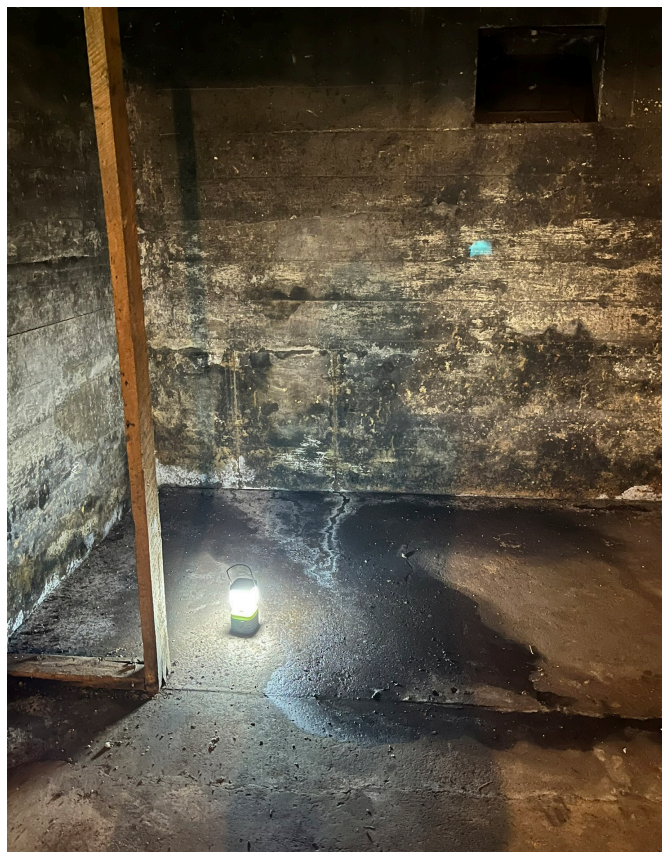
Figure 49. Interior concrete foundation wall with active water leak. (source: RRJ, 2025)
