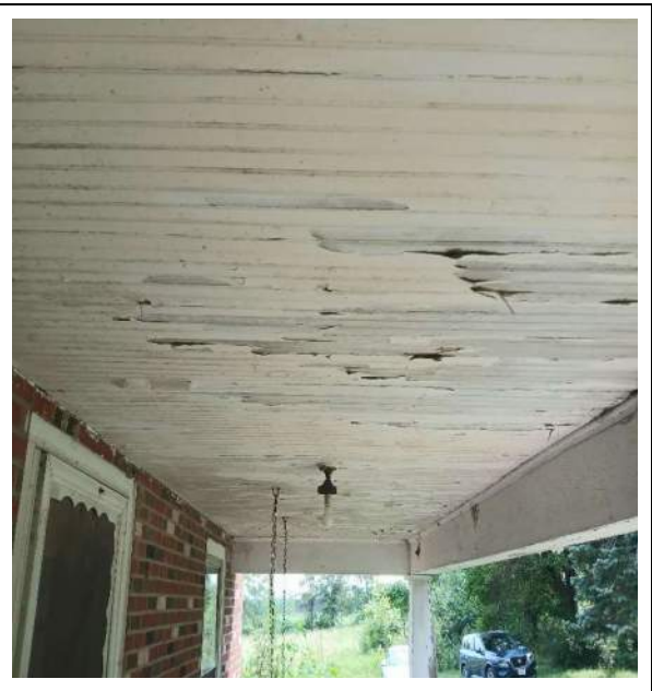
Photograph 4: LBP front porch ceiling and beams. LBP front door frame and windows, window frames and sill.
