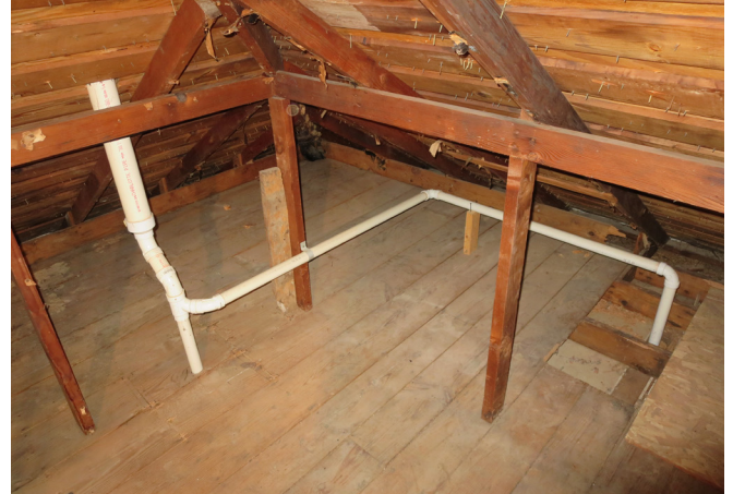
Figure 68. Attic Level, Looking Northwest at PVC Vent Piping Serving Second Level Restroom. (source: Alvine, 2025)
