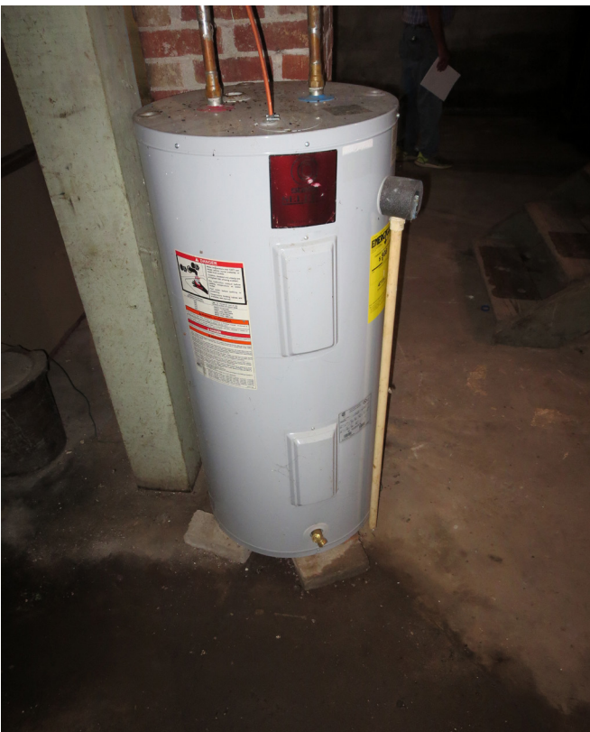
Figure 69. Basement Level, Looking South at Water Heater Adjacent to Brick Chimney and Furnace. (source: Alvine, 2025)
