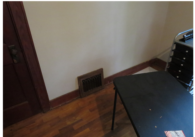
Figure 102. First Level, Looking West at Wall Located Return Air Inlet Grille. (source: Alvine, 2025)
