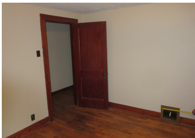
Figure 109. Second Level, Looking East at Wall Located Supply Air Register at Southwest Corner Room. (source: Alvine, 2025)
