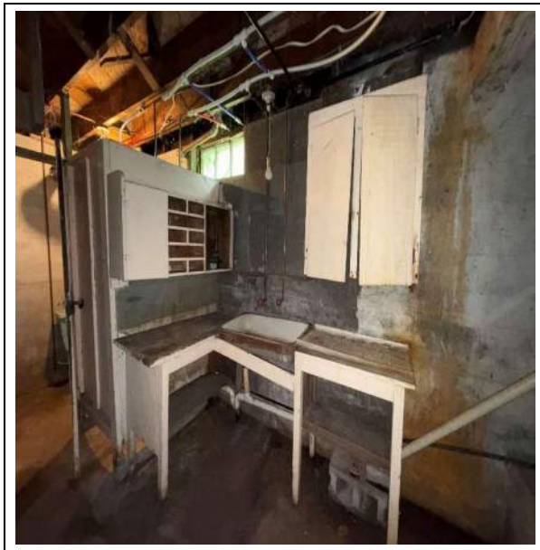
Photograph 23: Basement LBP cabinetry, cabinetry doors, shelving, tool bench and tool bench shelving.
