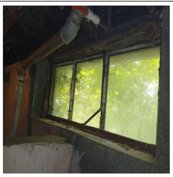
Photograph 20: Asbestos window glazing in two basement windows (south side).
