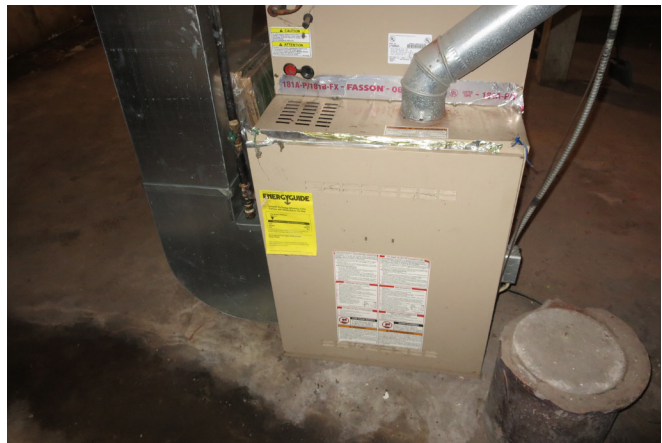
Figure 90. Basement Level, Looking South at Existing Propane-Fired Furnace. (source: Alvine, 2025)
