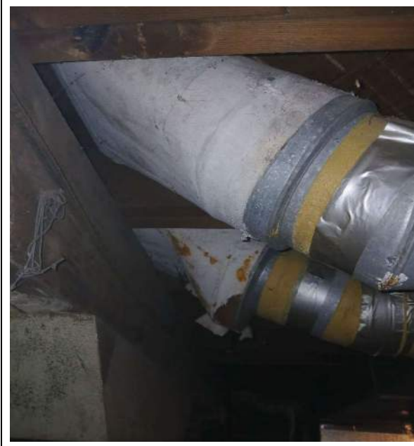
Photograph 17: Asbestos insulation on ductwork in basement (Note: Present behind walls on first and second floors, and wall and grates).
