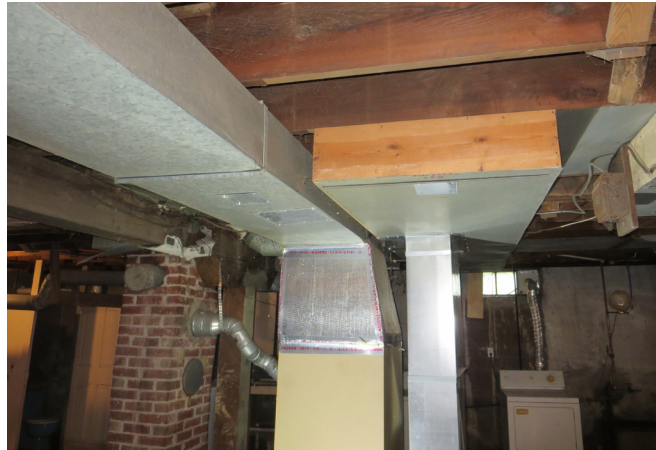
Figure 95. Basement Level, Looking North at Furnace Supply and Return Air Ductwork. (source: Alvine, 2025)
