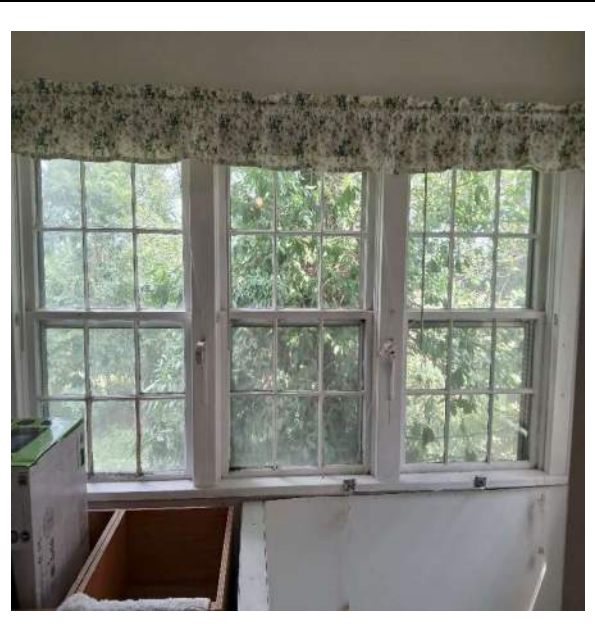
Photograph 26: East interior LBP window mullion, window frame and sill in first floor bath.
