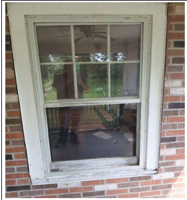
Photograph 5: LBP front porch window frame, window and sill.
