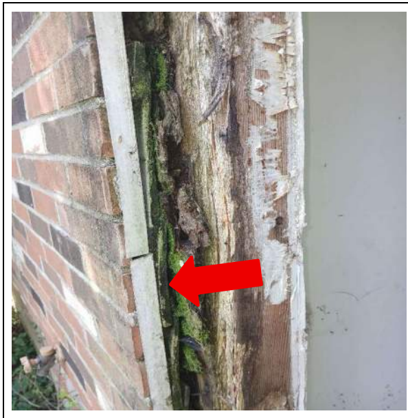
Photograph 11: North exterior wall (Note: LBP gray wood siding beneath fake brick veneer).
