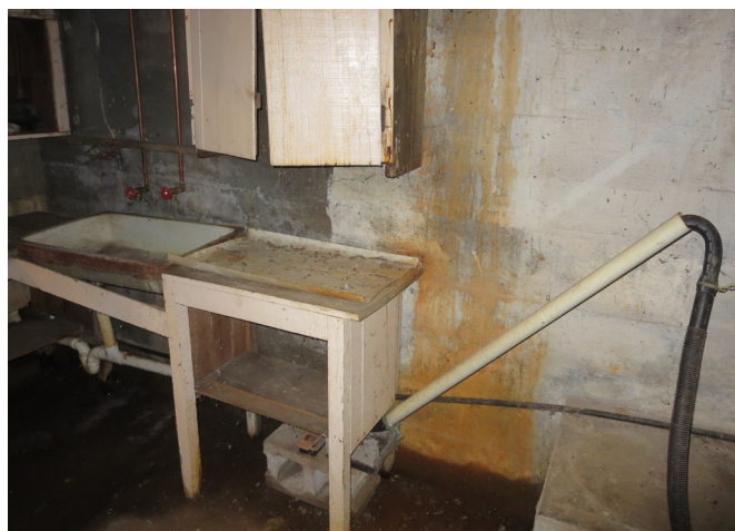
Figure 77. Basement Level, Looking at Sanitary Piping Washing Machine Standpipe at North Wall. (source: Alvine, 2025)
