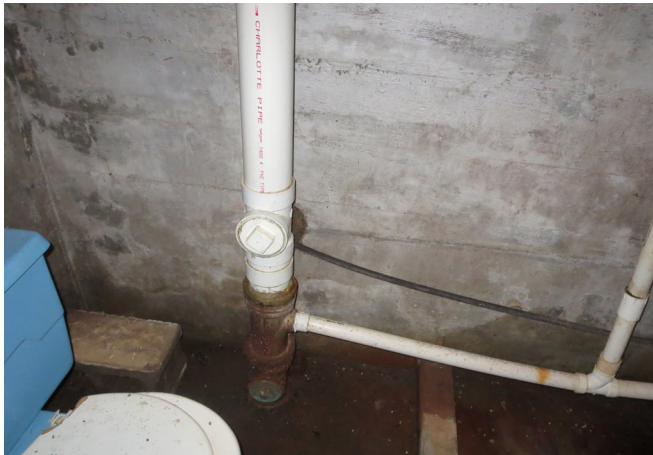
Figure 64. Basement Level, Looking North at Sanitary Piping Along North Wall. (source: Alvine, 2025)
