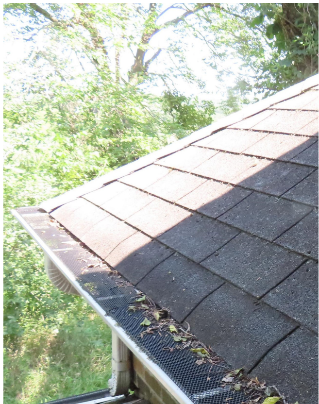
Figure 26. Roof level gutter with screen guard in place. (source: RRJ, 2025)
