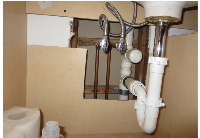
Figure 67. Second Level, Looking East at Piping Under Counter Lavatory. (source: Alvine, 2025)
