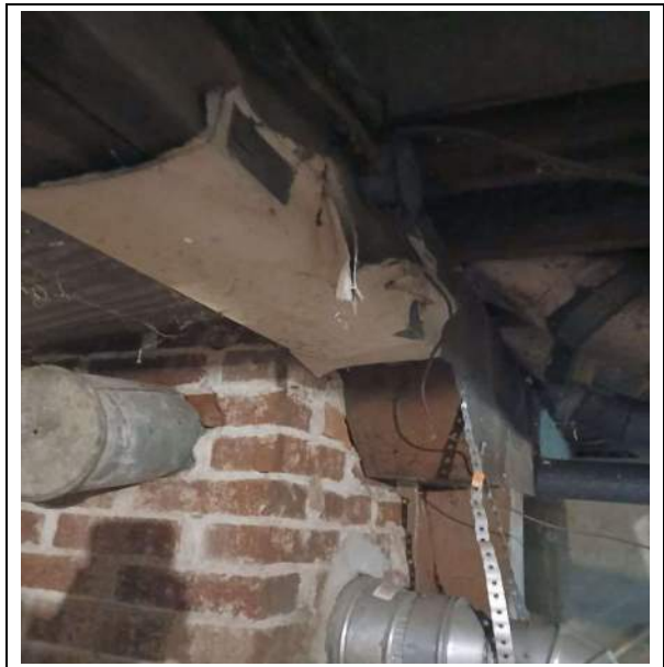
Photograph 16: Asbestos ductwork insulation location in basement.
