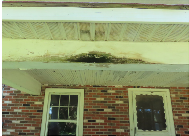
Figure 31. Large area of wood rot of the wood trim around the main porch beam. (source: RRJ, 2025)
