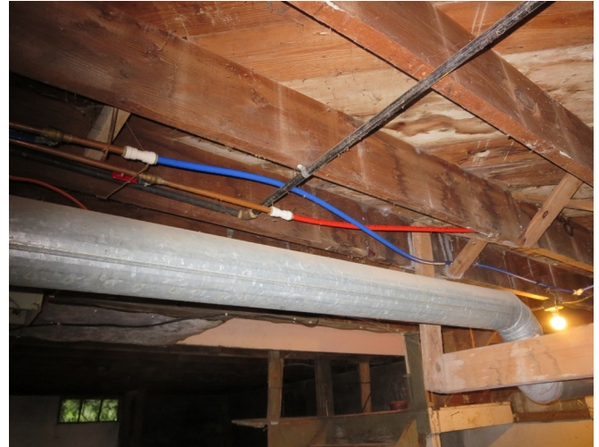
Figure 59. Basement, Looking Northeast Towards Stairs at Copper and PEX Water Piping. (source: Alvine, 2025)
