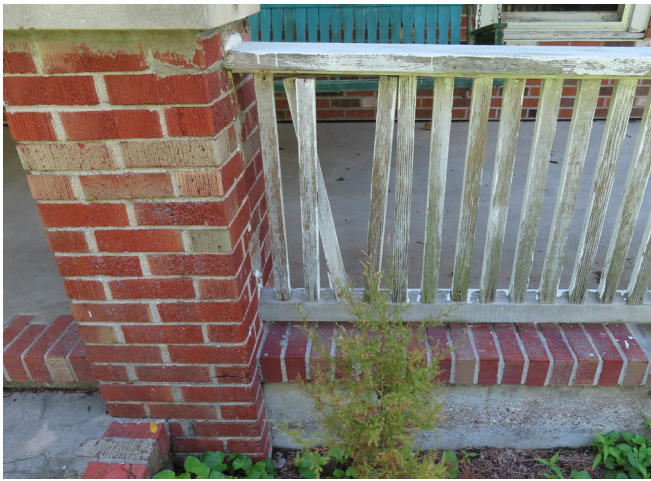
Figure 29. Porch railing with weathered paint and broken rails.. (source: RRJ, 2025)
