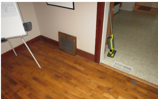
Figure 104. First Level, Looking West at Wall Supply Air Register and Floor Located Supply Air Register at Kitchen. (source: Alvine, 2025)
