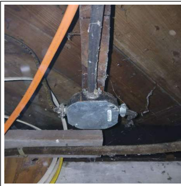
Photograph 19: Assumed asbestos wire cover visible in basement (Note: Eiring goes up through floor joists as observed in basement).
