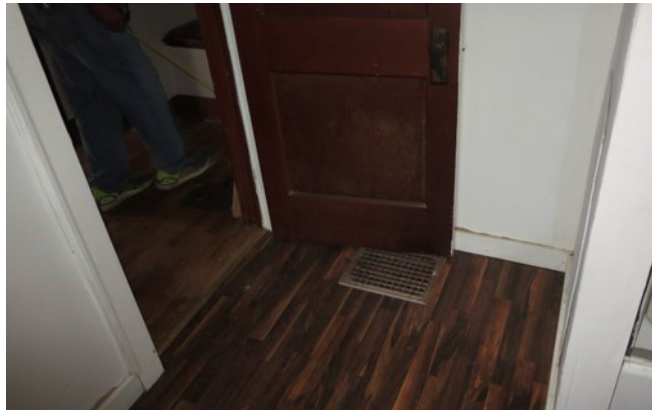
Figure 107. Second Level, Looking South at Floor Located Supply Air Register at Restroom. (source: Alvine, 2025)
