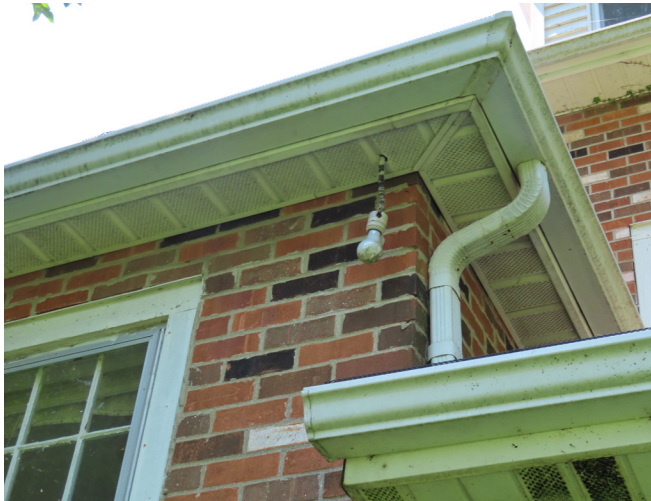
Figure 27. Downspout and gutter at rear porch. (source: RRJ, 2025)
