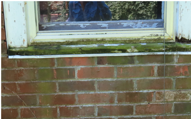
Figure 37. Deterioration of exterior wood sill, typical. (source: RRJ, 2025)
