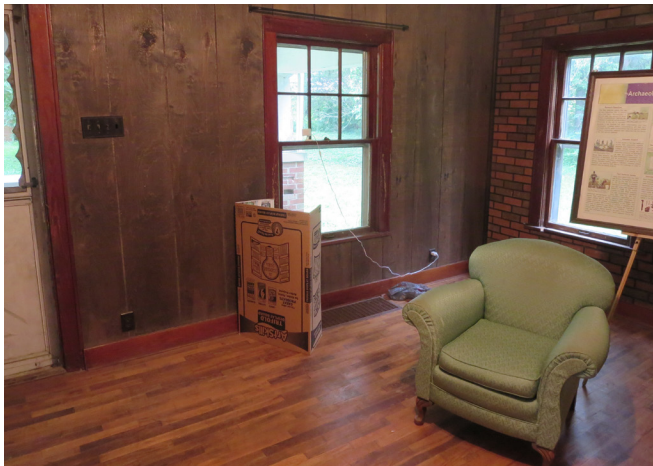
Figure 99. First Level, Looking Southeast at the Floor Supply Air Register Below the Window at the East Wall. (source: Alvine, 2025)
