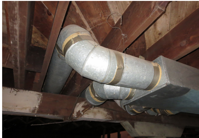
Figure 96. Basement Level, Looking Northeast at End of Supply Air Duct Main and Round Branch Ducts. (source: Alvine, 2025)
