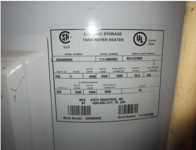
Figure 70. Basement Level, Looking at Water Heater Label. (source: Alvine, 2025)
