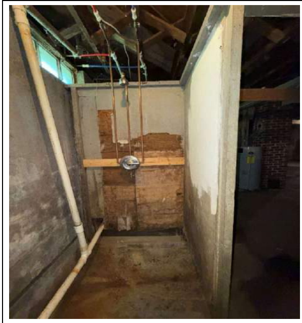
Photograph 21: Basement LBP shower walls.
