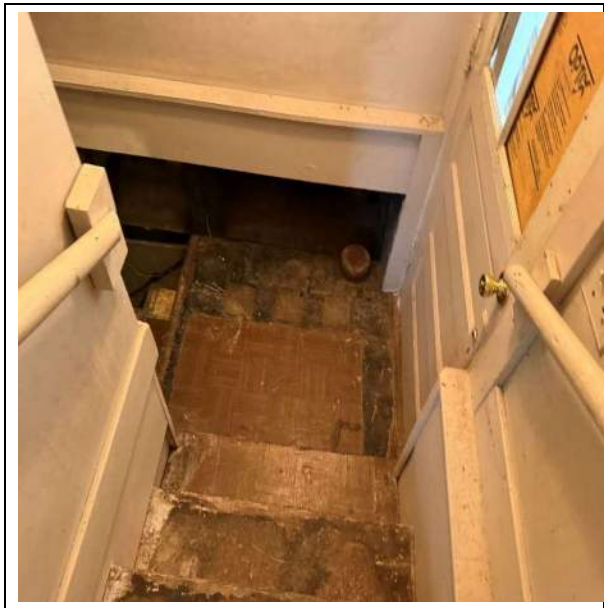
Photograph 32: Basement landing LBP door, door frame, baseboard, header board (Note: Asbestos floor tile beneath brown, black and brown floor tile, floor felt and yellow green floor sheeting).
