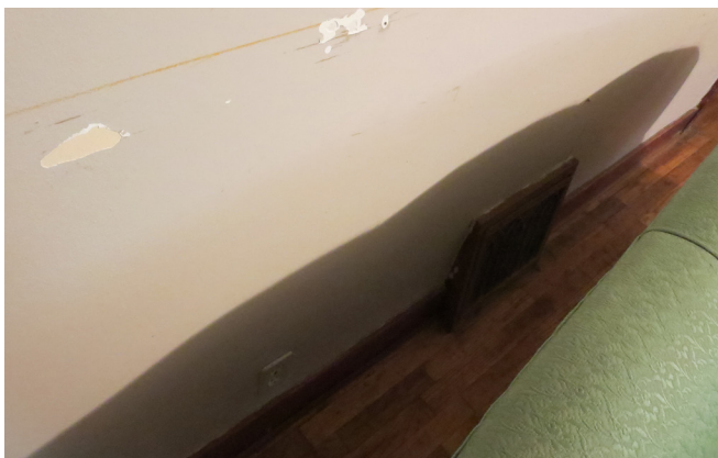
Figure 100. First Level, Looking West at Wall Located Return Air Duct Inlet Grille. (source: Alvine, 2025)
