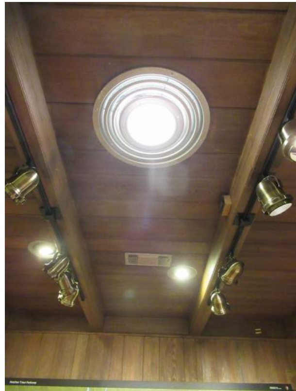
Figure 106. Detail of existing lighting in Exhibition Room.
