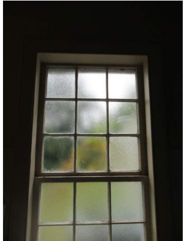
Figure 101. Mismatched obscure glazing from Accessible Family Restroom. The glazing should be replaced to maintain a consistent appearance of the original glazing.
