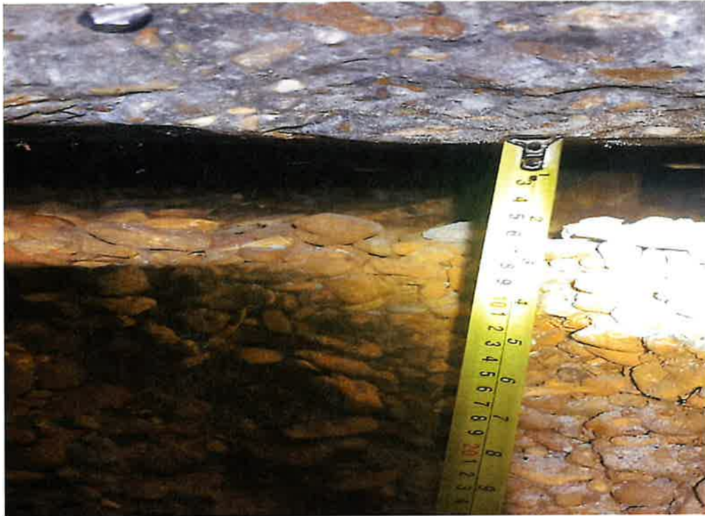
Photograph No. 9 - A void was observed below the concrete slab.
