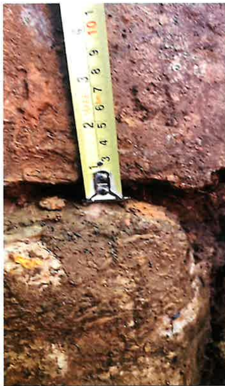
Photograph No. 4 – Top of pile was not in contact with grade beam near edge of exposed grade beam.
