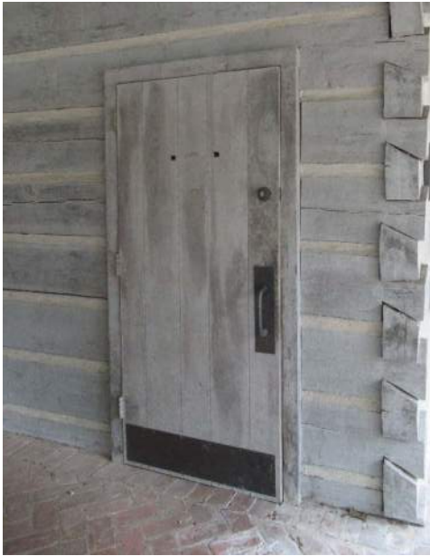
Figure 100. Consider replacement of veneered hollow core doors with solid wood batten doors with iron strap hinges and pulls.
