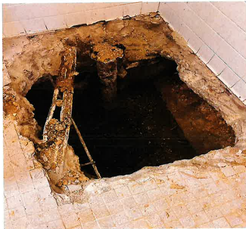
Photograph No. 8 – TP#2 inside of the women's bathroom. A significant number of rootlets were observed in TP#2.
