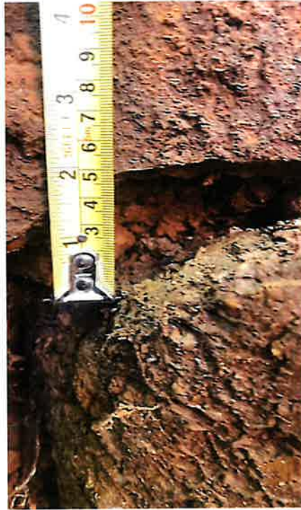
Photograph No. 5 – Top of pile was not in contact with grade beam near edge of exposed grade beam.
