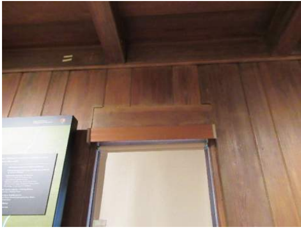
Figure 107. Valance for window treatment should be eliminated.
