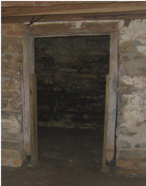
Figure 82. Interior basement door showing sistered pieces, 2010.
