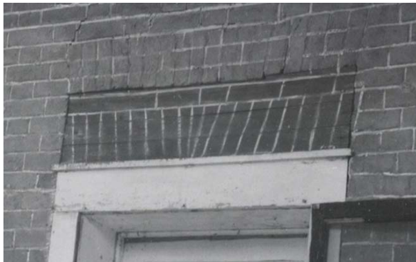
Figure 52. Wood-boxed opening masking the transom and painted to simulate brick jack arch, with disguised jack arch above. ("Frost," [Trout?] 1969, NATR collection #10907)
