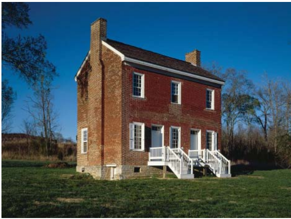
Figure 80. South elevation showing poor repointing, ghostmarks of earlier porches and second-floor center doorway, and stairs constructed in 1995. (color transparency, 1998, HAER Survey #MS-15)
