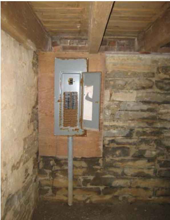
Figure 103. Electrical panel box of 1977-78 on north wall of Room 002.
