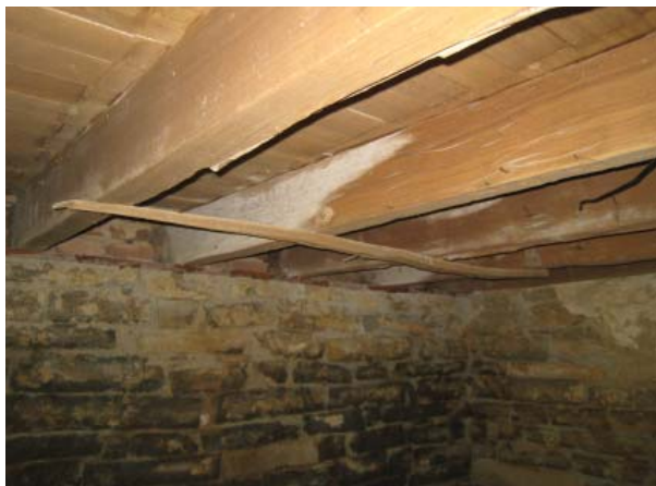
Figure 124. Split wood hanger in Room 001.
