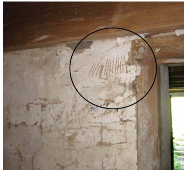
Figure 129. Graffiti scratched into limewash of west wall of Room 002.
