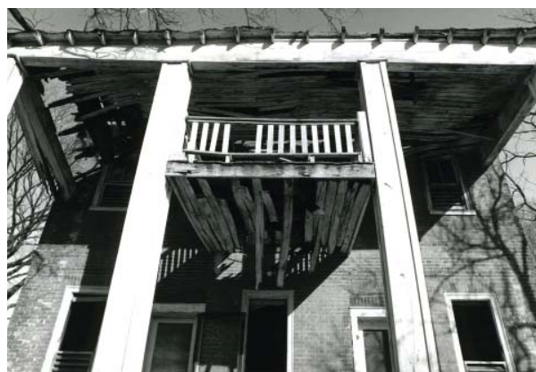
Figure 63. 1977 NPS photograph showing deteriorated condition of the porch. (NATR collection)
