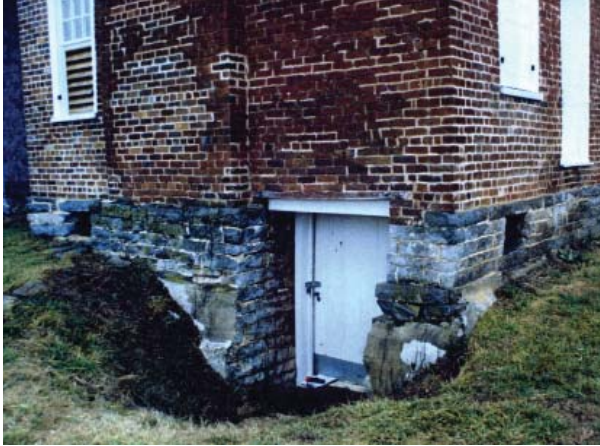
Figure 74. 1991 view showing inappropriate repointing and steep grade near basement entrance. (HSAR 1992)
