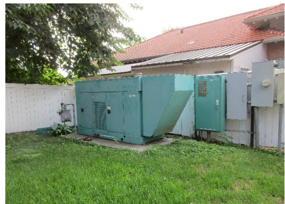
FIGURE 3-13. Photograph taken in 2019 of the site's electric generator and electrical panels. Suzanne Turner Landscape Architecture.
