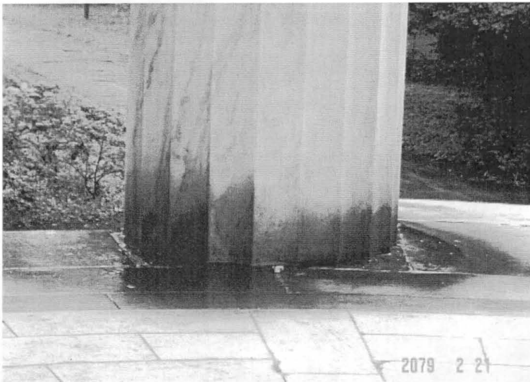
Dark-colored soiling at base of column. [MSSC, 2005]
