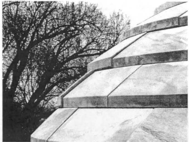
Photo 2. Displaced marble roof pieces.
