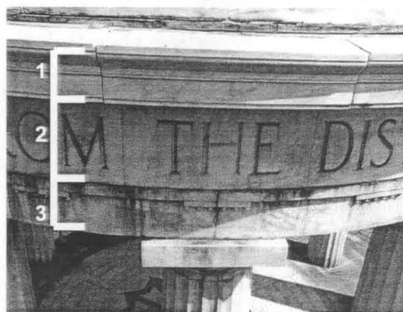
Photo 8. Displaced cornice element.
