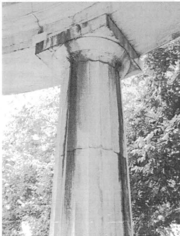
Vertical staining on interior of column. [MSSC, 2005]
