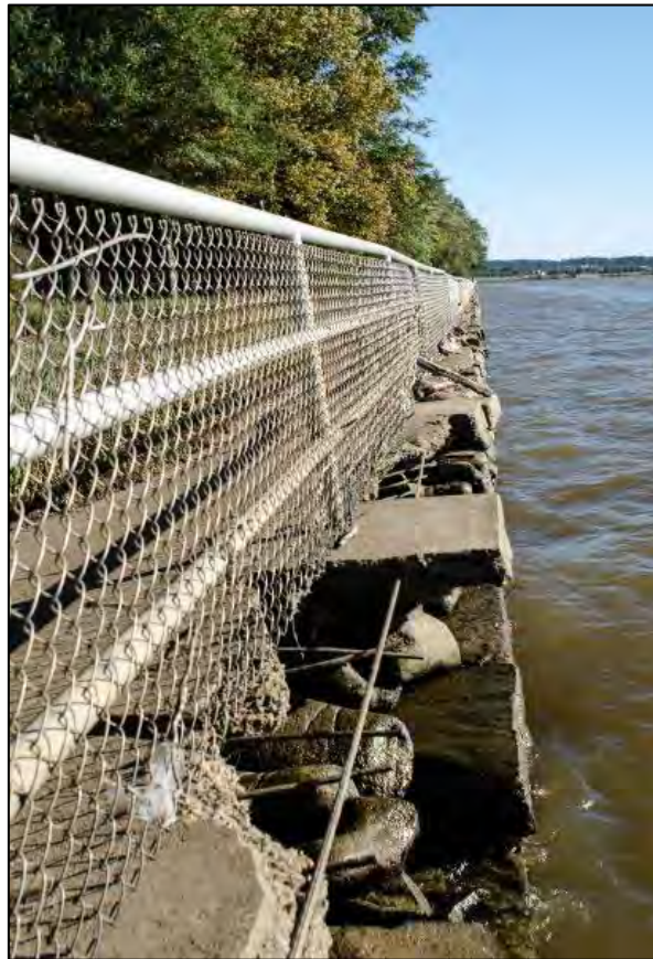
Fig 63. Photo looking southerly depicting damage to seawall on the Potomac River side of island (Matthew Traucht 2021).
