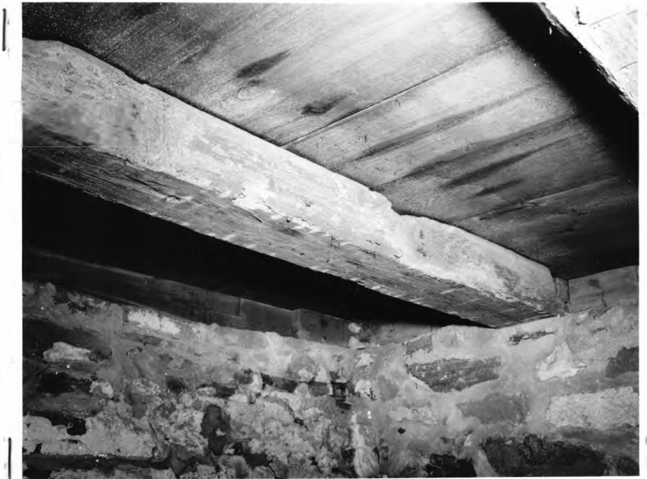
4. Condition of floor joists in cellar.
