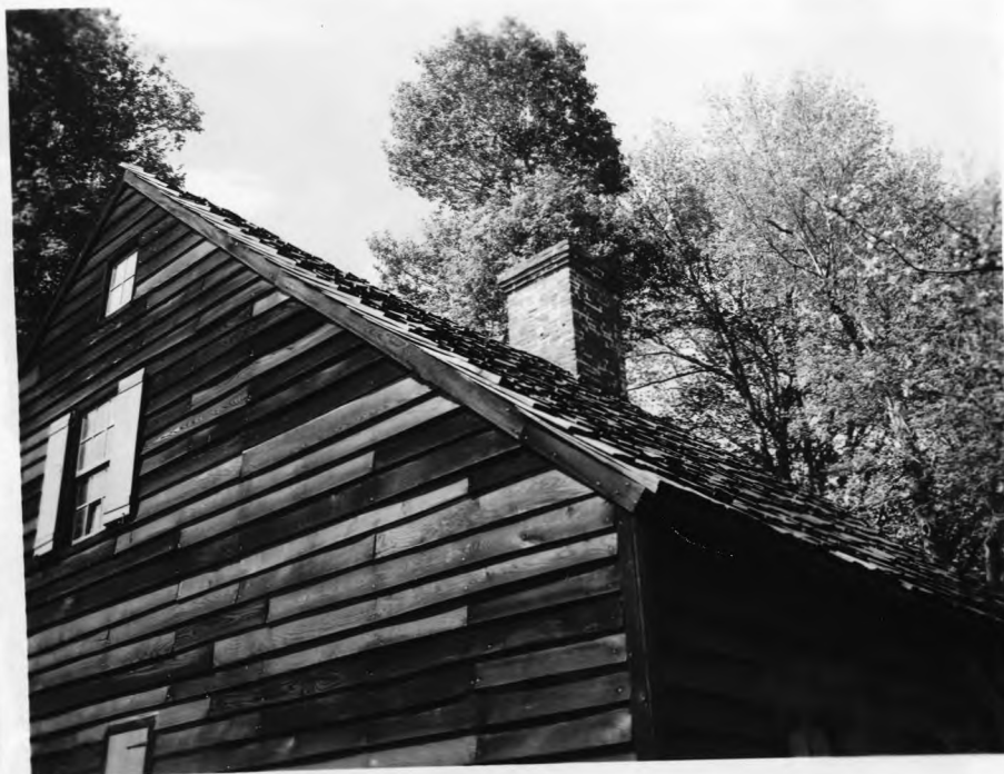
2. North and east sides of the chimney, showing the poor condition of the brick work.
