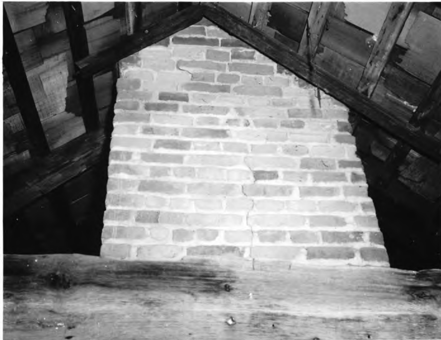
2. Chimney in attic, showing crack in brickwork.
