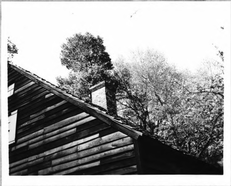
10. The warped siding of the east wall of the Wick House.
