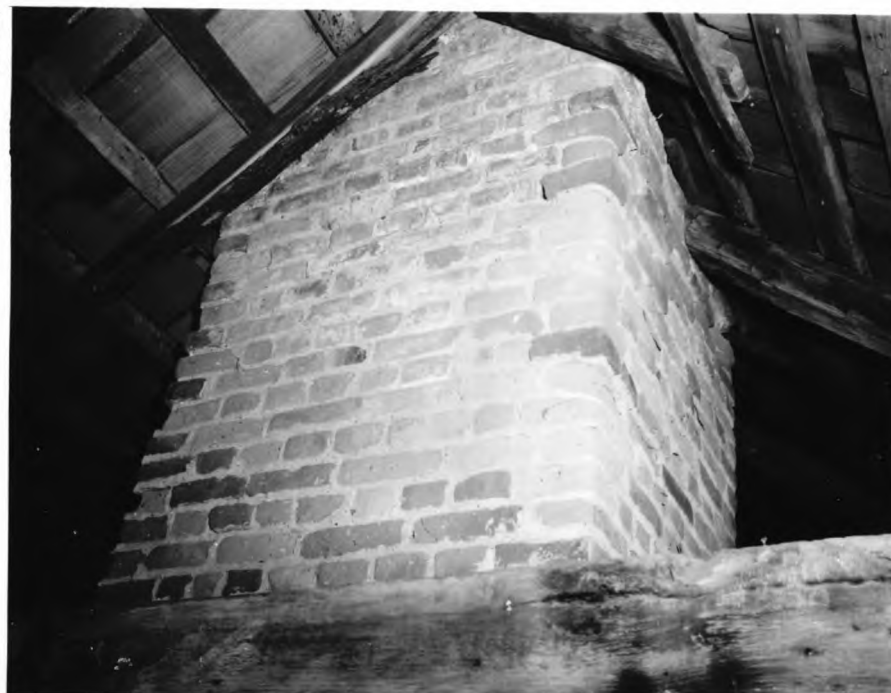
3. Chimney in attic, showing missing brick.
