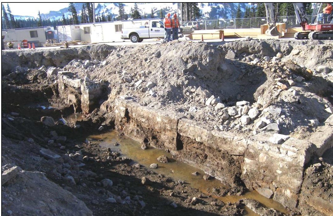
Figure 32. Paradise Camp Lodge, Exposed Eastern Foundation Wall
