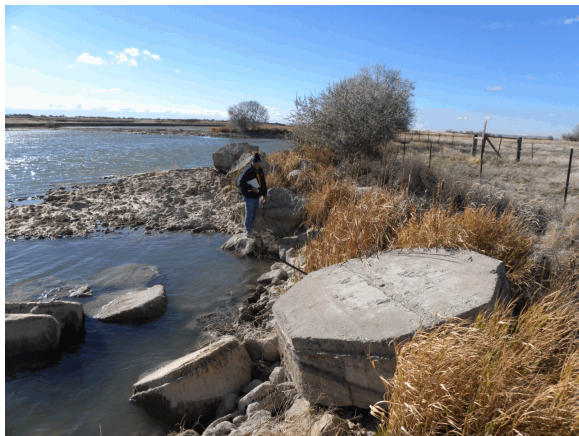
Figure 18. Large concrete debris, Robeson Property Feature 15.
