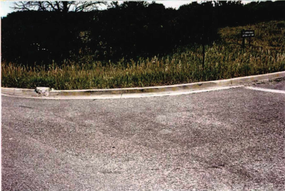
Photograph #12 - shows the curb for the exit from this driveway. It appears that right turning traffic out has broken the curb as evidenced by the black marks in the broken curb. Again, widening this throat and improving the radius would be desirable if this is the only entrance and exit.
