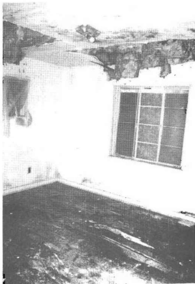
Figure 27. 1994 photograph of Bedroom 2 showing damaged floor and ceiling areas.
