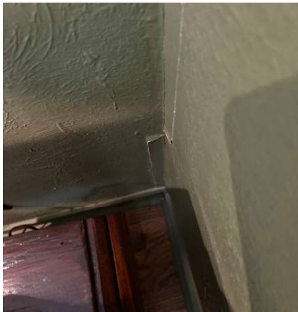
Figure 43. Torn and detaching corner bead in room 106.
