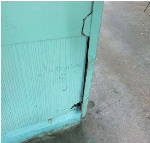
Figure 40. Broken panels and bent corner trim.
