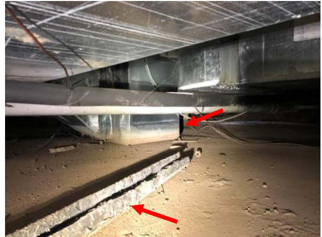
Photo 10 – Typical crawlspace. Dirt and debris. Water marks on ductwork.
