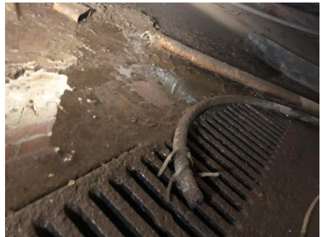
Photo 11 – Condensate lines draining in crawlspace.
