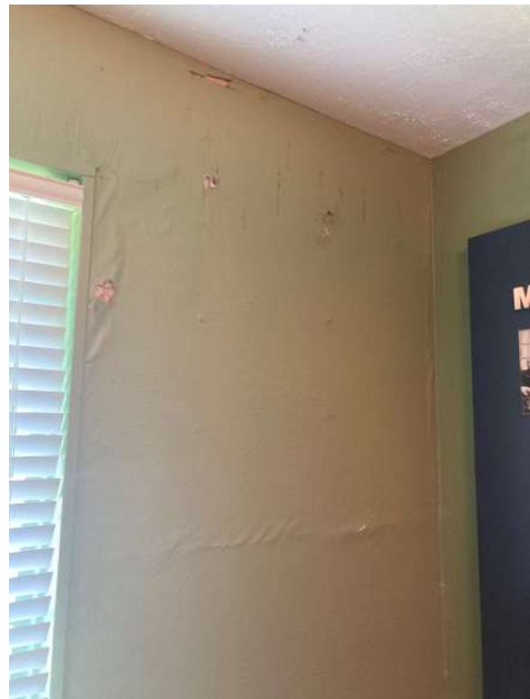
Figure 44. Visible moisture damage at exterior wall of room 107.
