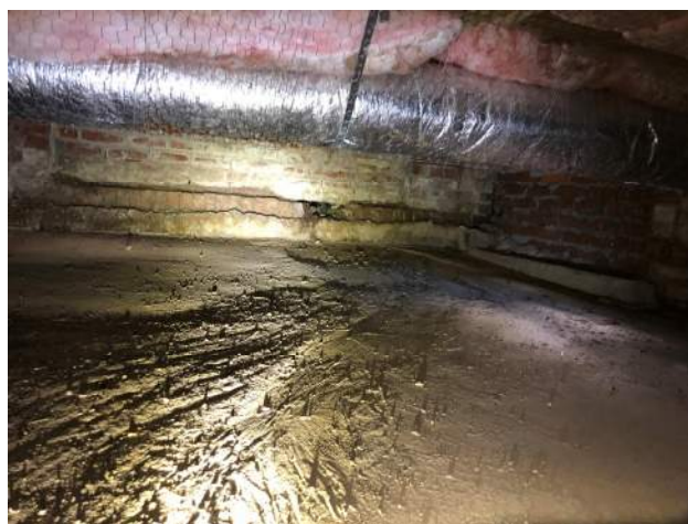
Photo 17 – Erosion of silt from moving water, leaking through west wall.
