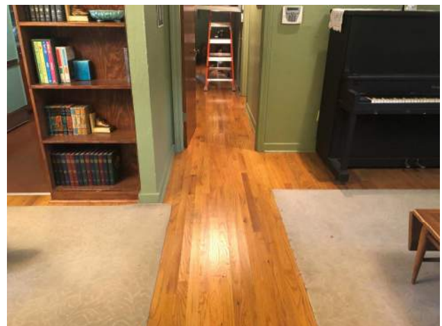
Photo 12 – Cupping of hardwood floors.
