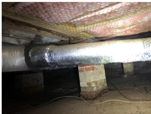
Photo 16 – Moisture at base of pier.
