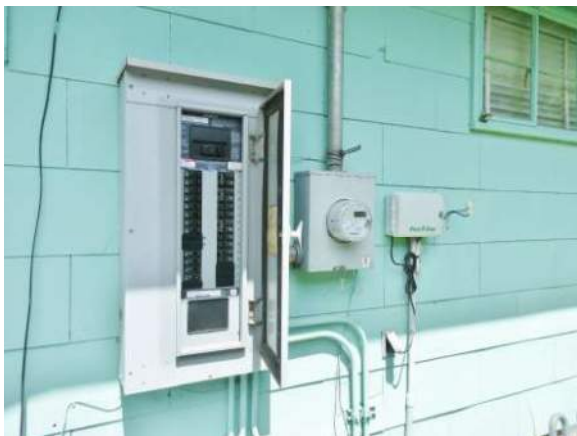
Figure 45. Active electrical panel.
