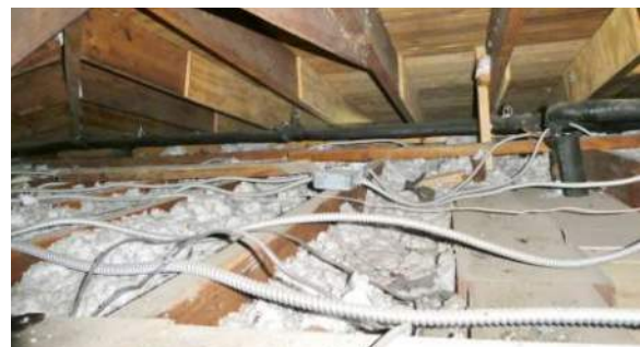
Figure 47. MC Cable and open junction box in attic.
