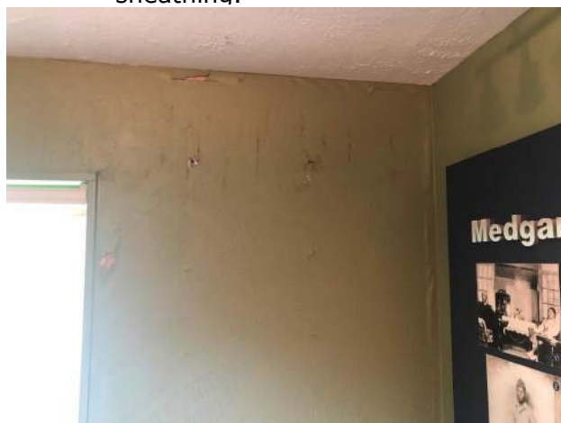
Photo 5 – Water damage of south wall of front bedroom.
