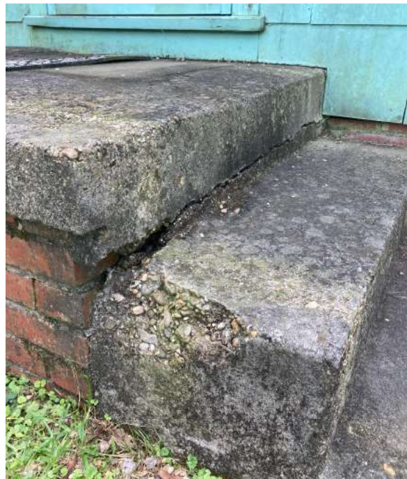
Figure 23. Spalling and crack at rear stair.
