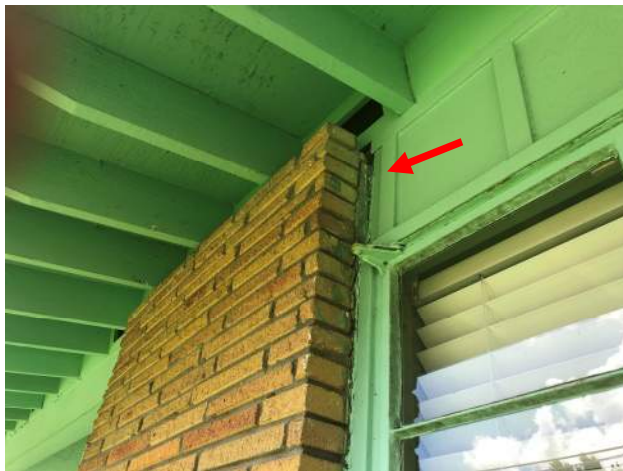
Photo 8 – Brick veneer at front of house. Slight gap.
