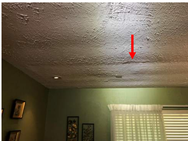
Photo 1 – Ridges in ceiling at attachment to furring strips.
