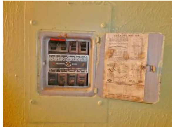
Figure 46. Original, inactive electrical panel.
