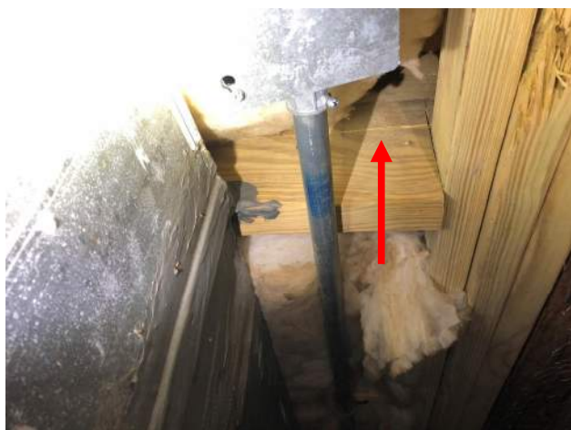
Photo 15 – Split in joist at notch at center beam.
