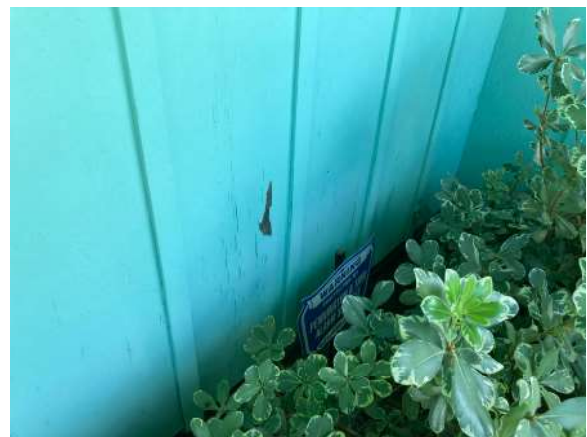
Figure 37. Paint peeling at planter.
