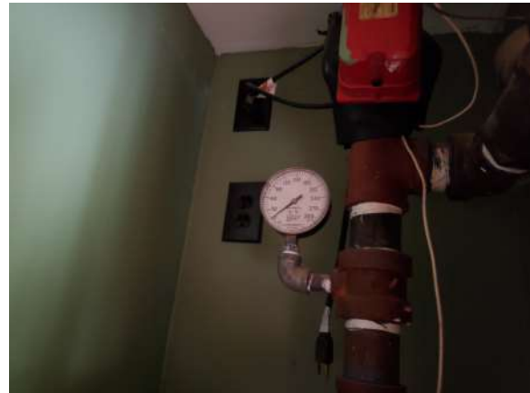
Figure 48. Pressure gauge indicating 0 psi.
