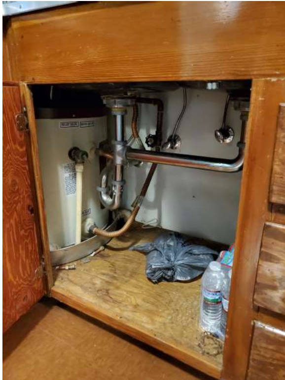
Figure 52. Water heater below kitchen sink.
