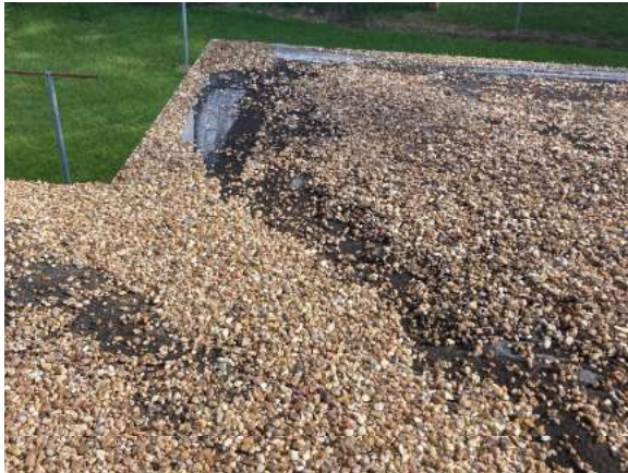
Figure 34. Shifted ballast in valley and edge of roof.
