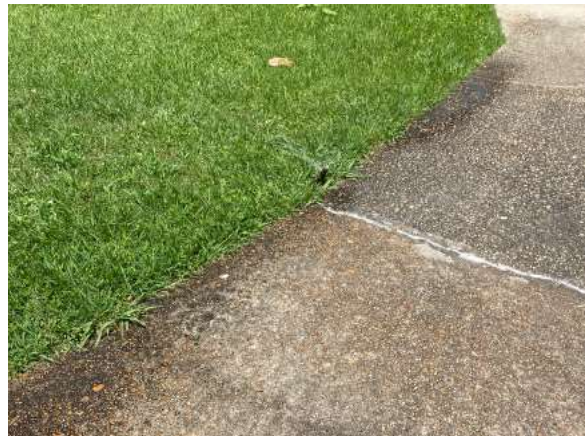
Figure 20. Damaged sprinkler head.
