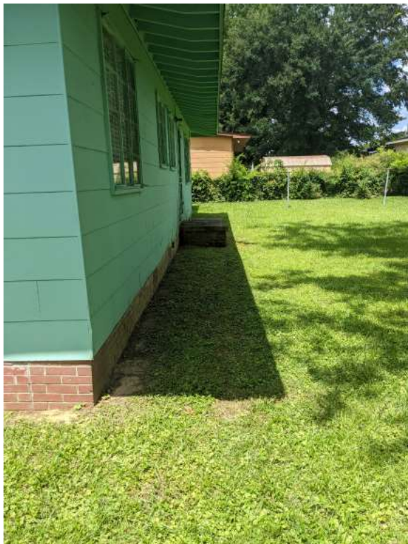
Figure 28. Drip edge erosion from roof.
