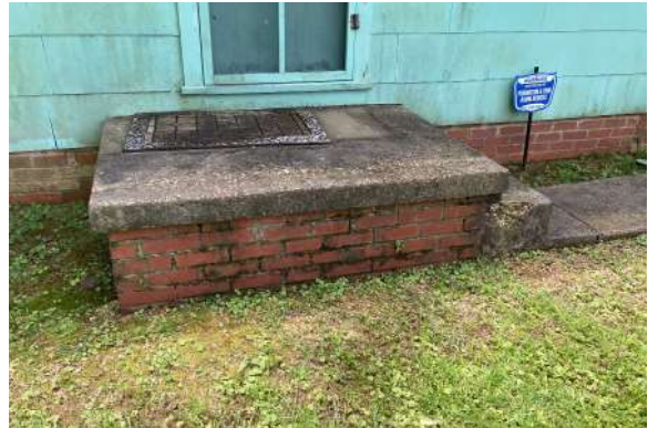
Figure 22. Existing rear stoop.
