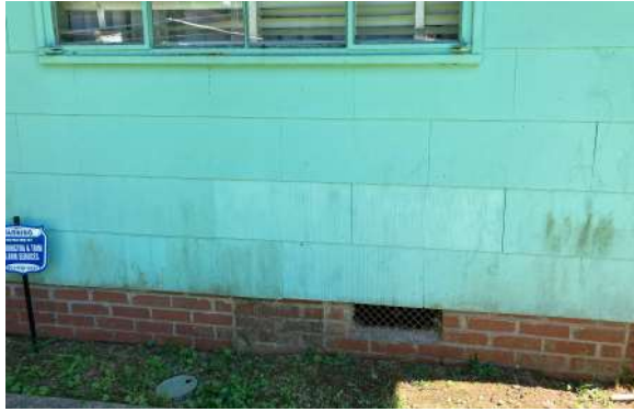
Figure 38. Dirt and discoloration on siding.
