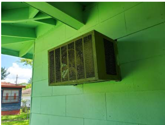
Figure 51. Historic Whirlpool wall unit, not in use.
