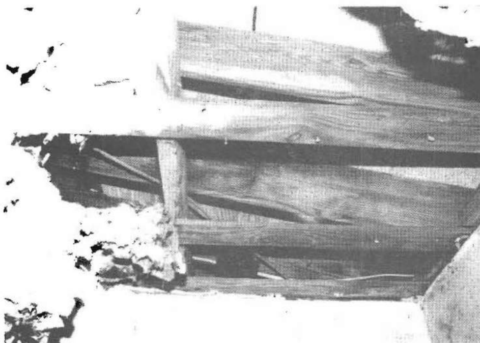
Figure 28. The fallen and deteriorated ceiling allows a view of the attic space above Bedroom 2 in this 1994 photograph. Areas of patched roof decking visible in the photograph have halted the leaks that caused the water damage.
