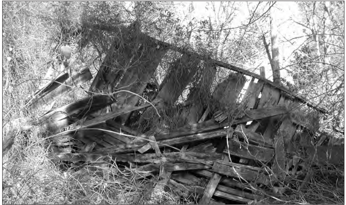
Figure 46. The ruined superstructure of the doublecrib barn is located a few hundred feet northeast of the farmhouse. (2002; NCR CLP digital photo)
