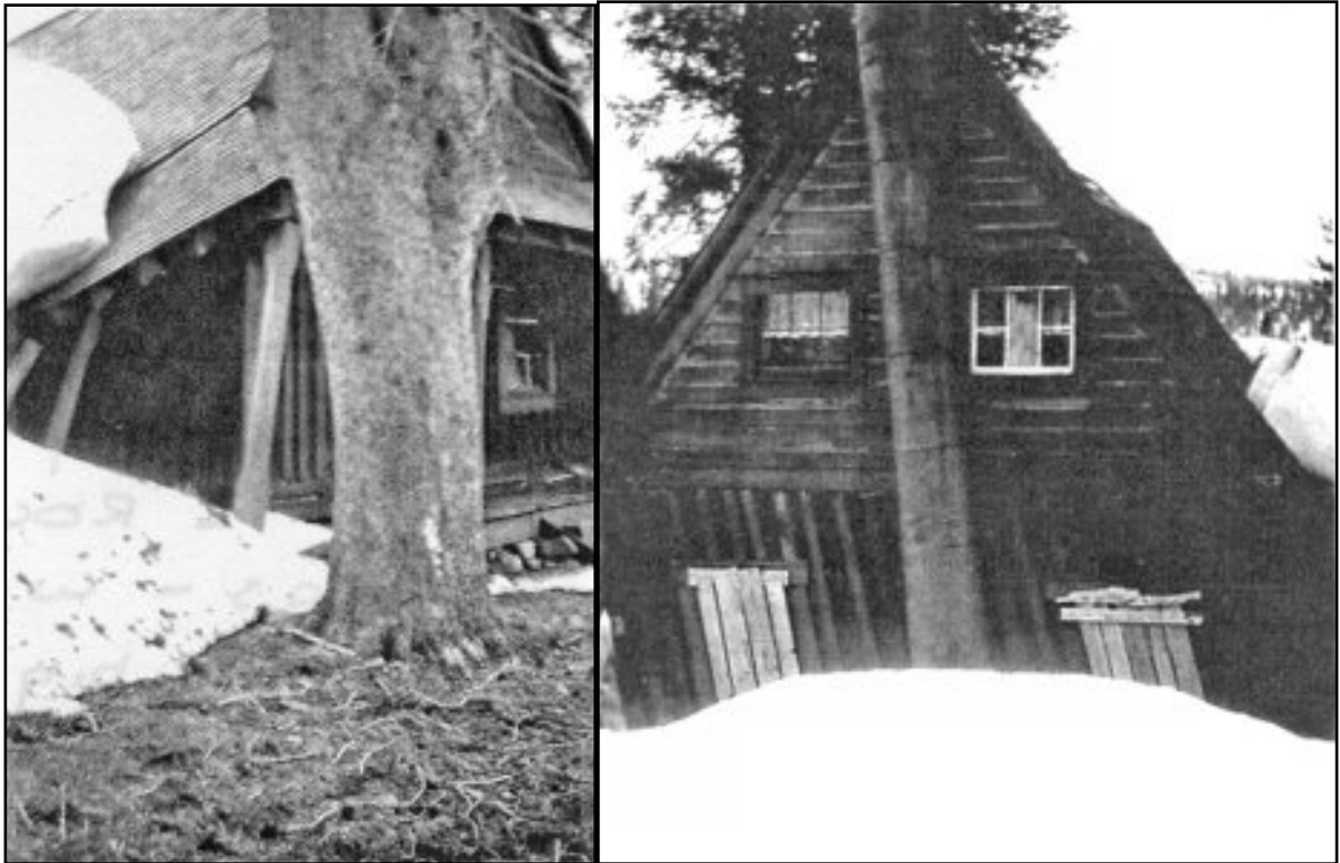
1938--Damage to the Lodge Left-- the Southwest Corner of the Lodge Right--the North Fireplace end
