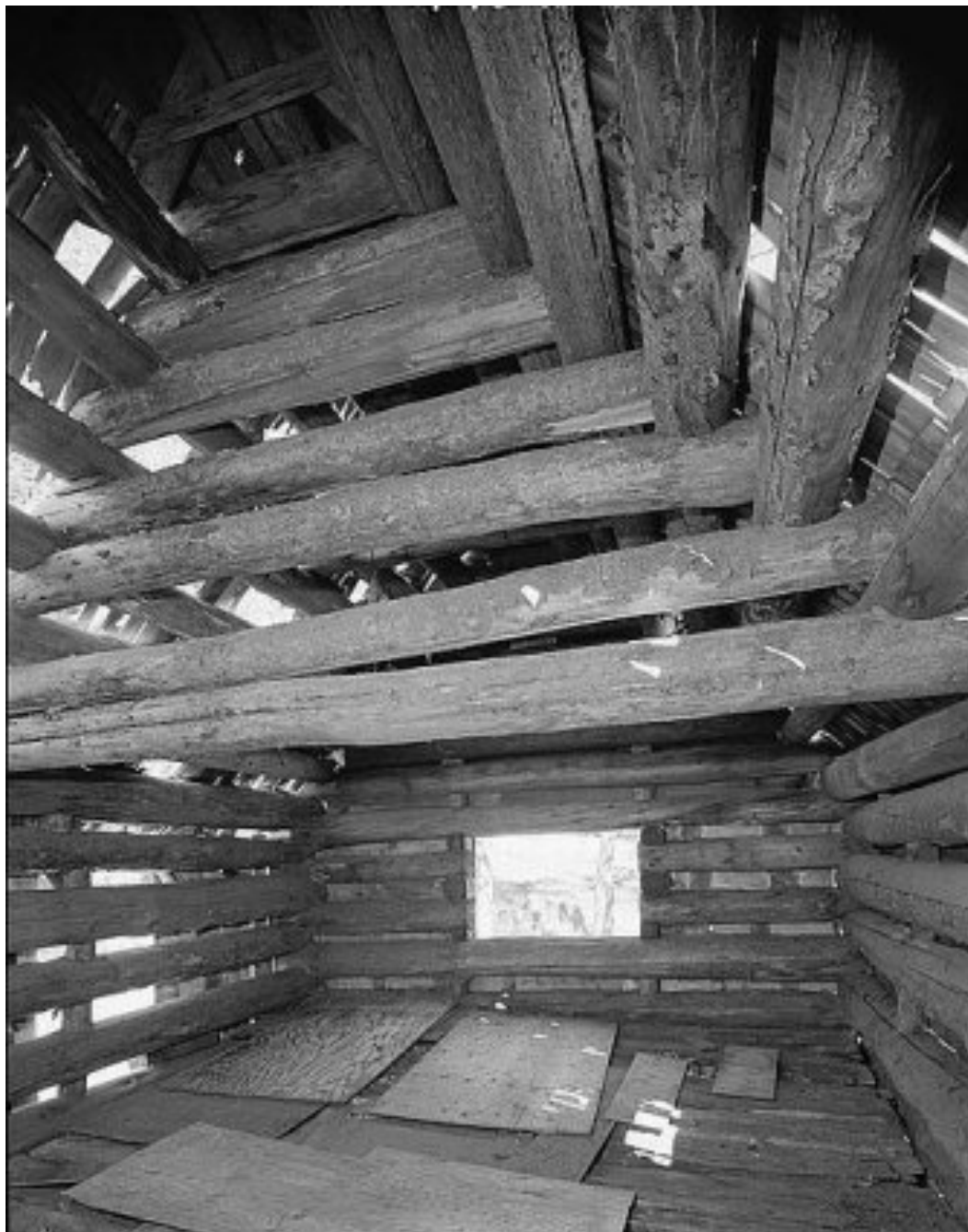
Circa 1976 Interior of log barn
