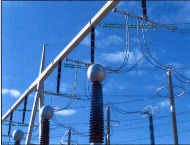
Grand Coulee Dam's 500kV Switchyard
