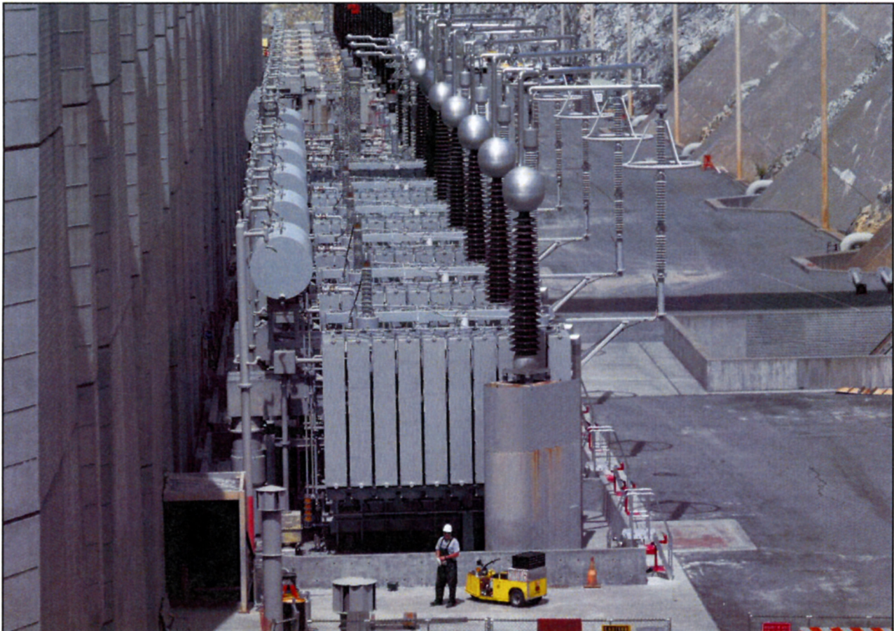
Third Power Plant Transformer Deck
