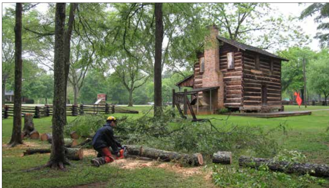
Removing a hazardous tree adjacent to the historic Logan Log House at Ninety Six National Historic Site. (OCLP)
