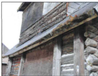
Figure 89. Biological growth, west elevation, photographed by Kathleen Wackrow, NPS, April 2016 (NPS, AKRO, Historic Architecture, Patterson Cabin Digital Files).
