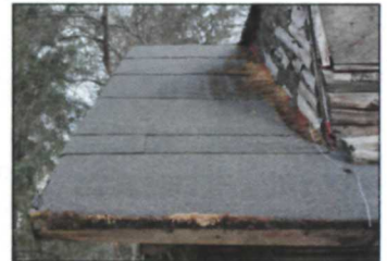
Figure 90. Biological growth, west elevation, photographed by Kathleen Wackrow, NPS, April 2016 (NPS, AKRO, Historic Architecture, Patterson Cabin Digital Files).
