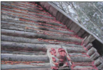
Figure 91. Dark stains, south elevation, photographed by Kathleen Wackrow, NPS, April 2016 (NPS, AKRO, Historic Architecture, Patterson Cabin Digital Files).
