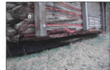
Figure 84. Wood rot on sill, west elevation, photographed by Kathleen Wackrow, NPS, April 2016 (NPS, AKRO, Historic Architecture, Patterson Cabin Digital Files).
