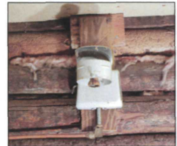
Figure 83. Propane lamp, second floor (attic), photographed by Kathleen Wackrow, NPS, April 2016 (NPS, AKRO, Historic Architecture, Patterson Cabin Digital Files).
