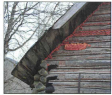
Figure 87. Broken vergeboard, north elevation, photographed by Kathleen Wackrow, NPS, April 2016 (NPS, AKRO, Historic Architecture, Patterson Cabin Digital Files).
