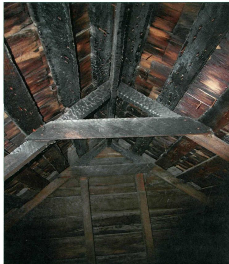
Figure 104: Charred ridge board, rafters and collar ties in attic section B. (NPS July 2008).
