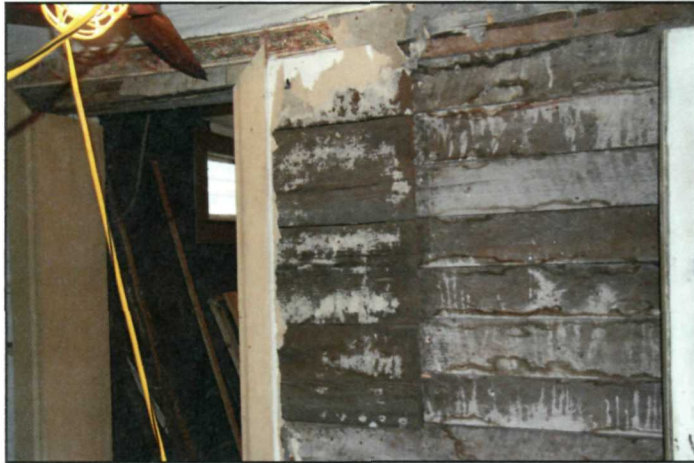
Figure 98: Wall in southwest corner of Room A-2, notice signs of water damage to boards (NPS July 2009).
