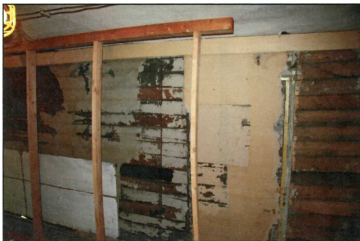
Figure 95: East interior wall room A-1 showing old door frame and remnants of felted cardboard that backed paper memorabilia that previously lined the wall (NPS July 2009).
