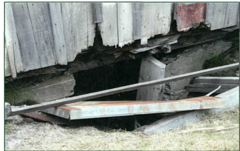
Figure 85: Deteriorating boards at crawl space on the west elevation (NPS July 2009).
