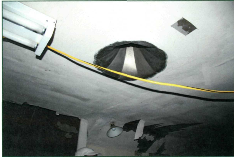
Figure 102: Northeast part of ceiling in Room C showing signs of water damage in the white paper covering (NPS July 2009).
