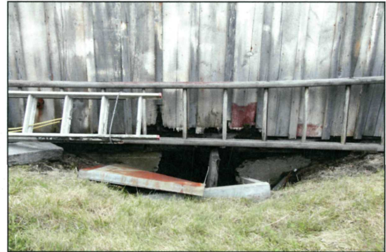
Figure 72: Cave-in along west side beneath section A-2 (NPS July 2008).
