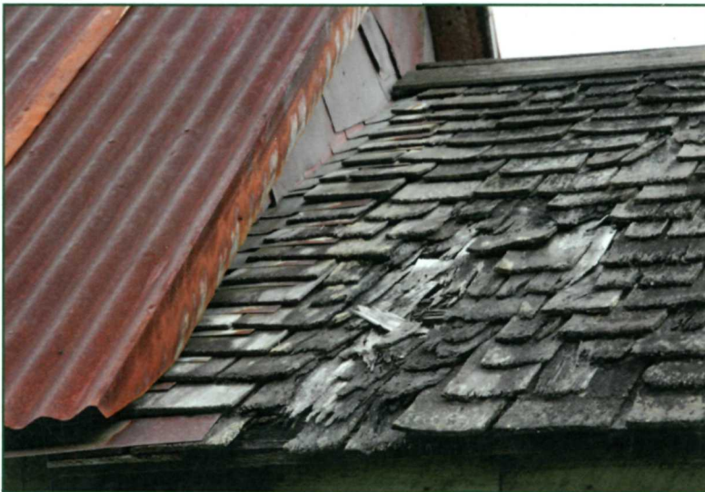
Figure 87: Eave connection at southeast corner of roof section A (shingles) and northeast corner (rusted metal) of roof section B. Note the damaged shingles (NPS July 2008).
