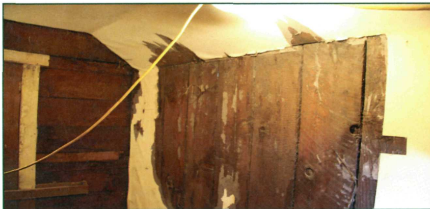
Figure 103: Southwest corner of Room C showing walls in fair condition and white paper covering on ceiling and portion of east wall (NPS July 2009).
