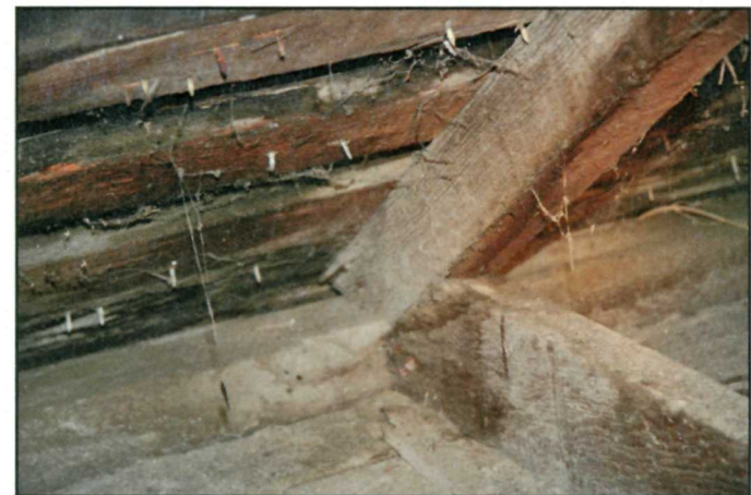
Figure 120: Attic A-1 rafters ends at top plate (NPS July 2008).
