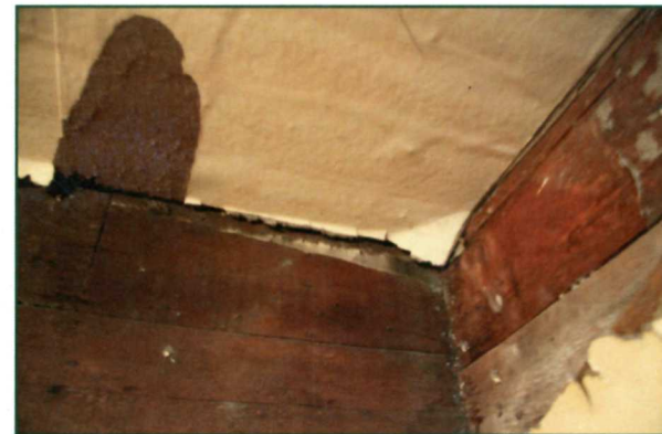
Figure 101: Ceiling and wall in northeast corner of Room B, notice minor bubbling in white paper ceiling (NPS July 2009).
