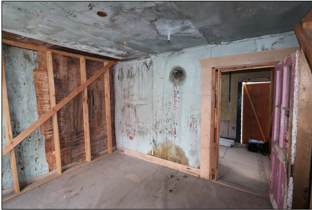
Figure 11: Alaska Street Crib, front chamber showing metal thimble, 2019 Source: Field Photograph by John Wachtel, Historical Architect, AKRO, HABS fieldwork, NPS, KLGO, IMG_6701.
