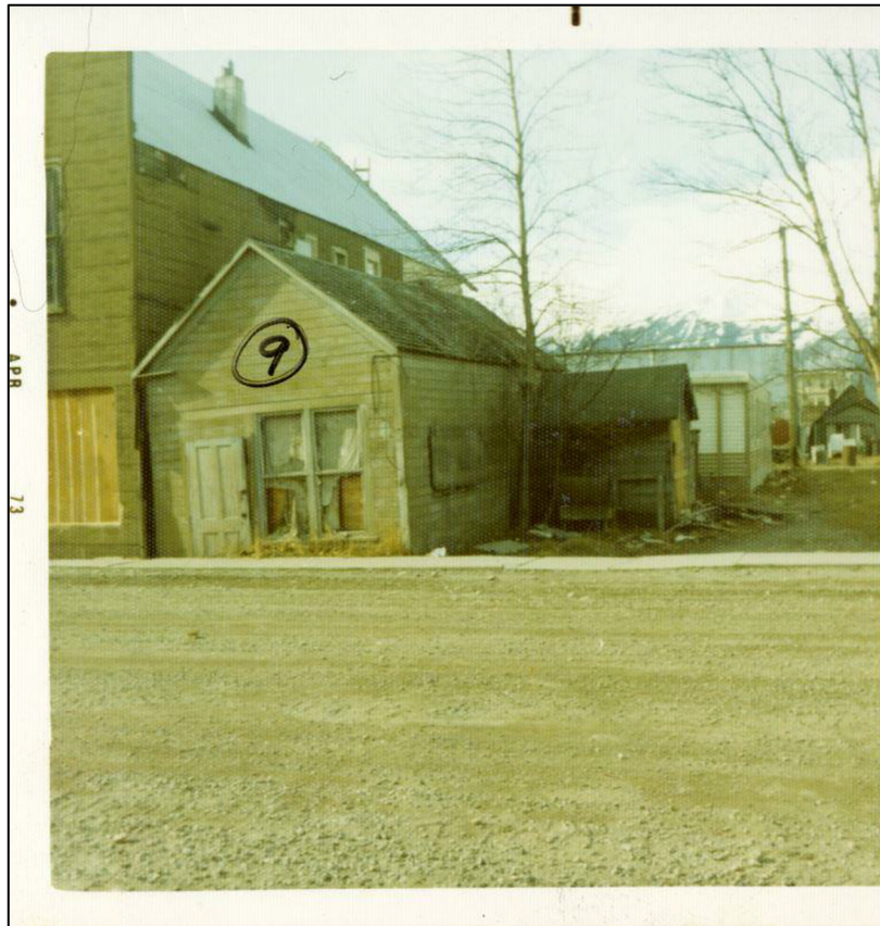
Figure 6: Front elevation of store, showing door and window no longer align, April 1973.
