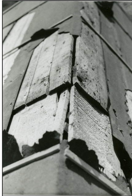
Figure 1: Roof patch on Goldberg Cigar Store and Confectionery, circa 1972, showing previous roof opening that likely accommodated a stove pipe.
