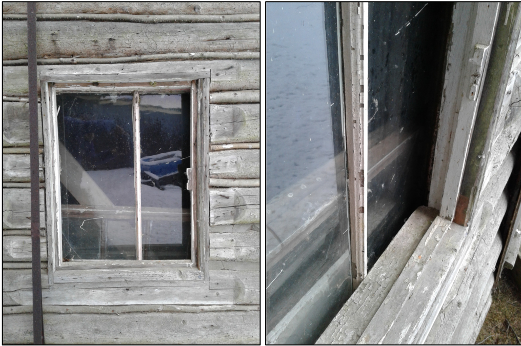
Figure 12: North elevation window, left of the door, showing window leaning against opening Source: Field Photograph by Anne E. Matsov, Chief of Resources, KLGO, 2019 20191203_133202 and 20191203_133145
