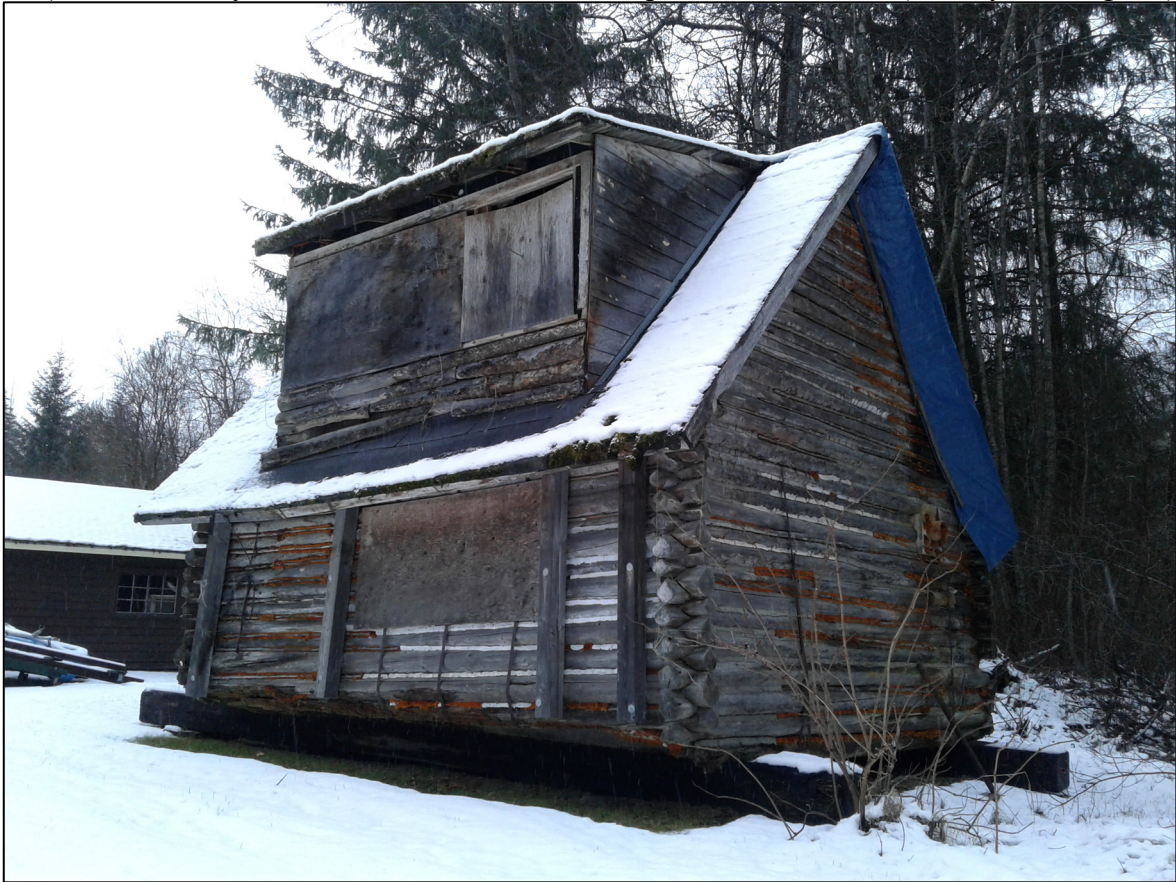
Figure 2: Southwest corner of Patterson-McDermott Cabin, showing McDermott era dormer Source: Field photograph by Anne E. Matsov, Chief of Resources, Klondike Gold Rush National Historical Park (KLGO), 2019 20191203_133310
