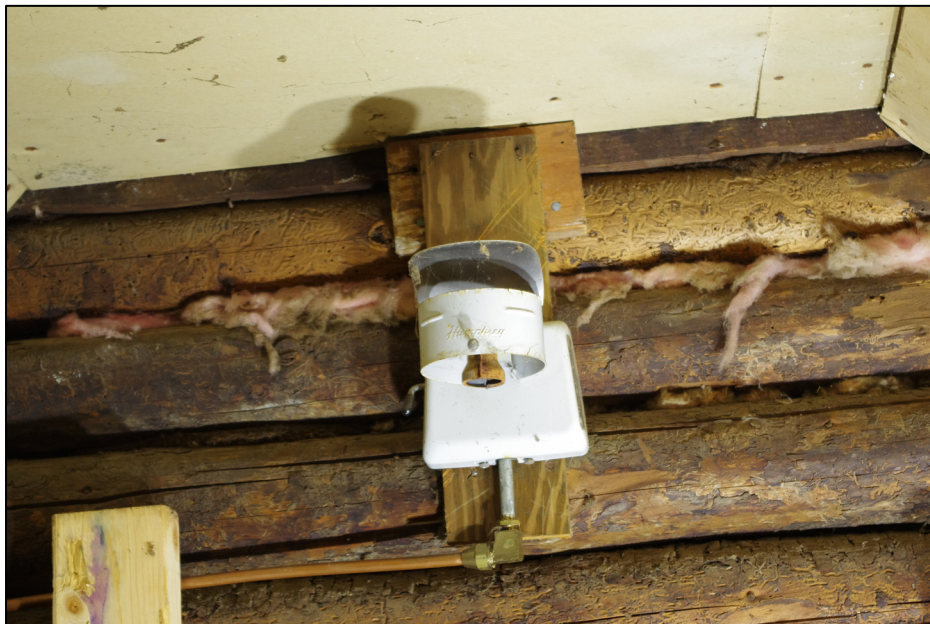
Figure 17: Remaining light fixture
