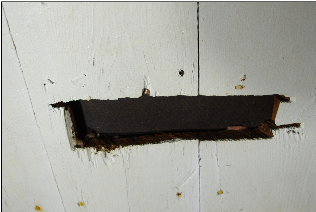
Figure 15: Rectangular cut out on ceiling of first floor, evidence of well point theft Source: Field photograph by Kathleen Wackrow, NPS, April 2016, NPS, AKRO, Historic Architecture, Patterson Cabin Digital Files IMGP6281
