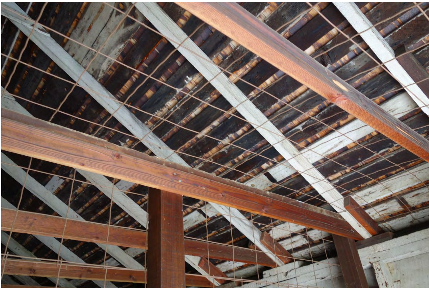
Photo 16: Carriage House interior. Note the differing stain patterns on the exposed roof skip sheathing. Camera facing southwest. Christopher E. Johnson, April 9, 2018.
