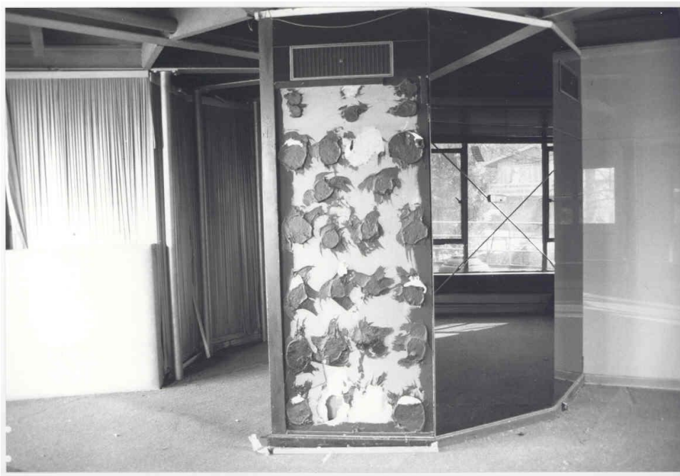
View 4 - Central Core – Note the use of Black and Gray Carrara glass, and the missing glass.
