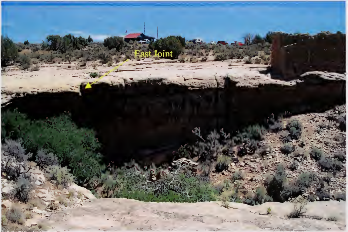
Photograph 2-1: View of joint on east side of Little Ruin Canyon.
