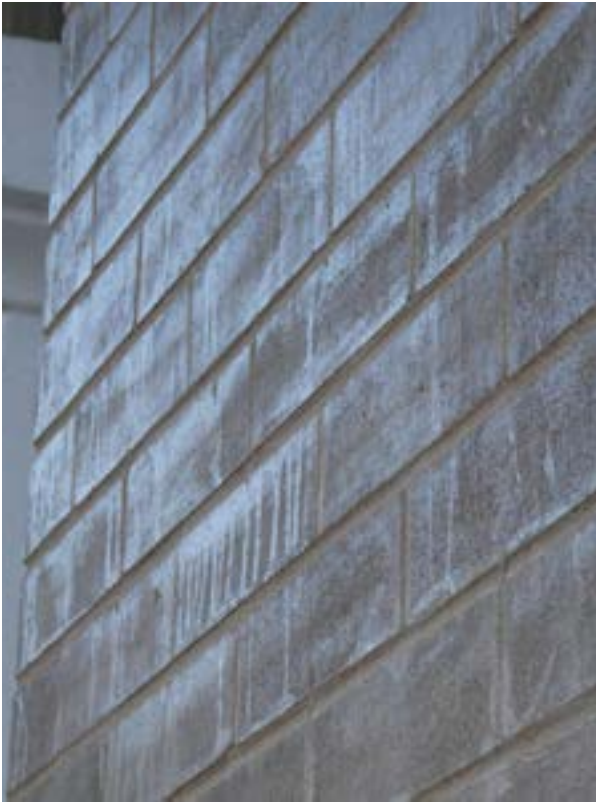
Figure 1.D.34. What appears to be evidence of a clear sealer on the blonde ironspot brick.
