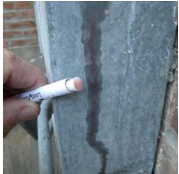
Figure 1.D.63. The red color reveals the base steel is coated with lead.
