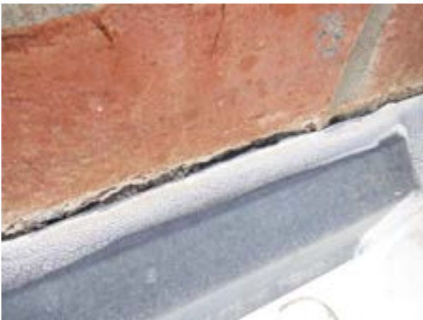
Figure 1.D.45. The sealant joint at this interface has typically failed.
