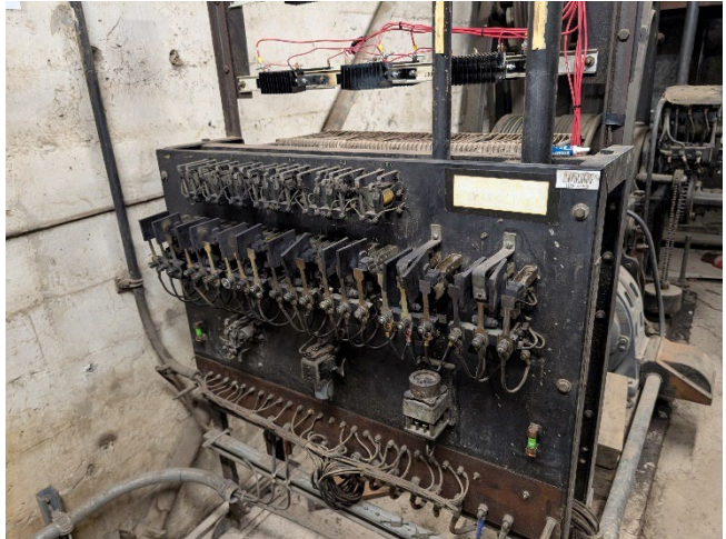
Elevator relay logic controller components
