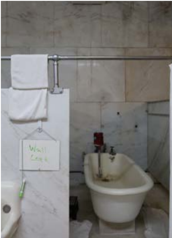
Figure 1.D.67. Staining of marble wall panels at north wall of men's bath hall (106) from plumbing leak.
