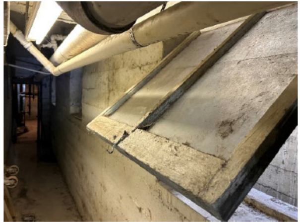
Photo 2 RACM window glazing observed on basement windows HA-7.
