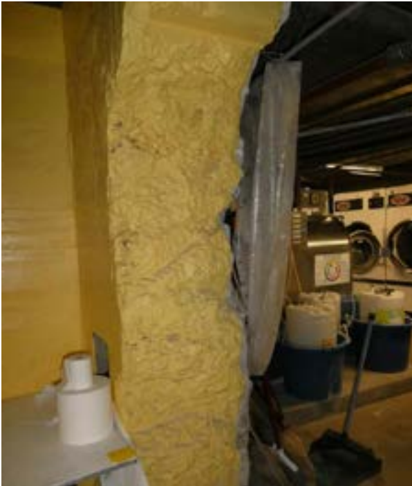
Figure 1.D.13. There is no evidence of any reinforcing steel where portions of this concrete wall were removed.
