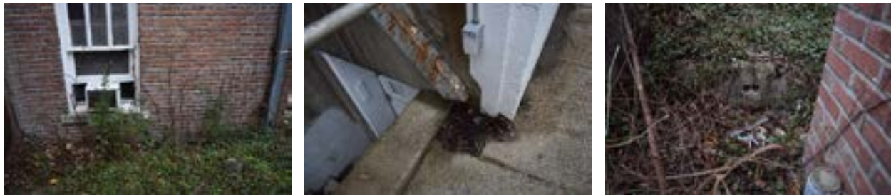
Figure 1.D.2. Areas with drainage concerns typically have debris buildup and degraded concrete. The proximity of the building to the retaining wall east of the bathhouse makes facilitating positive drainage difficult (WLA Studio, 2025).
