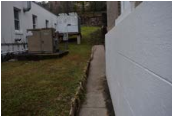
Figure 1.D.100. Electrical and HVAC equipment on the north side of the building (WLA Studio, 2025).
