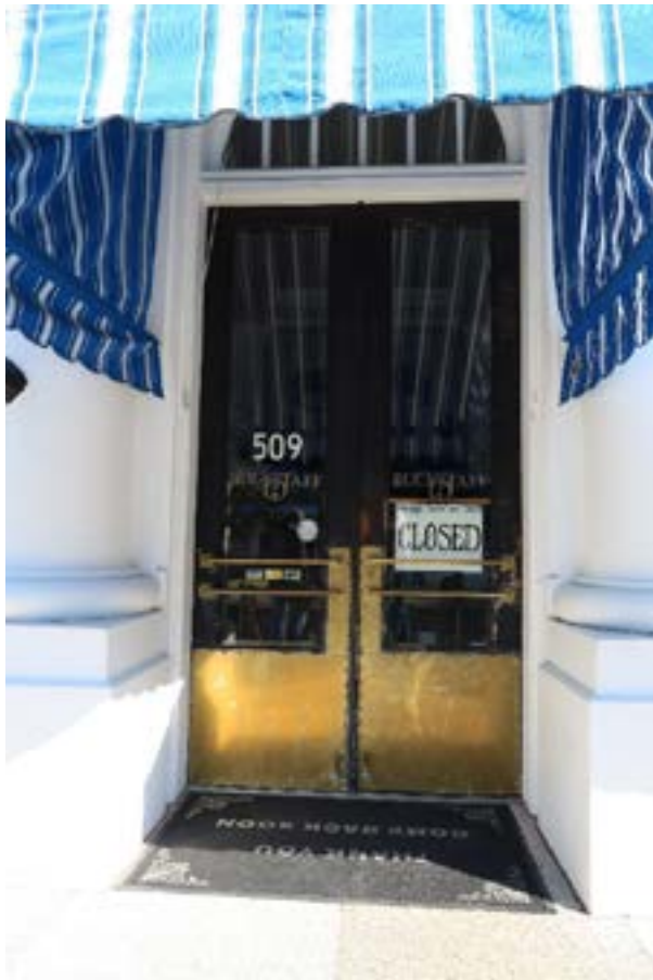
Figure 1.D.56. Front doors, showing wear to finishes.
