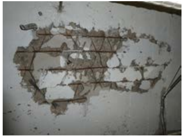
Figure 1.D.26. Portions of the concrete have fallen in this location exposing the slab reinforcement.
