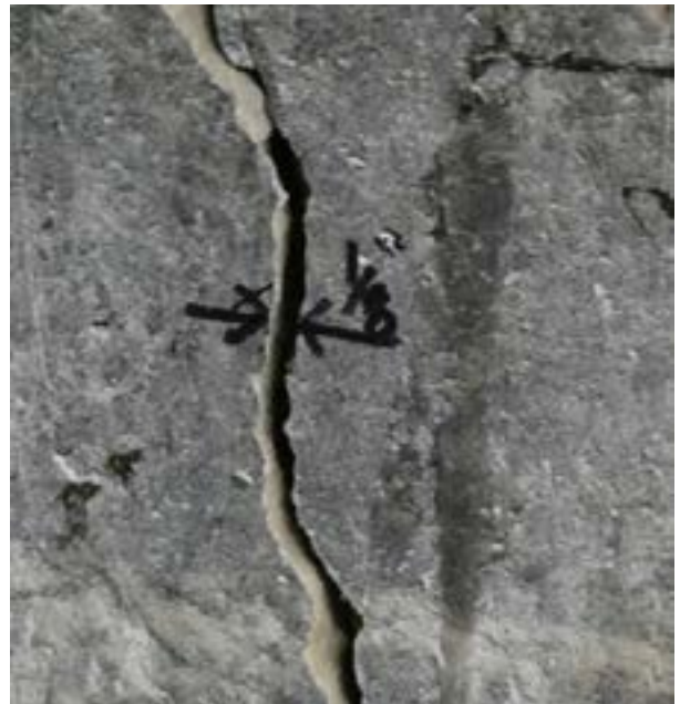
Figure 1.D.17. The widest portion of the crack was measured to be 1/8 inch.
