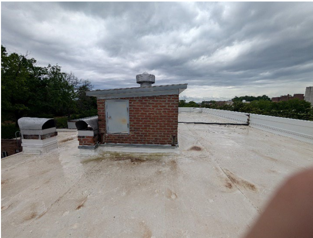
Top of Hoistway Access
