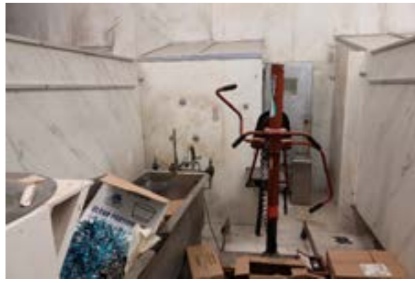
Figure 1.D.68 Mineral accumulation and staining at marble wall panels and partitions in men's bath hall (106).
