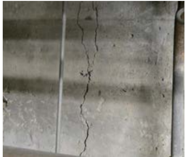
Figure 1.D.16. Crack in an interior concrete wall in the crawlspace, which is load bearing. This occurs under a girder connection.
