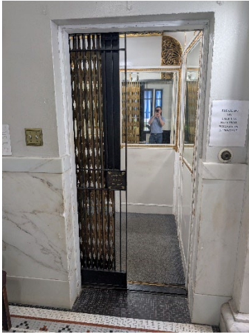
Floor 1 Hoistway Entrance
