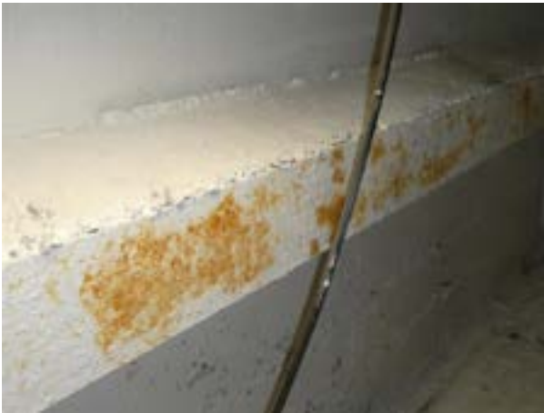
Figure 1.D.24. Slight corrosion bleeding through the paint in another location in the basement.
