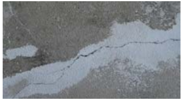
Figure 1.D.15. A cementitious material was buttered over some of the cracks on the exterior face of this wall.
