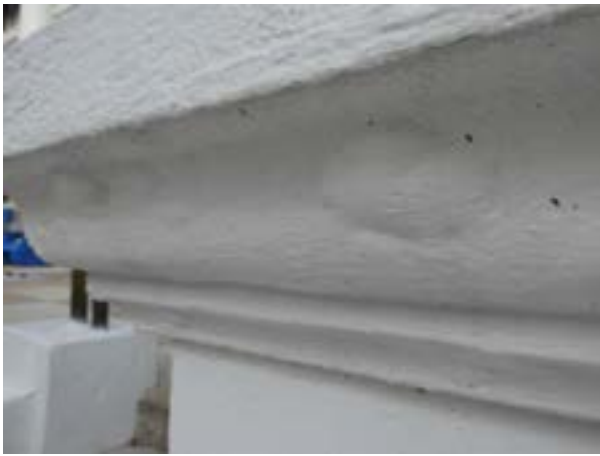
Figure 1.D.29. Blisters in the coating were observed in a few isolated locations around the porch.
