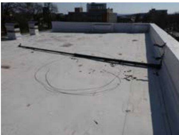
Figure 1.D.51. The flagpole has fallen onto the upper roof.
