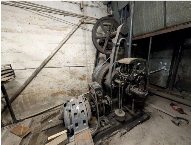
Otis basement-set winding drum machine
