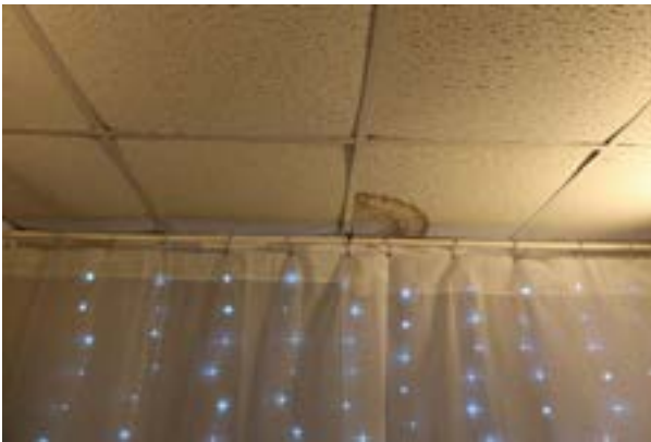
Figure 1.D.70. Non-historic suspended ceilings are in fair condition, with staining from leaks and typical and sagging cupping of aging acoustical tiles.
