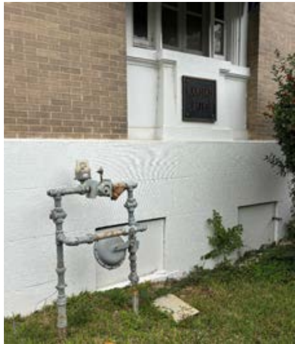
Figure 1.D.101. Gas meter at northwest corner of the Bathhouse (RATIO, 2025).
