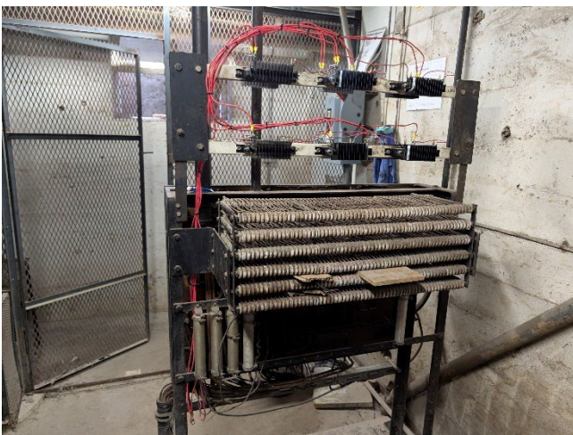
Elevator relay logic controller components
