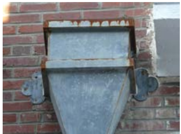
Figure 1.D.62. The original collector heads and downspouts are also made of terne metal. The base steel is beginning to corrode.
