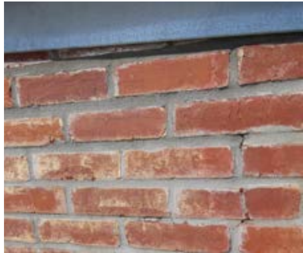
Figure 1.D.41. The mortar joints in the top of the elevator hoist are in poorer condition.
