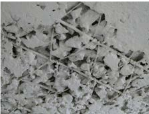
Figure 1.D.25. Slab reinforcement visible in the basement where honeycombing occurred during construction.
