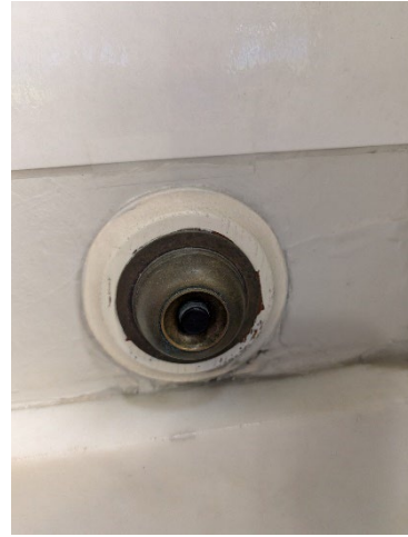
Elevator Push Button
