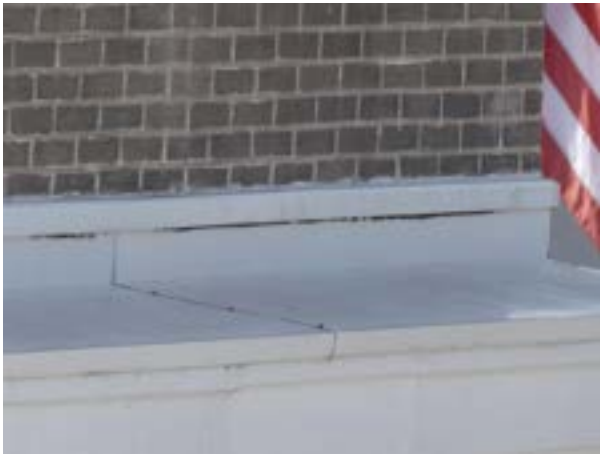
Figure 1.D.50. Gaps are visible in the counterflashing.
