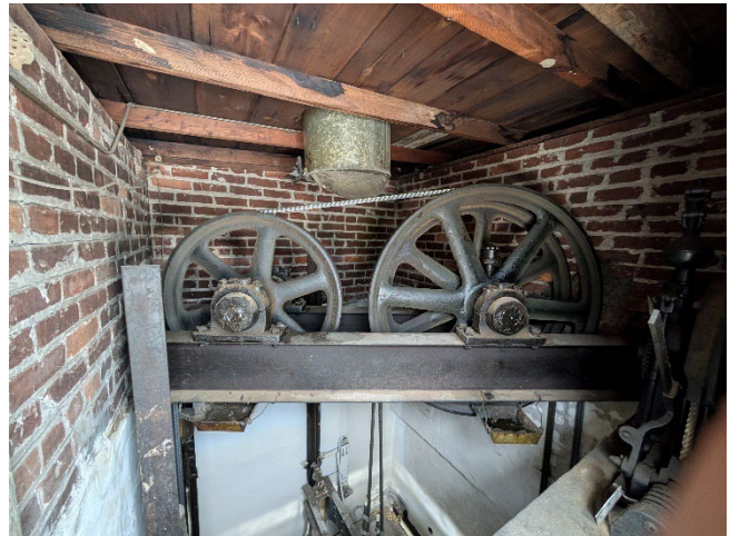
Top of Hoistway Sheaves
