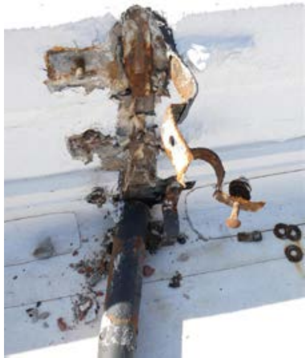
Figure 1.D.52. Failure of the metal brackets which originally screwed the base of the pole to the back of the masonry parapet.
