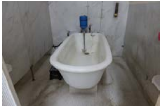
Figure 1.D.73. Mosaic tile floor in men's bath hall (106) showing typical mineral accumulation around plumbing fixtures.
