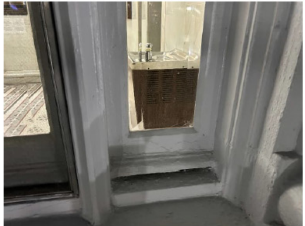
Photo 4 ACM Exterior caulking around windows and doors HA-9.
