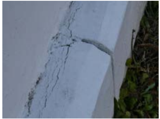
Figure 1.D.28. Minor cracking was observed in the concrete walls supporting the porch on the east elevation of the building.
