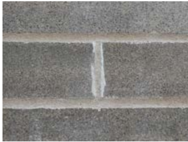
Figure 1.D.32. All of the mortar joints have been cut out and repointed. In general, they are in good condition but there is evidence of a lighter colored cementitious material on portions of the brick. This is probably a remnant of a previous repair effort where the mortar joints were "masked and grouted."
