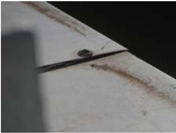
Figure 1.D.49. Gaps in this lap may allow wind driven rain to infiltrate under the metal.
