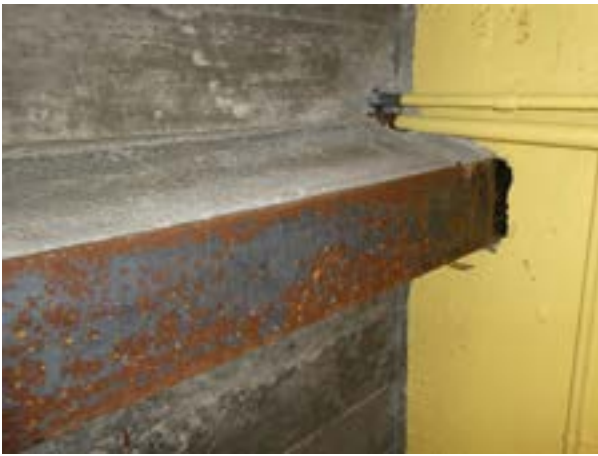
Figure 1.D.23. Slight corrosion on the bottom flange of a steel beam in the basement.
