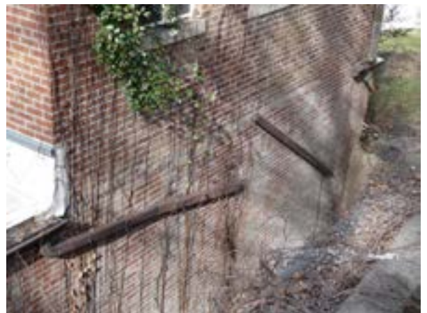
Figure 1.D.64. One of the more recent aluminum downspouts has failed.
