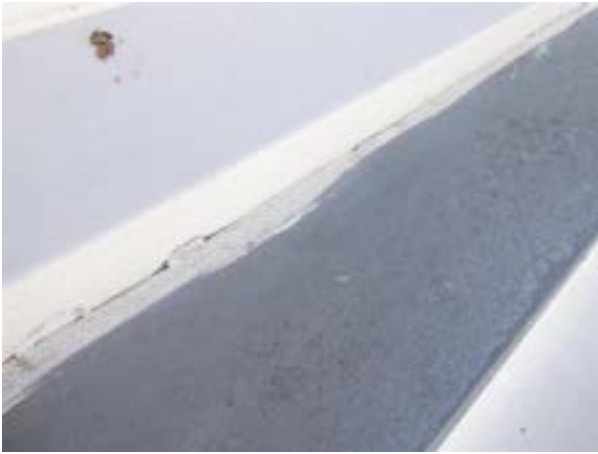
Figure 1.D.43. Sealant joints are often beginning to debond.
