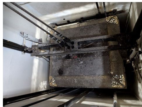
Top of Elevator Car
