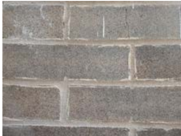
Figure 1.D.33. A location where the remnants of the "mask and grout" repair is much more evident.
