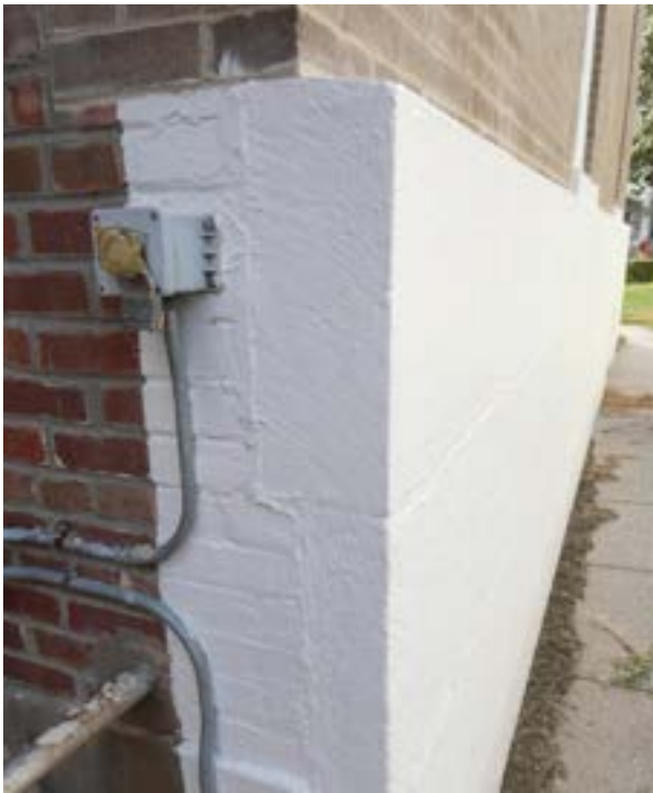
Figure 1.D.38. This is evident where the coating continues onto the adjacent brick.
