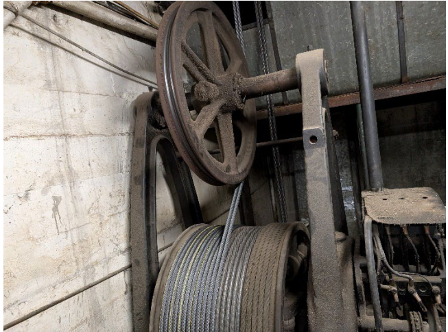
Otis basement-set winding drum machine
