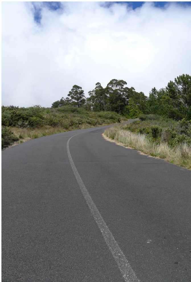
Circulation #1 Hosmer Spur Road towards Hosmer Grove, view northeast (NPS, September 2018).
