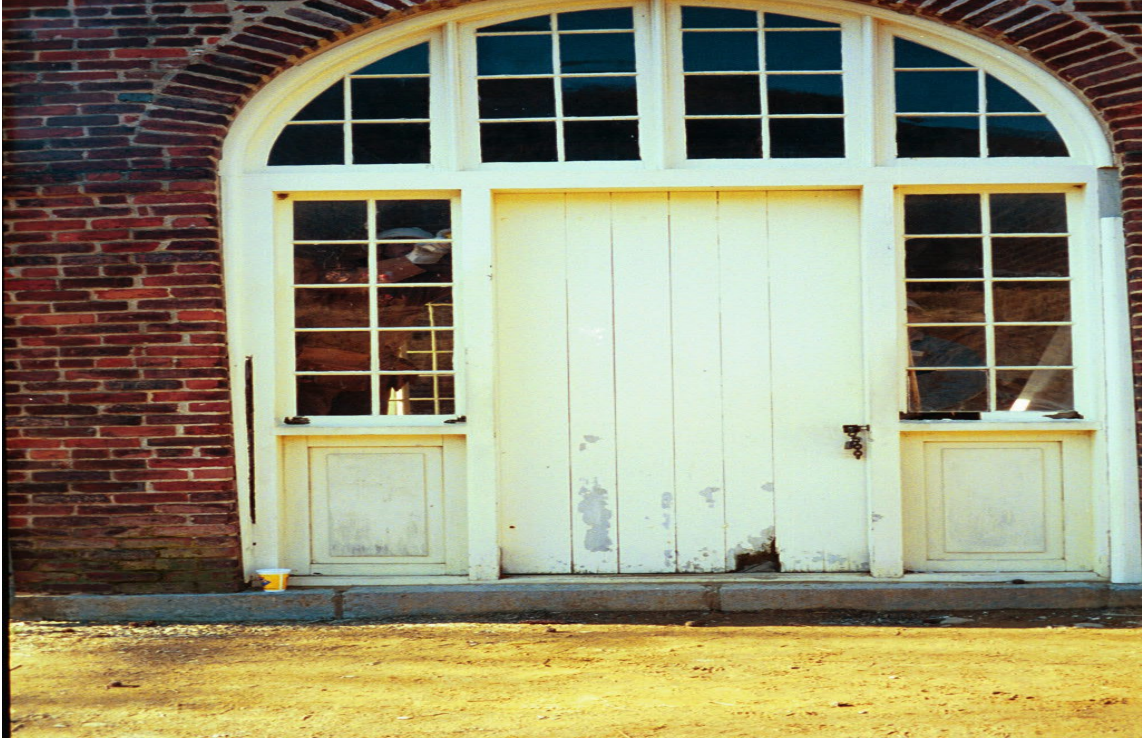
Photo 1: Guard Room Door (D101) and side-lites prior to repairs.
