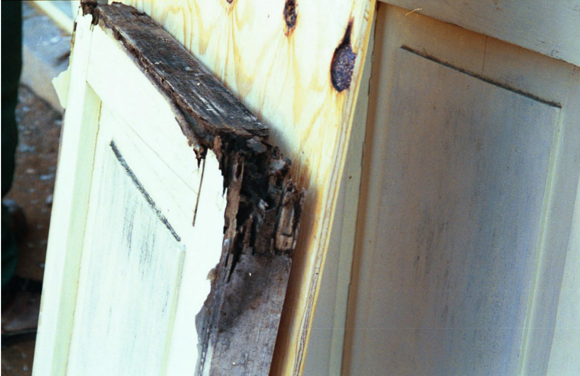
Photo 3: Moisture damaged side-panel from Guard Room Door.
