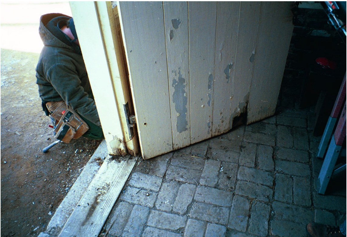
Photo 2: Deterioration of door jamb due to moisture damage.
