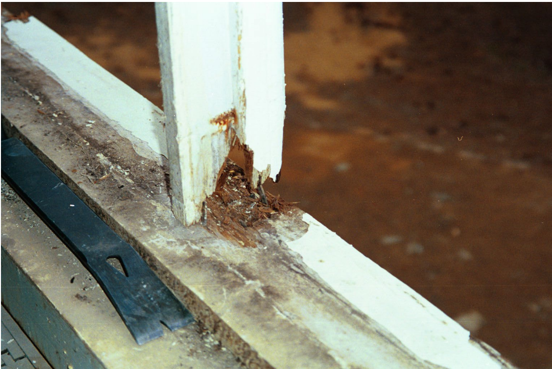
Photo 4: Deteriorated mullion and sill of WT103.
