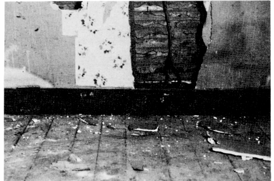
PHOTOGRAPH 65 (1981) North Wall, Room 201
