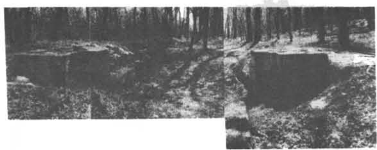
3 HEAD GATE - LOOKING SOUTH 29 (PRIORITY 1E)
