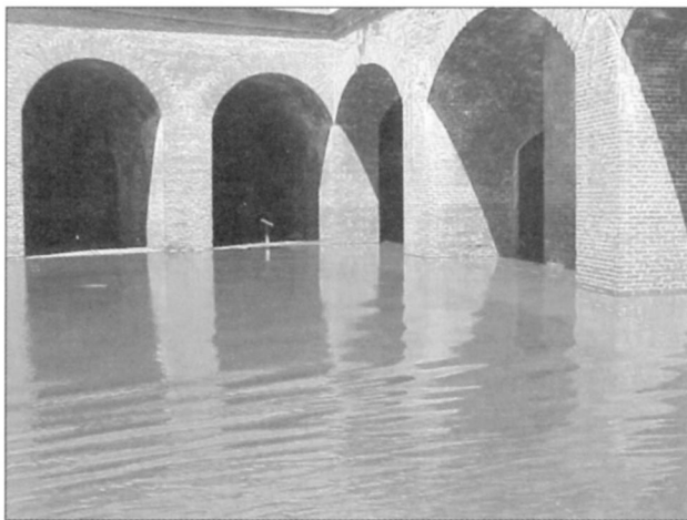
Fort Massachusetts, on West Ship Island in Mississippi, sustained flooding damage from Hurricane Ivan. It is now, as are all other Mississippi sites, open to the public.
