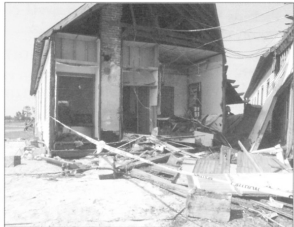
Building 5, where the Fort Pickens Museum and rangers' offices were located, was pushed off its foundation and split in half by the storm surge coupled with 130 mile per hour winds.
