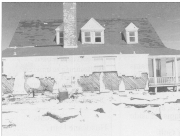
The Ranger Station received quite a bit of damage to the exterior as illustrated by this photograph. Information will be offered to camping enthusiasts at this ranger station once again when the Fort Pickens Area is reopened to the public.
