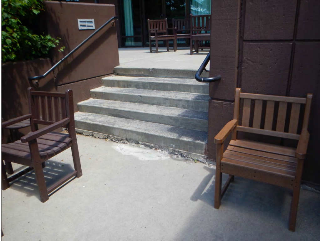
Photograph 2.19. Deteriorating concrete stairway outside of the Blue Heron Lounge, facing northeast, 2014 (Source: Logan Simpson).
