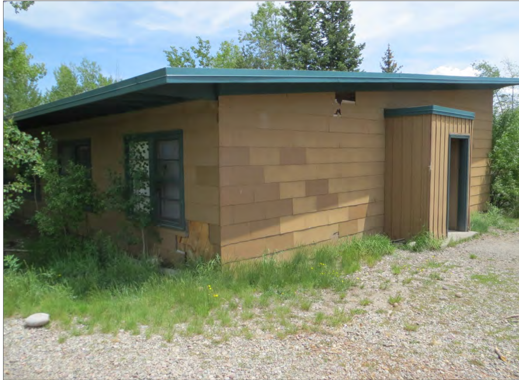
Photograph 2.7. Rear façade of Dorm #7 (JL-36), showing the replacement of original asbestos shingle siding with modern siding, facing east, 2014. Note the additional loss (visible at bottom left) and the warping of siding near the base of the projecting entry (Source: Logan Simpson).
