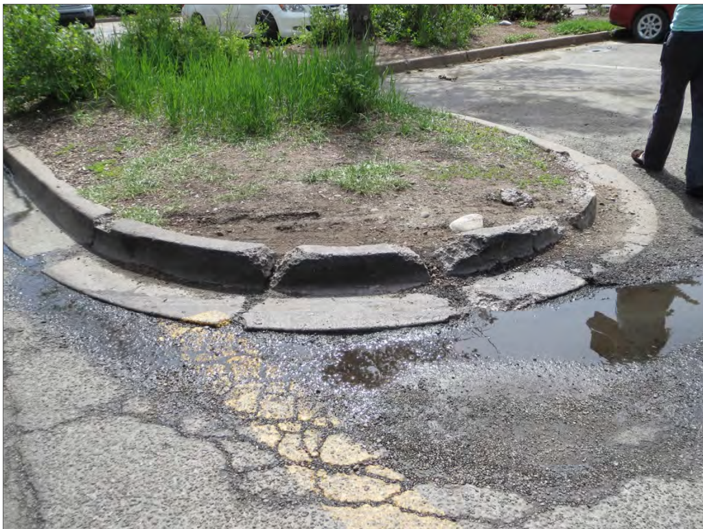
Photograph 2.16. Damaged concrete curb along one of the islands in the parking lot, facing southeast, 2014 (Source: Logan Simpson).
