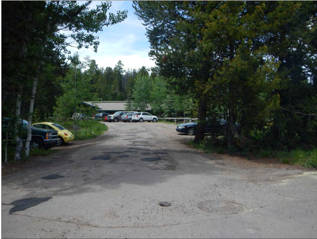
Photograph 2.15. Potholes and patched pavement near the northern end of Dorm Street, facing northwest, 2014 (Source: Logan Simpson).
