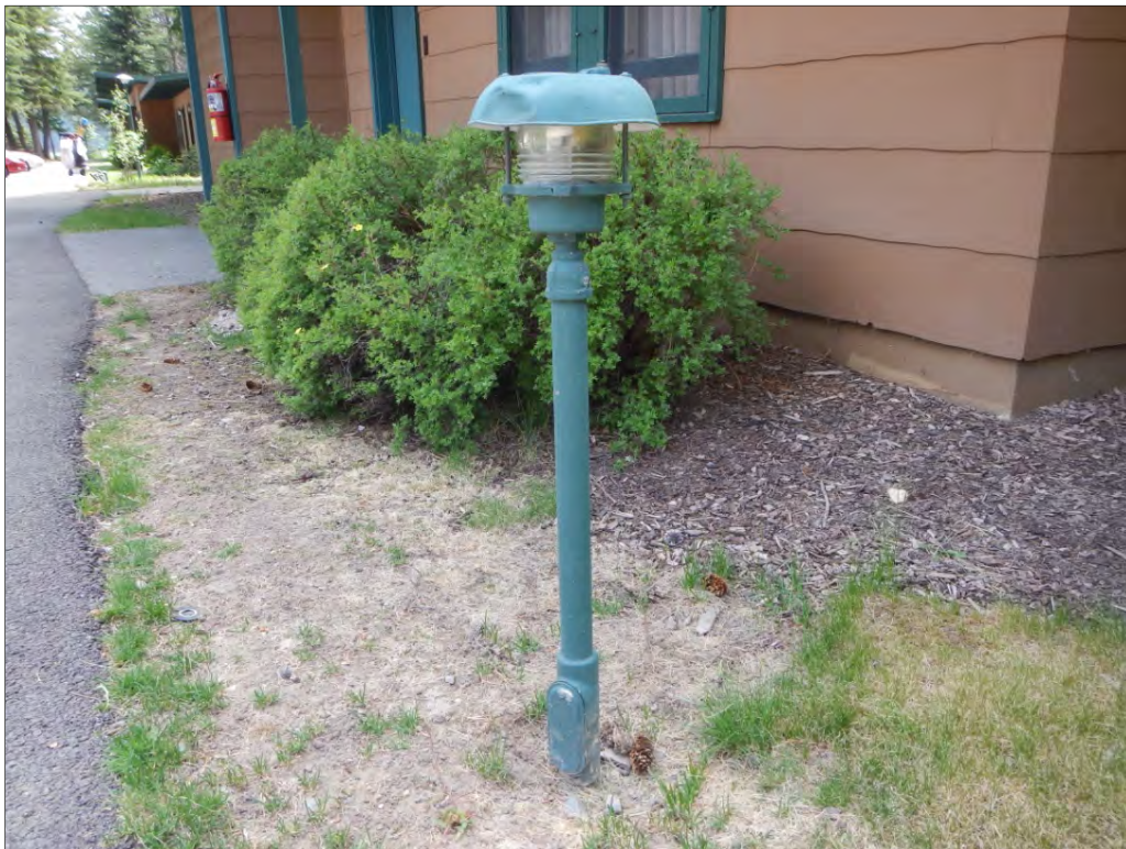
Photograph 2.24. Example of path light along a walkway in the south guest cottage area, facing southwest, 2014 (Source: Logan Simpson).
