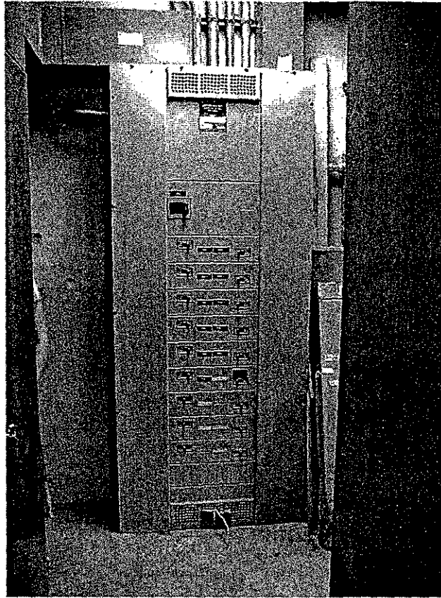
e: Main Electrical Distribution Panel
