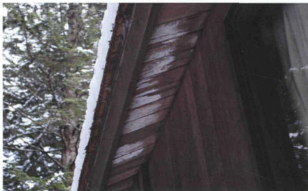
Figure 159. White stain beneath eave, March 2017.
