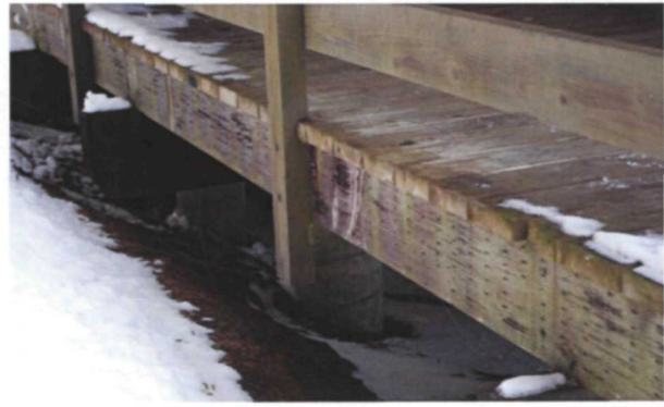
Figure 167. Mold on boardwalk, March 2017.
