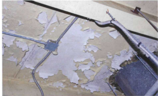
Figure 166. Paint peeling on utility room ceiling, March 2017.
