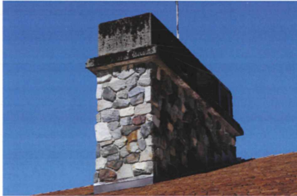
Figure 144. Biological growth on the chimney, May 2017.
