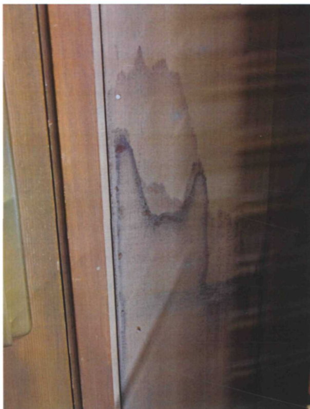
Figure 150. Water stains on cedar wall, May 2017.
