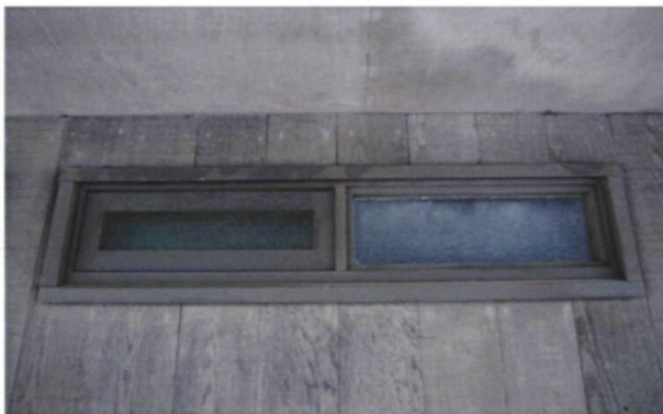
Figure 121. Bathroom window, March 2017.
