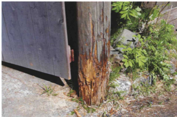
Figure 146. Damage to structural post, May 2017.
