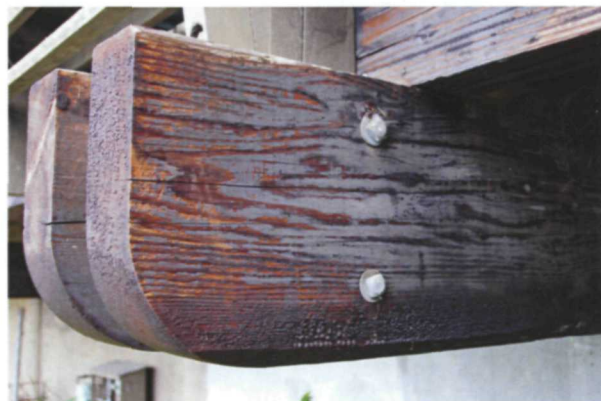
Figure 139. Moisture damage on girder, May 2017.
