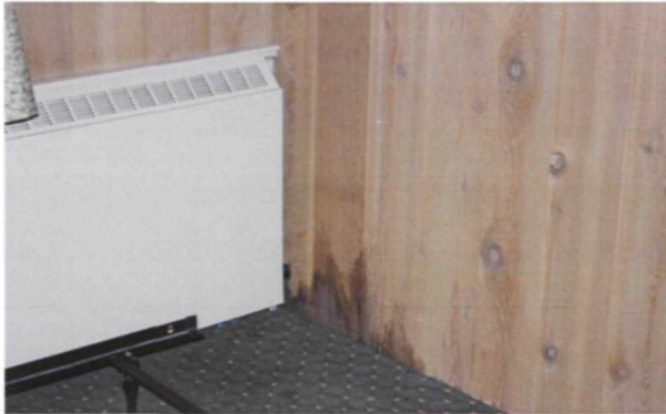
Figure 163. Moisture damage, March 2017.
