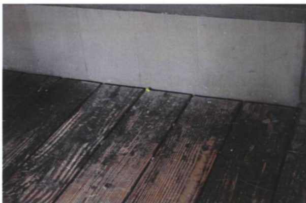
Figure 141. Cellar rot on deck, May 2017.
