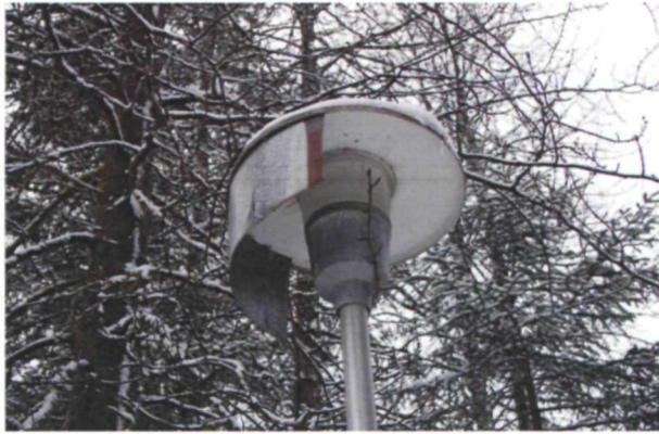
Figure 100. Outdoor lighting, March 2017.
