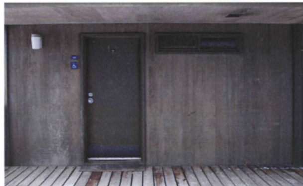
Figure 161. Mud backsplash on cabin, March 2017 wall cut
