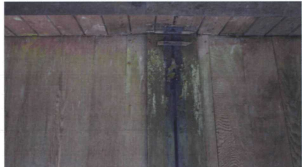
Figure 160. Metal screen for bat abatement with biological substance, March 2017.
