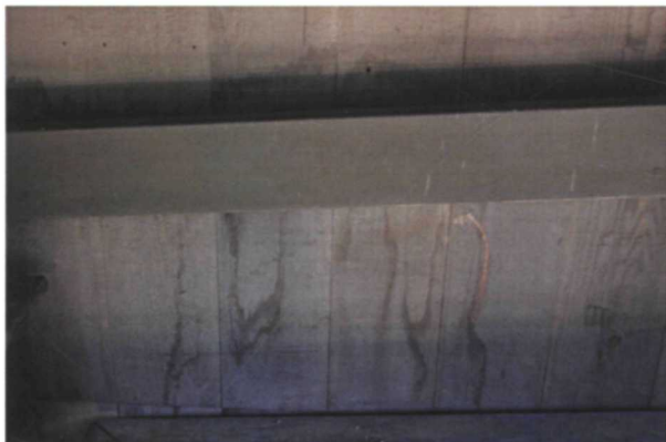
Figure 140. Moisture damage on siding, May 2017.
