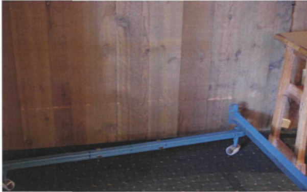
Figure 162. Dents in cedar wall, March 2017.
