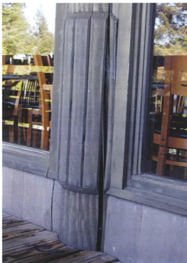
Figure 137. Crack on post, May 2017.
