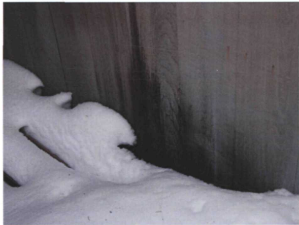
Figure 155. Moisture damage at wall-soffit joint, March 2017.
