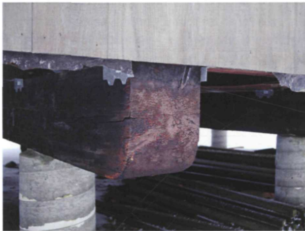
Figure 153. Blistering stain on cabin girder, March 2017.
