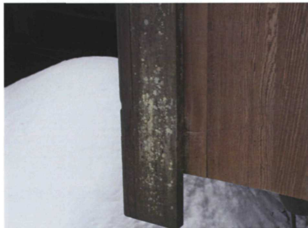
Figure 157. Moisture damage to corner board, March 2017.
