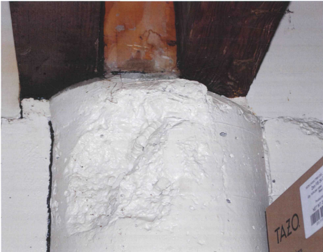
Figure 169. Spalling pier, May 2017.
