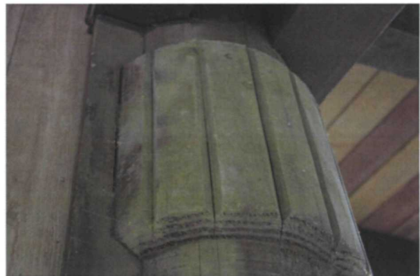
Figure 142. Green mold on concrete pier, May 2017.
