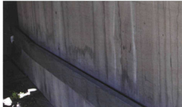
Figure 148. Mark across south elevation, May 2017.
