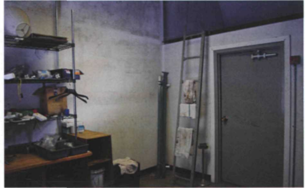
Figure 165. Mold in utility room, March 2017.
