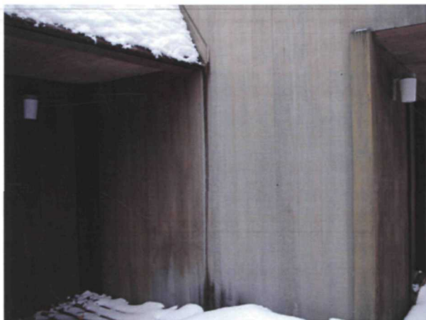
Figure 154. Moisture damage at wall-soffit joint, March 2017.
