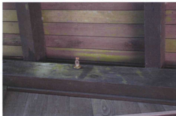
Figure 143. Green mold beneath eave, May 2017.
