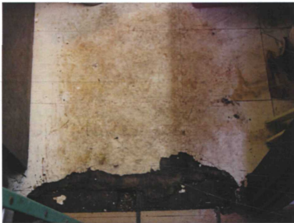
Figure 152. Loss of linoleum tiles of kitchen bathroom floor, May 2017.
