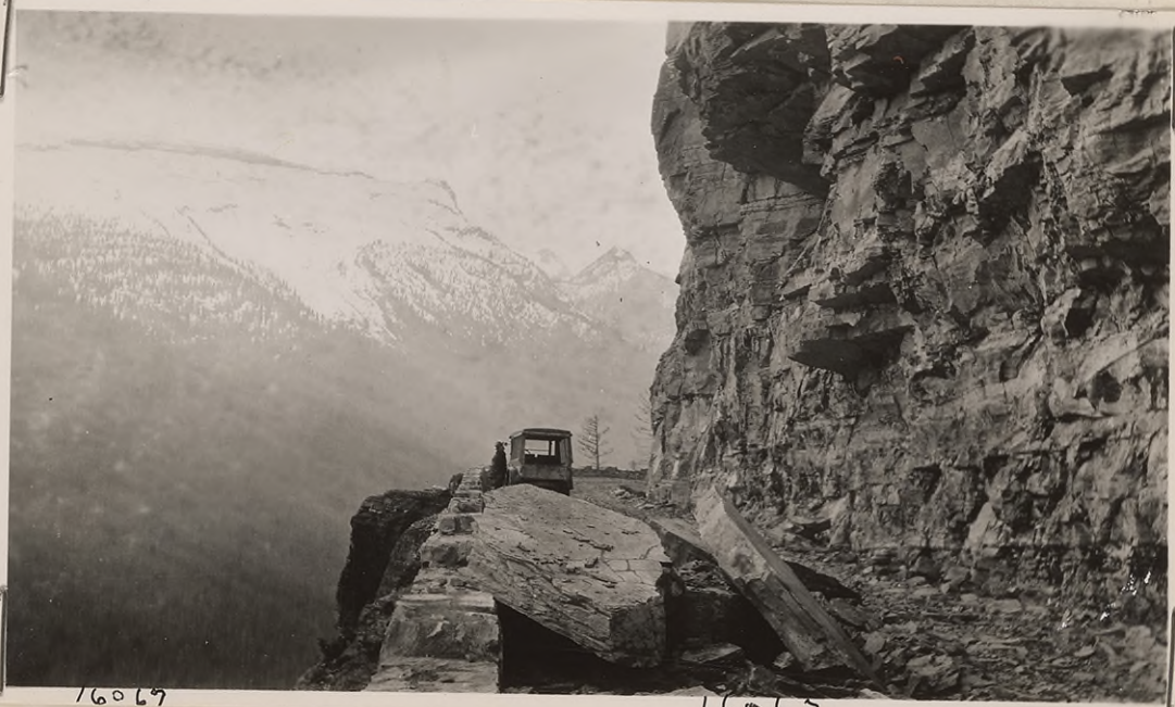
#16067 - Sta. 381 ahead. June 1928. Showing large rocks fallen from half tunnel or under cut section. A source of danger along cliff sections of highway. Very slight damage to wall.
