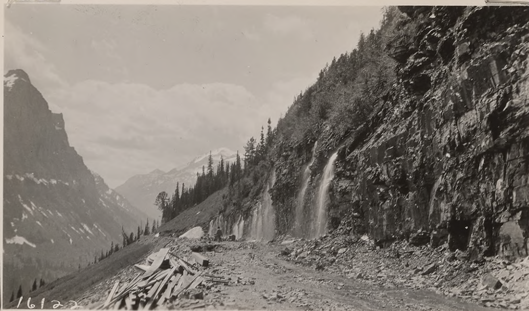
#16122 - Sta. 155 ahead showing water conditions along rock cut. Almost continuous sheet of water from Sta. 155 to 162, from snow field above. Wide, deep ditch with frequent culverts provide for run-off. June 23, 1928.
