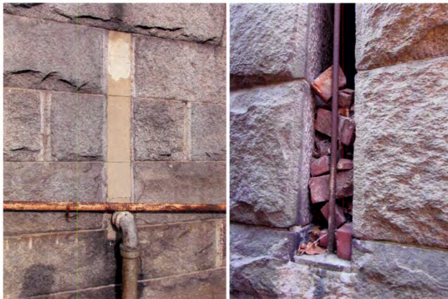
Figure 9: Embrasure infilled with concrete and a pipe (left) and embrasure infilled with debris (right).
