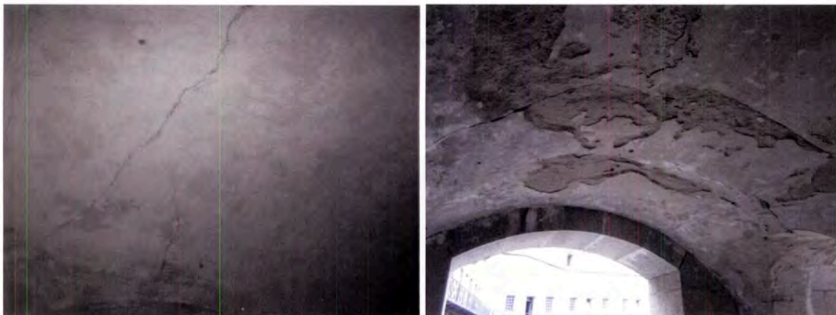
Figure 60: Crack in concrete roof (left) and concrete spalling (right).
