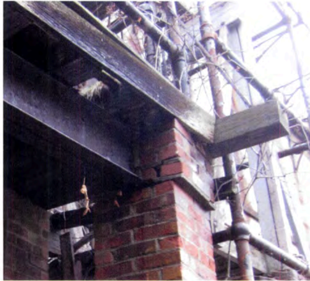
Figure 39: Cracked pillar at beam landing.
