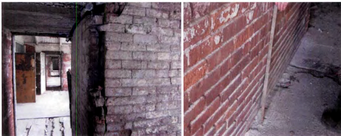
Figure 82: Broken door jamb (left) and bowing wall (right).
