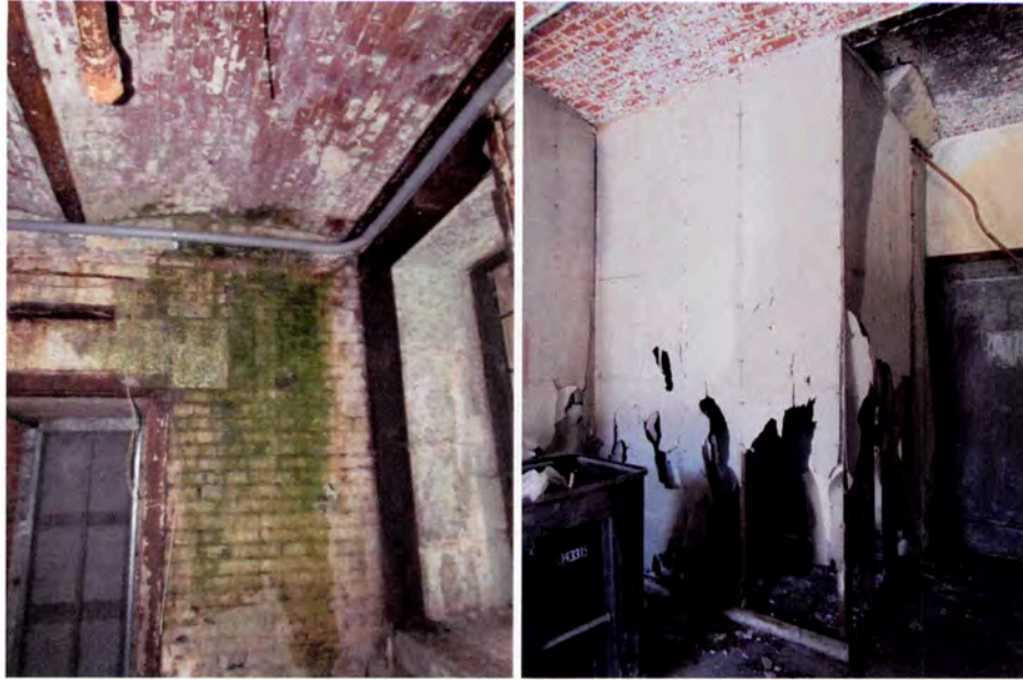
Figure 41: Water damage and severe staining on brick wall (left) and deteriorating plasterboard partitions (right).
