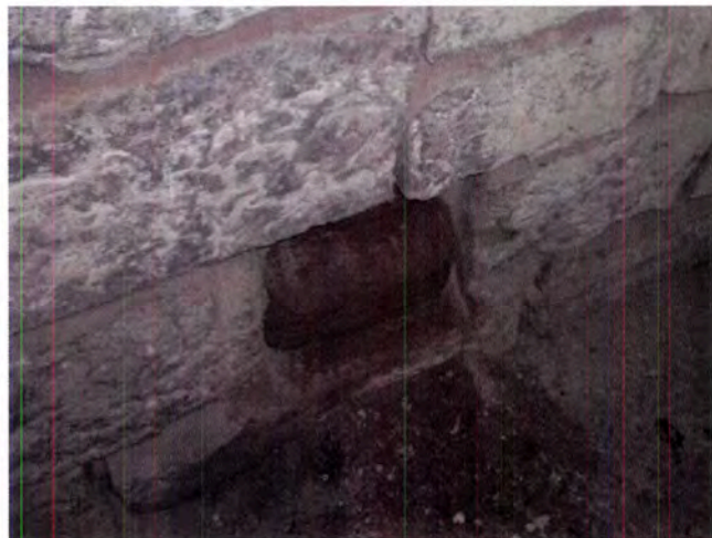
Figure 93: Pointing missing in wall (above) and deteriorating sandstone (below).
