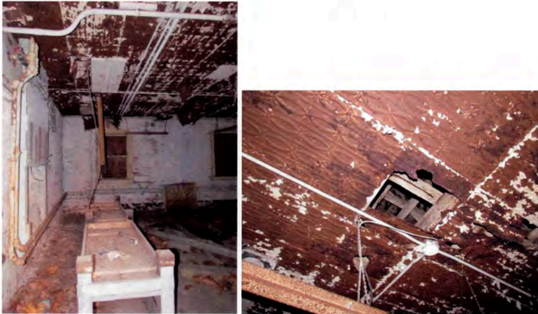
Figure 104: Overview of interior of Building 138 (left) and deteriorating metal roof (right).
