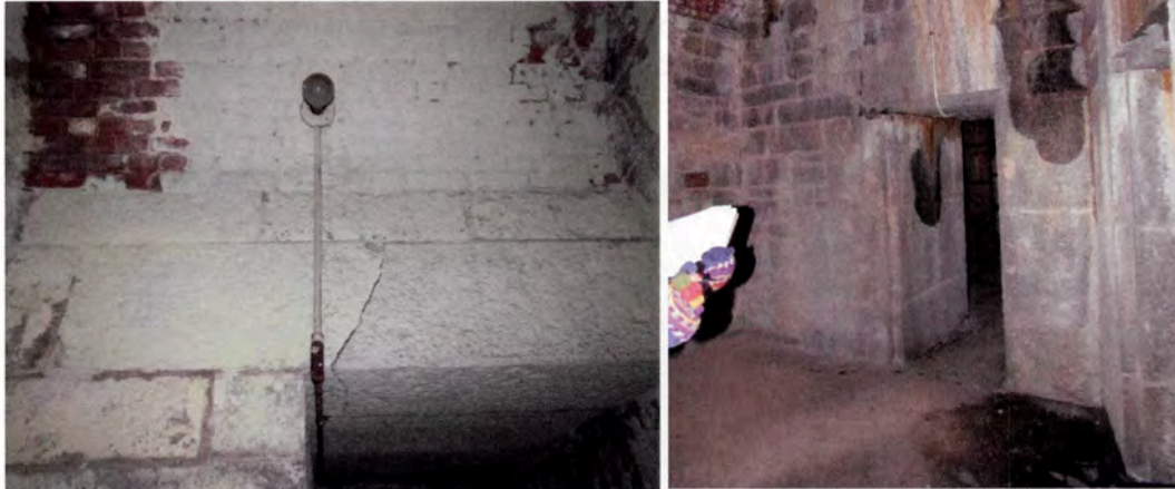
Figure 88: Crack in granite and deteriorating paint (left) and severe water damage on granite walls (right).
