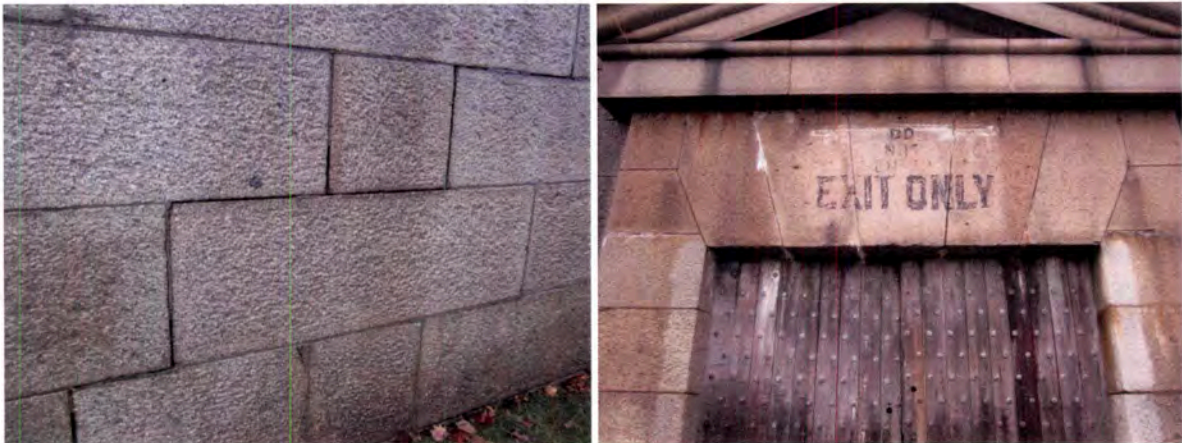
Figure 14: Diagonal crack in granite (left) and flat arch on east elevation (right).
