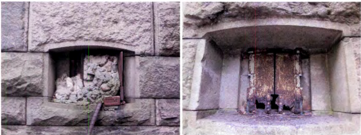
Figure 24: Infilled window (left) and rusted metal shutters (right) of Counterscarp.
