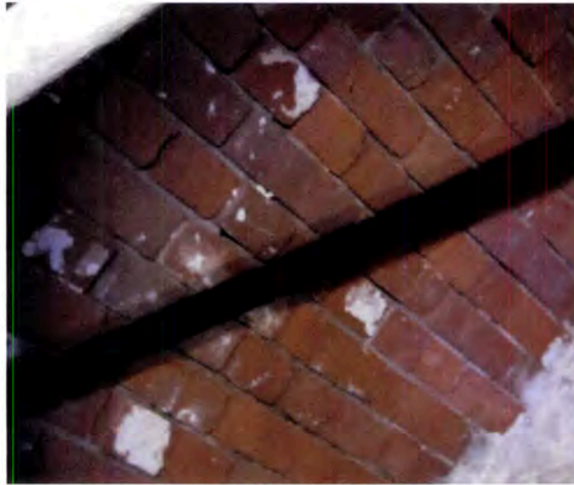
Figure 58: Brick arch with missing pointing in room 136A.
