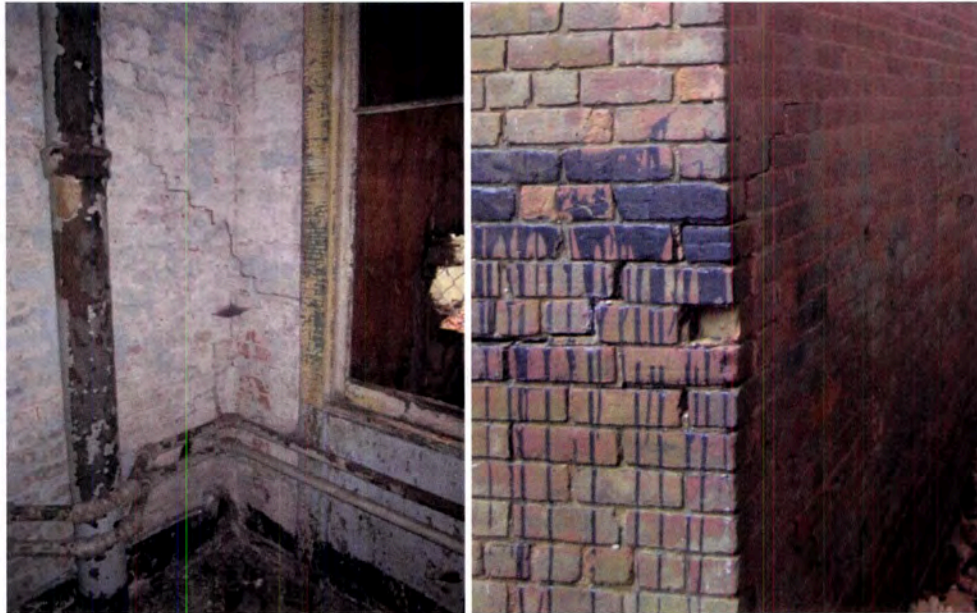
Figure 105: Diagonal crack in northeast corner of interior (left) and exterior (right) of Building 138.
