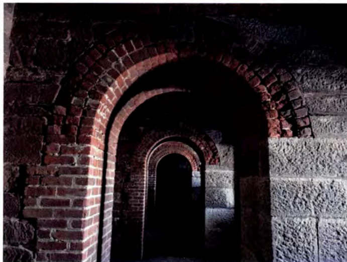
Figure 96: Brick and mortar deterioration at the northeast "tail" of the counterscarp.
