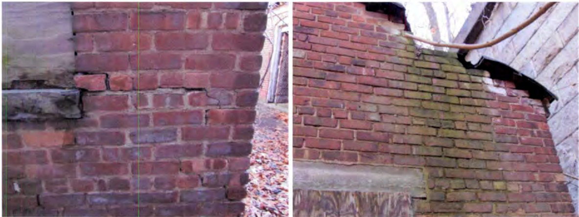
Figure 107: Stepped crack in masonry (left) and missing section of roof causing deteriorating conditions on the masonry (right).
