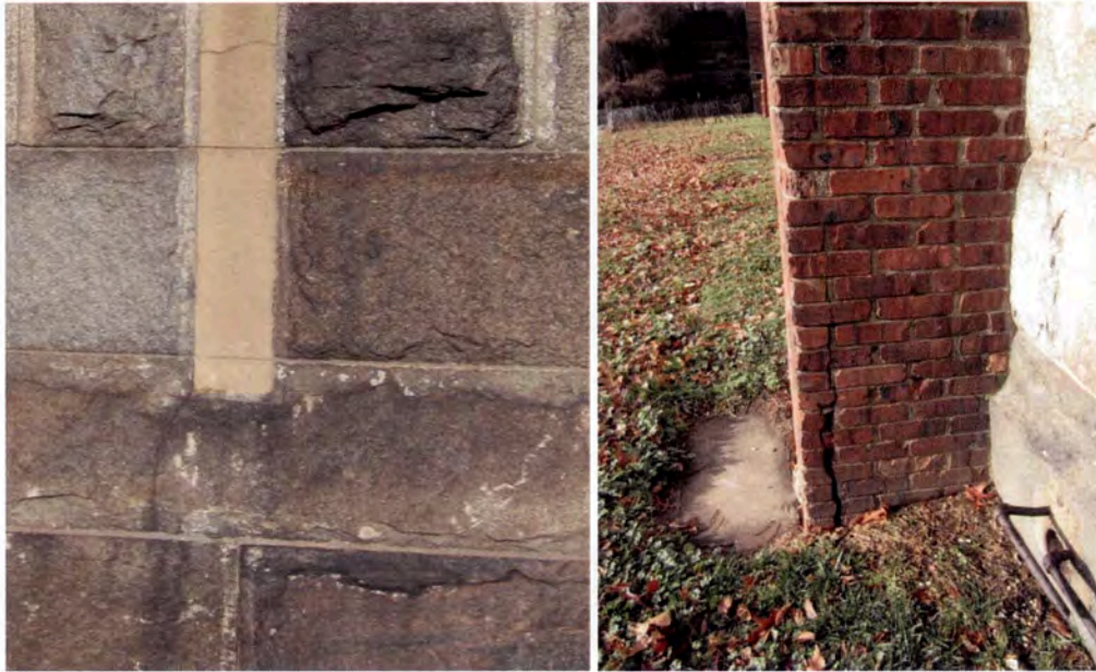
Figure 16: Crack below masonry opening (left) and crack at base of east chimney on south elevation (right).
