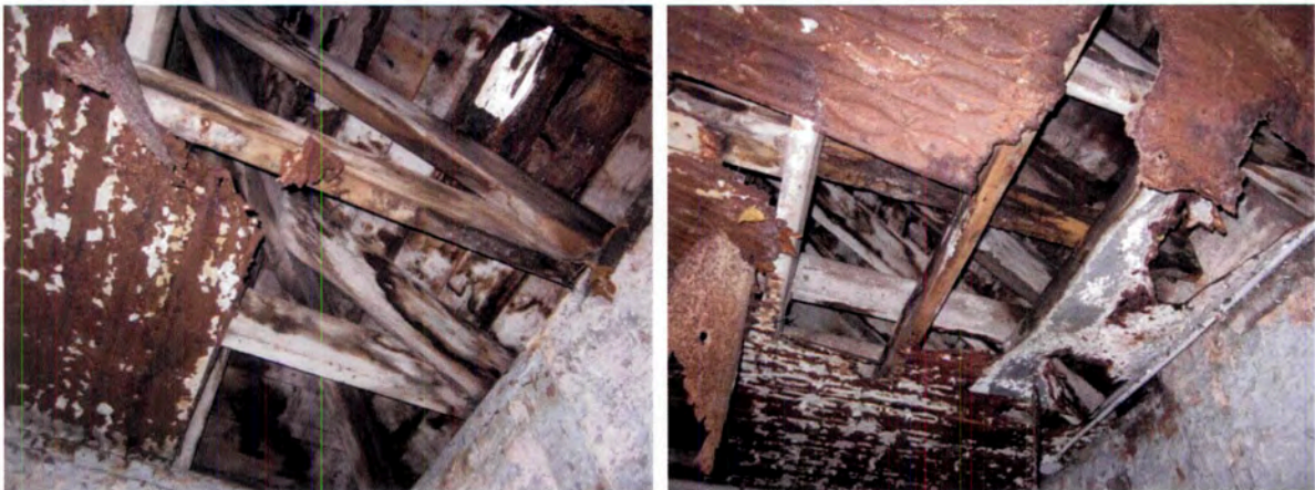
Figure 106: Holes and deteriorated wood in roof of Building 138.
