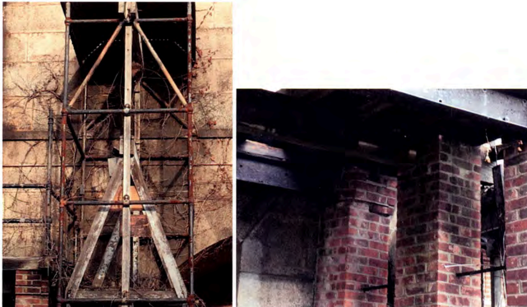
Figure 29: Rusted metal framing of lift structure (left) and detail of cracked brick column supporting platform.
