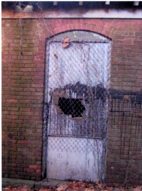
Figure 103: Large hole in plywood infill and paint stains on masonry of north elevation.
