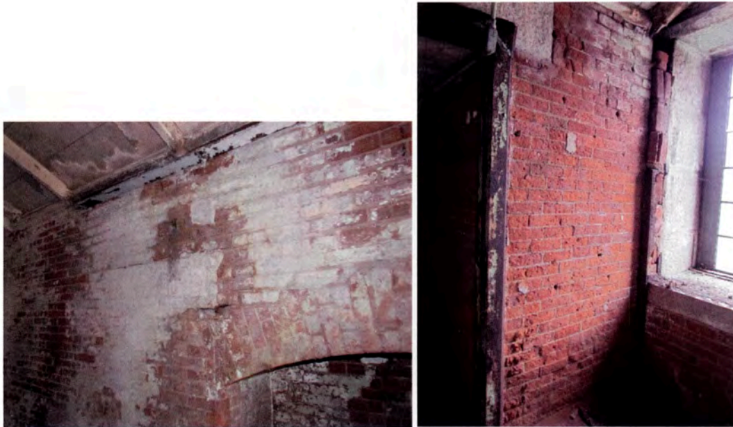
Figure 74: Deteriorating brick walls.
