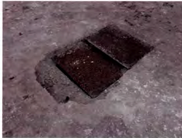
Figure 61: Hatch in floor with damage to concrete, missing frame and rusted hatch.
