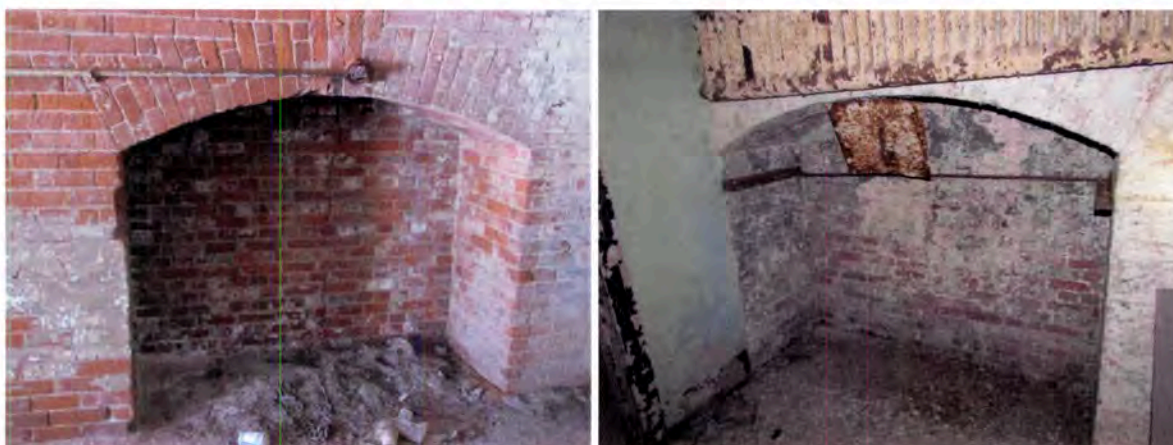
Figure 48: Brick fireplace with crack at back wall (left) and modified fireplace (right).
