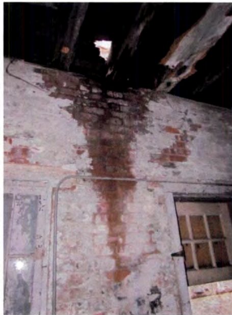
Figure 110: Hole in roof and water stains on brick interior wall.
