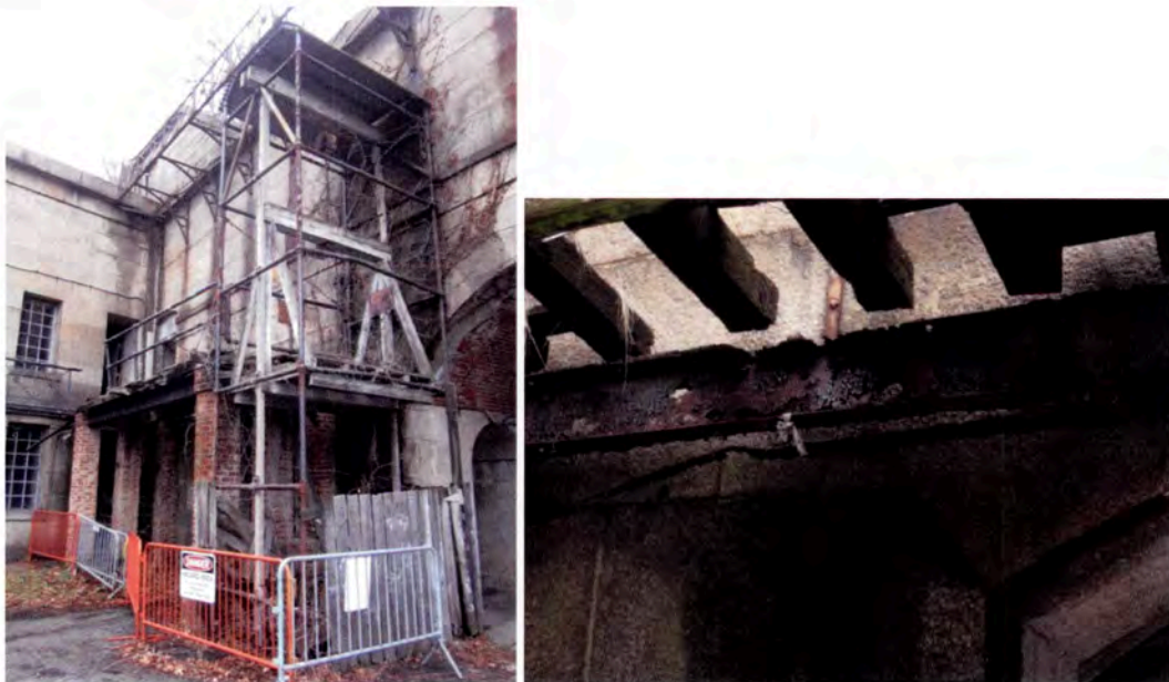
Figure 38: Hoist structure (left) corroded beam (right).
