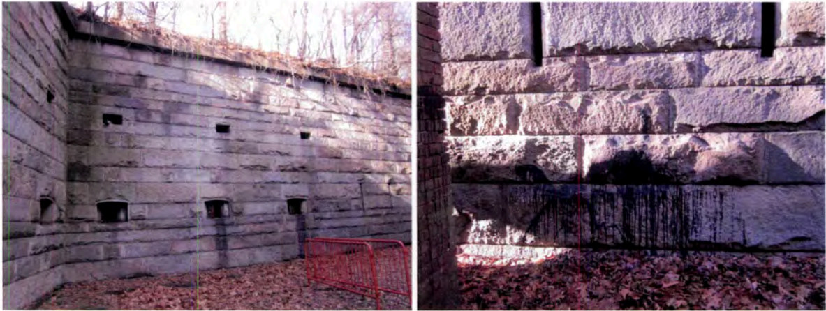
Figure 23: Staining under masonry openings (left) and paint stains (right) on south elevation.
