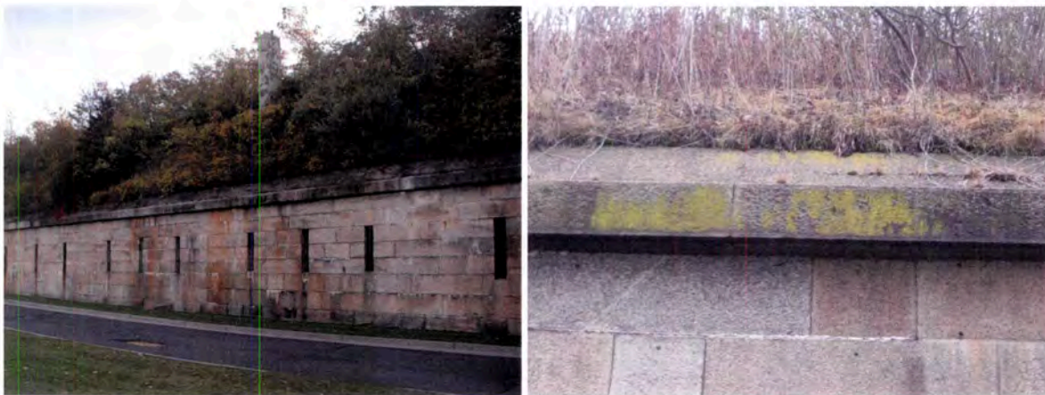
Figure 2: Severe stains on the smooth-face granite (left) and biological staining on the coping (right) of the east elevation.
