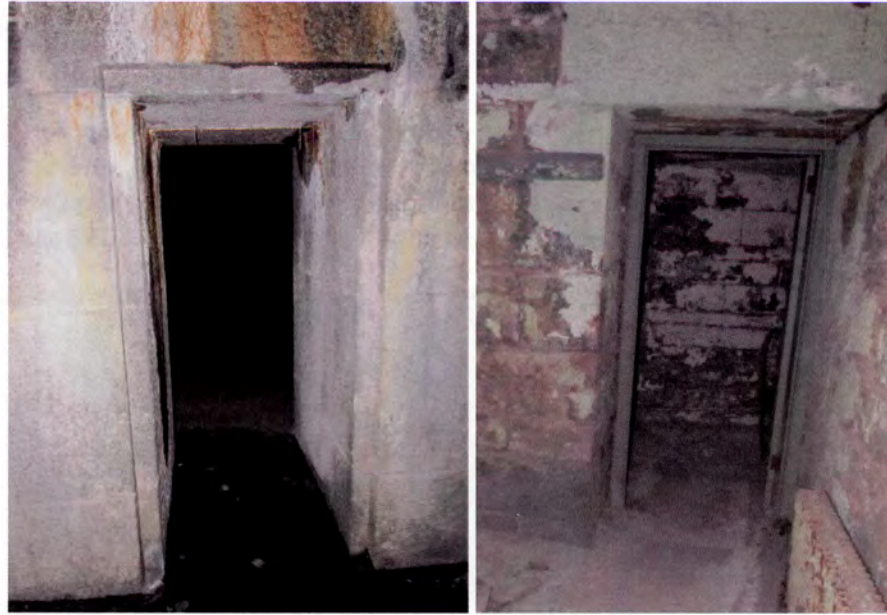
Figure 91: Typical doors in corner sections showing water damage (left).
