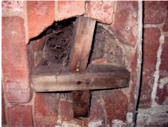
Figure 55: Hole in arched opening.
