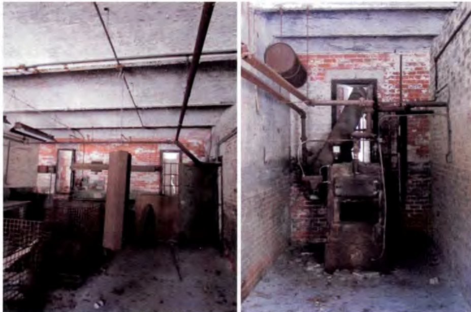
Figure 47: Deteriorating electrical and mechanical systems of first floor.
