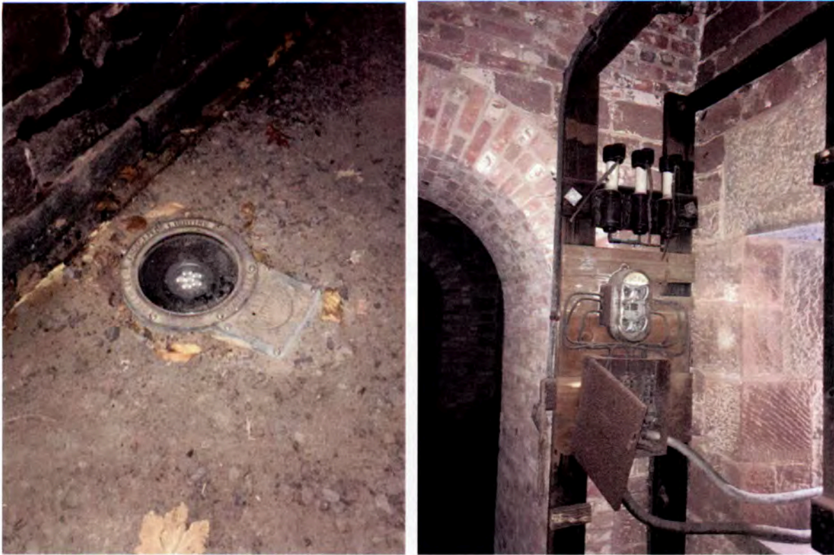
Figure 98: Modern floor light fixture (left) and badly deteriorated electrical equipment (right).
