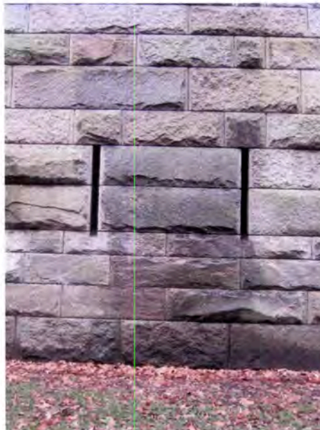
Figure 21: Water damage near ground level of the west elevation.
