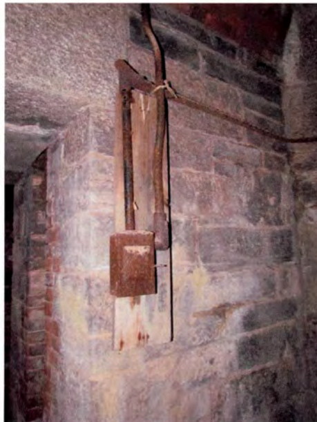
Figure 85: Electrical equipment in corner section of second floor.
