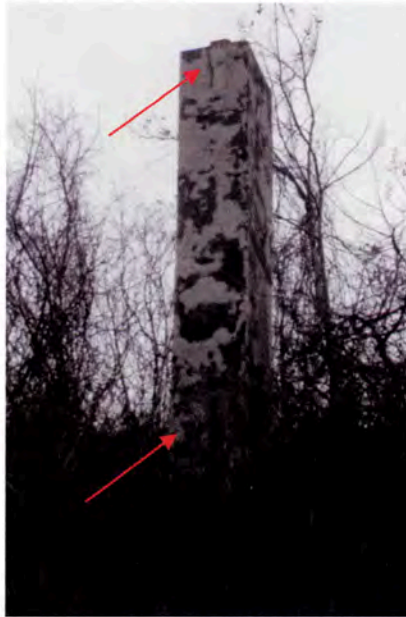
Figure 12: Small crack at the top of the east chimney and an area of patching at the bottom.
