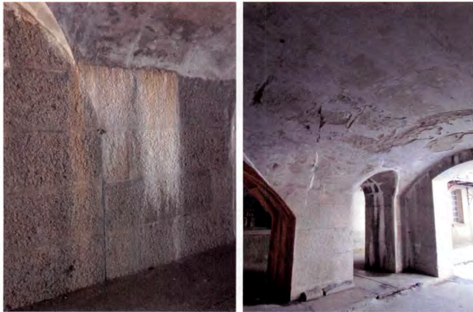
Figure 59: Efflorescence on wall of north sally port (left) and spalling concrete ceiling in south sally port (right).
