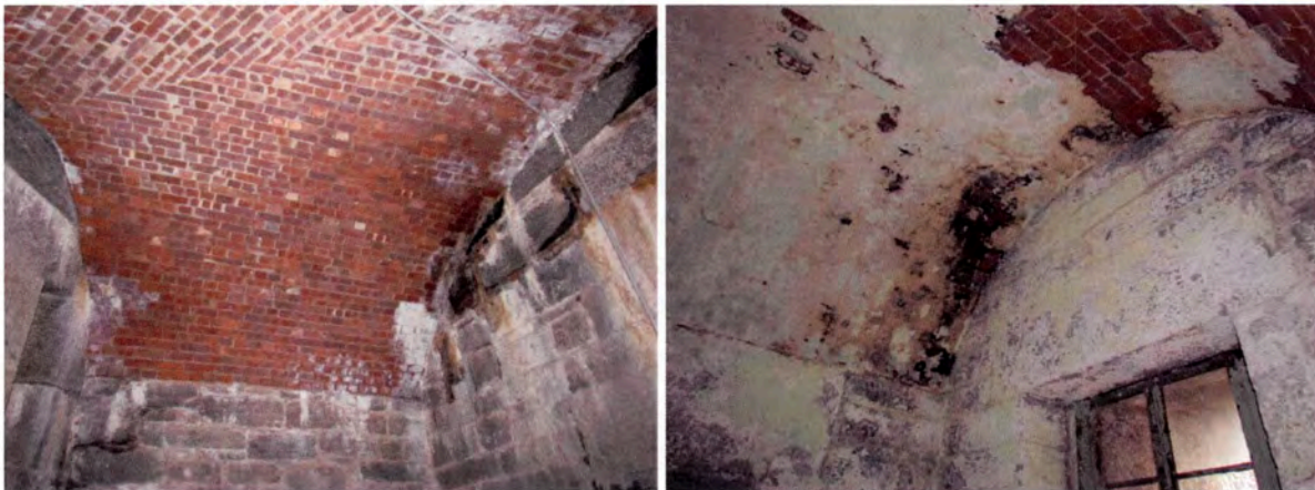
Figure 89: Typical brick ceilings in corners with evidence of water damage.
