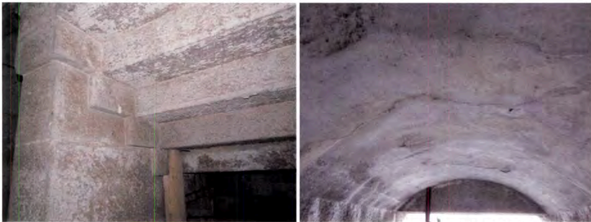
Figure 71: Wood post in north stair (left) and crack in roof structure on south stair (right).
