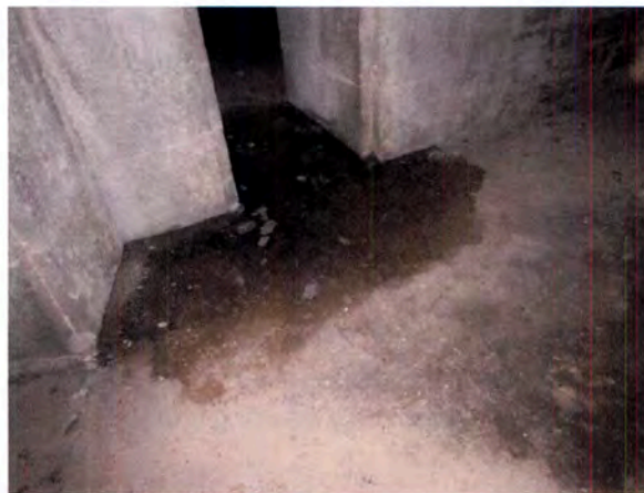
Figure 87: Water damage on concrete floor in corner section.
