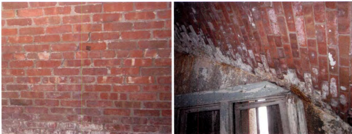
Figure 70: Crack in masonry barrel arch (left) and water intrusion on east wall (right).
