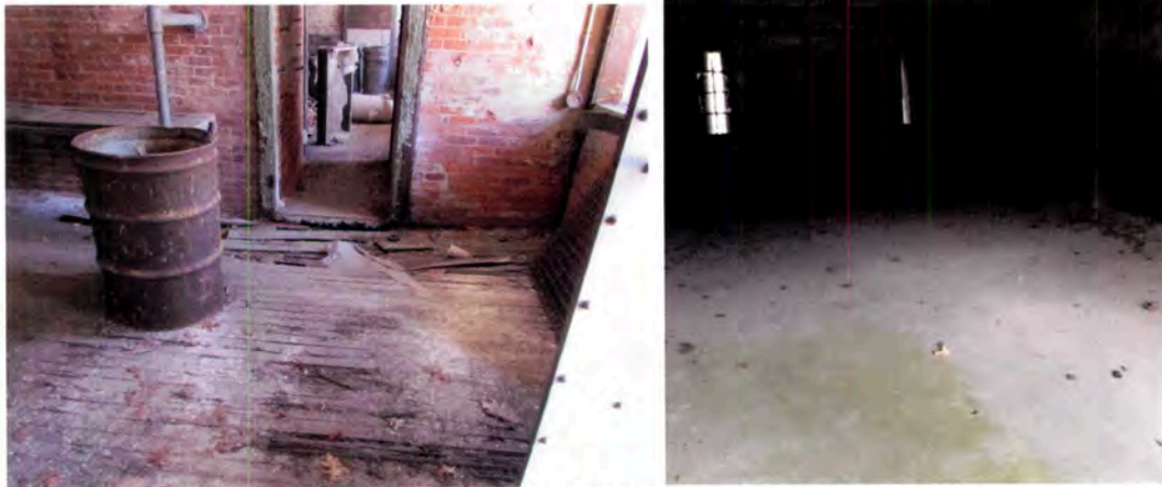
Figure 40: Deteriorating wood floors (left) and concrete floor (right) on first floor.
