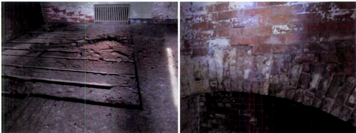
Figure 81: Deteriorated floor (left) and crack above fire place (right).
