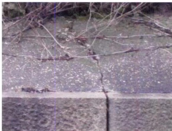
Figure 19: Crack in concrete below level of vegetation.
