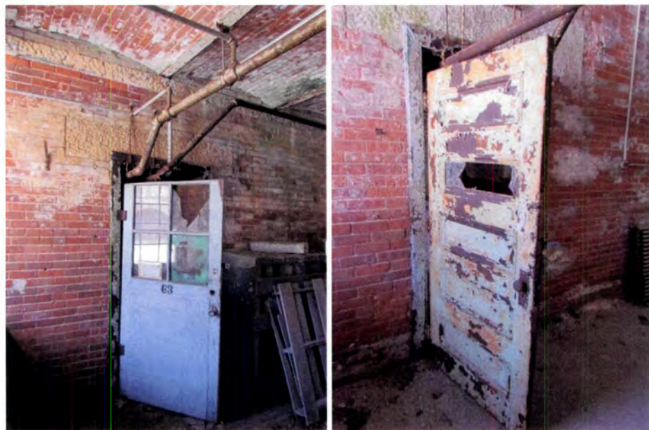
Figure 46: Modified wood-paneled door (left) and deteriorating five-paneled metal door (right).
