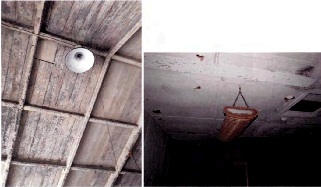
Figure 75: Typical ceiling mounted light (left) and typical suspended fluorescent fixture (right) on the second floor.
