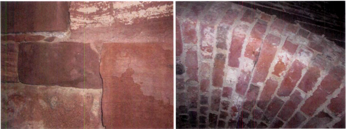
Figure 100: Eroded sandstone (left) and crack in brick arch (right).
