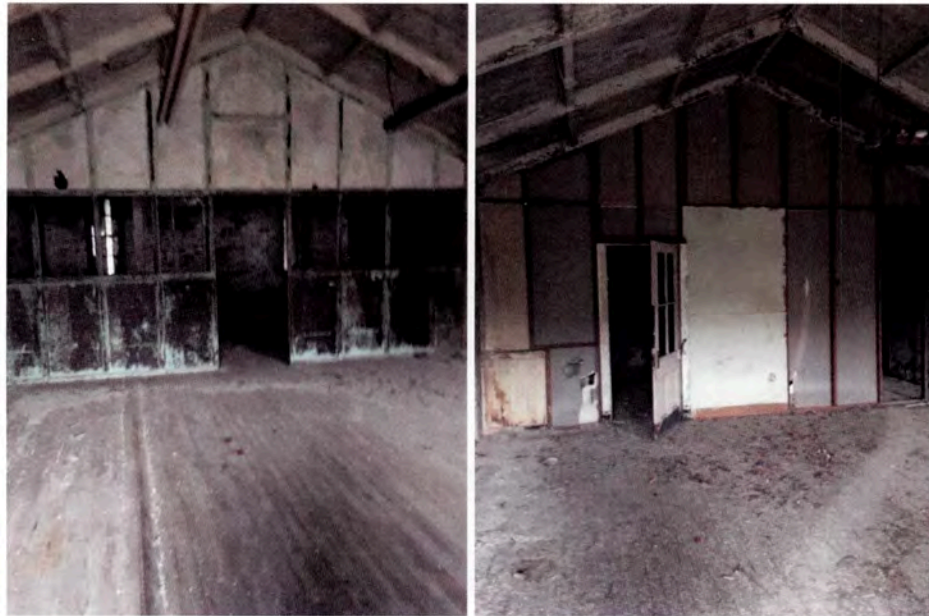
Figure 75: Deteriorating plasterboard partitions.
