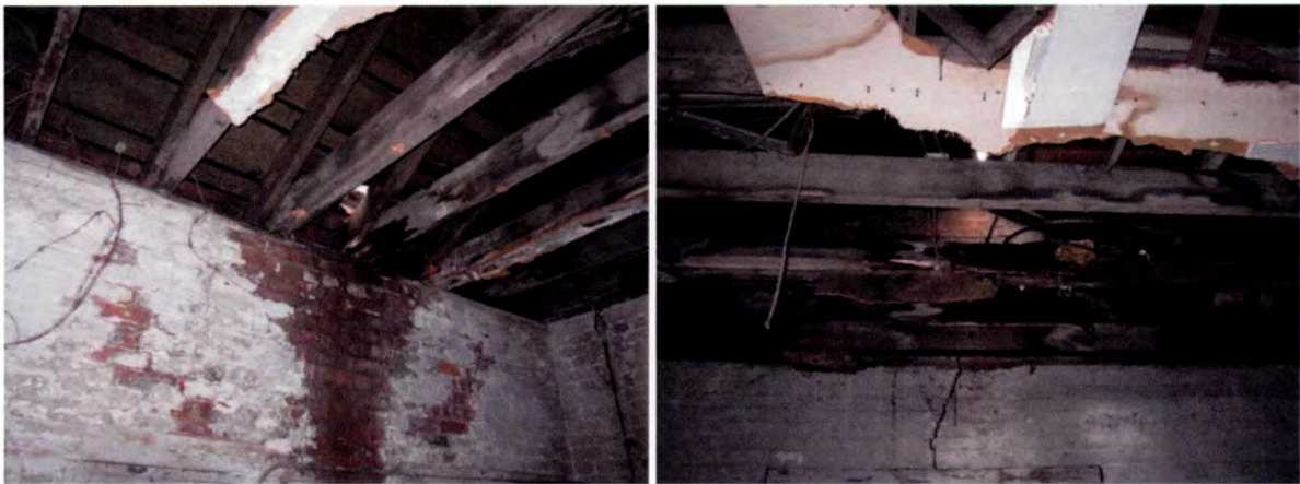
Figure 112: Deteriorating wood trusses in Building 139.
