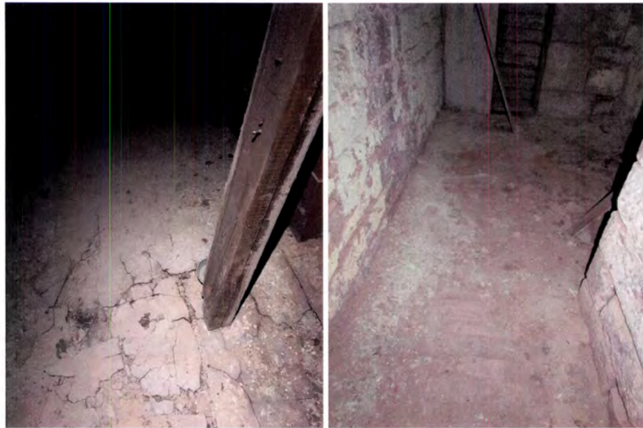
Figure 86: Deteriorated composite sheet flooring (left) and brick floors obscured by debris (right).
