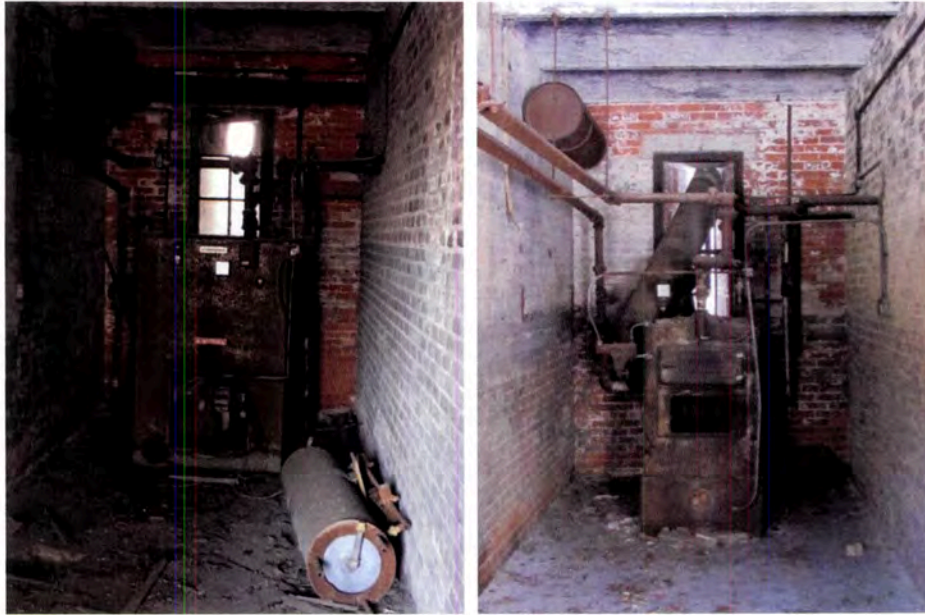
Figure 39: Boilers in Rooms 119 and 143.
