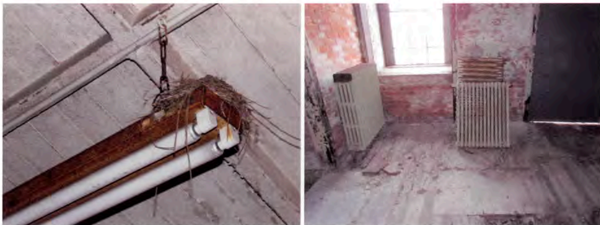
Figure 80: Rusty suspended fluorescent light fixture with bird nest (left) and typical conditions of radiators (right).
