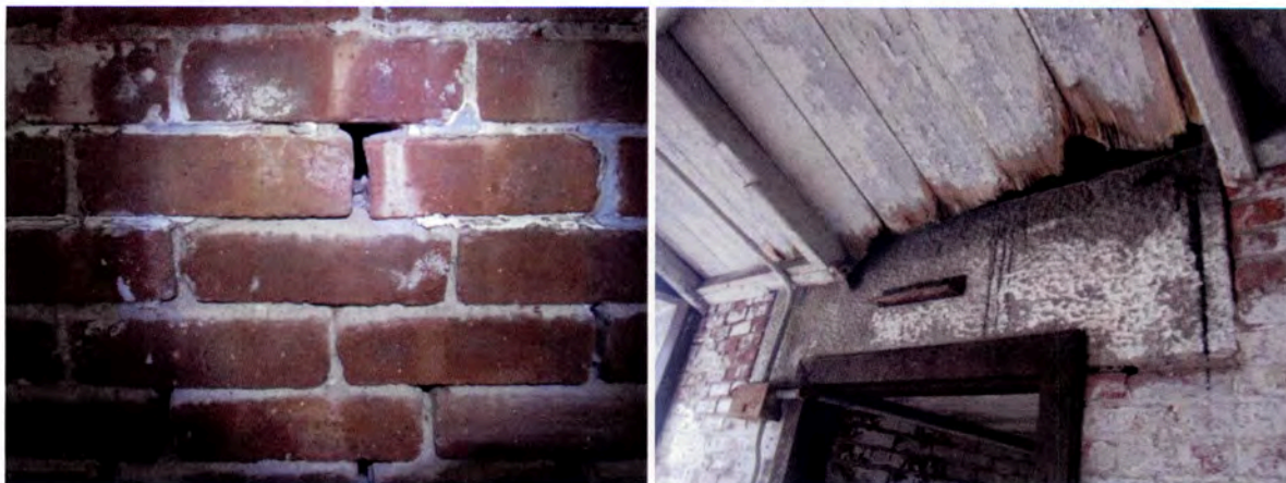
Figure 83: Missing mortar in bowing wall (left) and failed roof purlin bearing (right).
