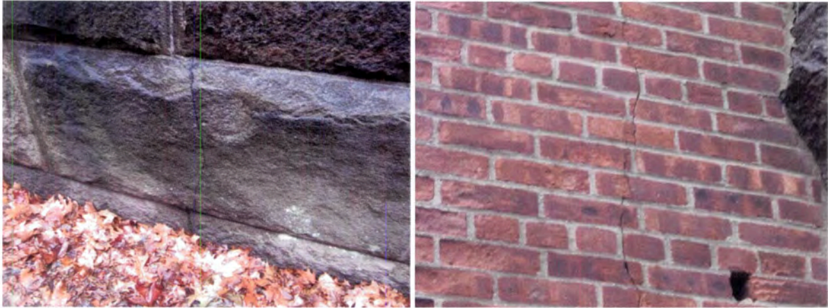
Figure 18: Crack at base of wall on north elevation (left) and crack in chimney on west elevation (right).
