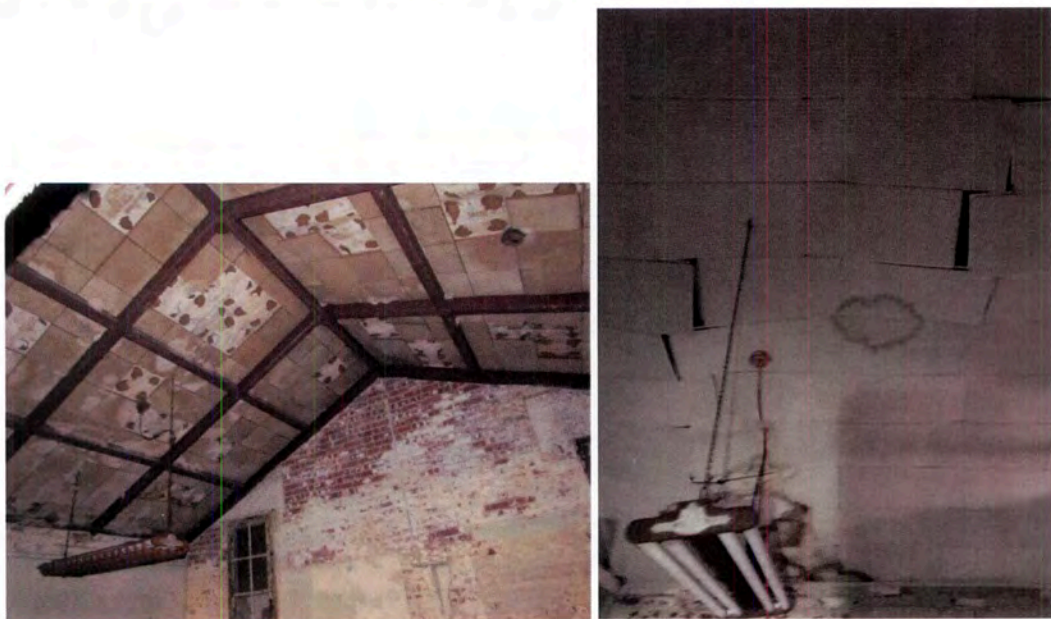
Figure 77: Deteriorating ceiling tiles.
