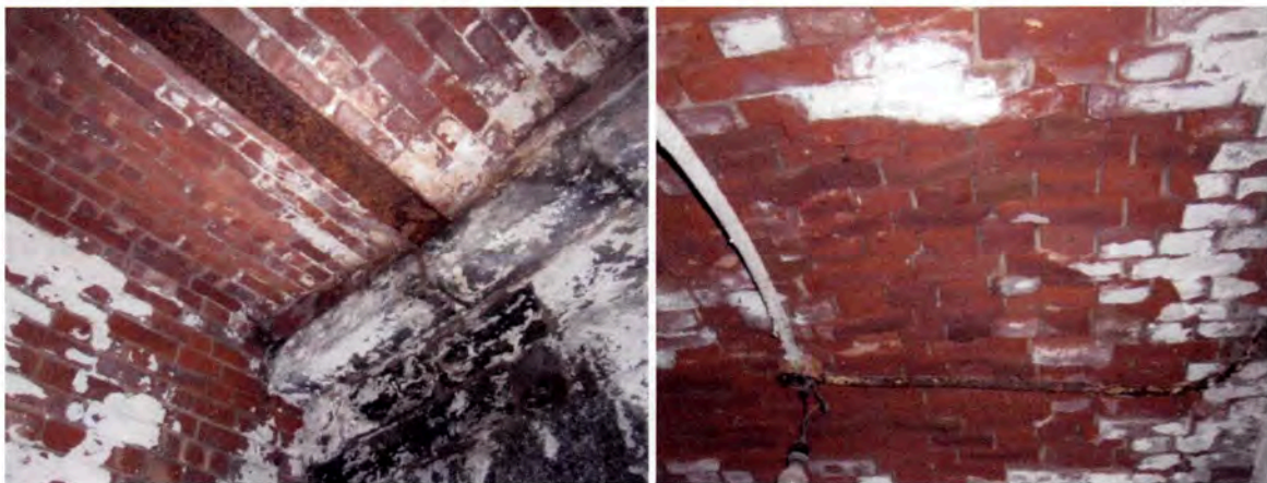
Figure 57: Rusted beam at entrance to Room 111 (left) and brick loss in Room 124 (right).
