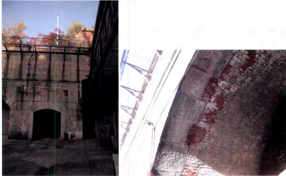
Figure 28: Southeast corner of Parade showing staining and efflorescence on east elevation (left) and crack in masonry arch on east elevation.
