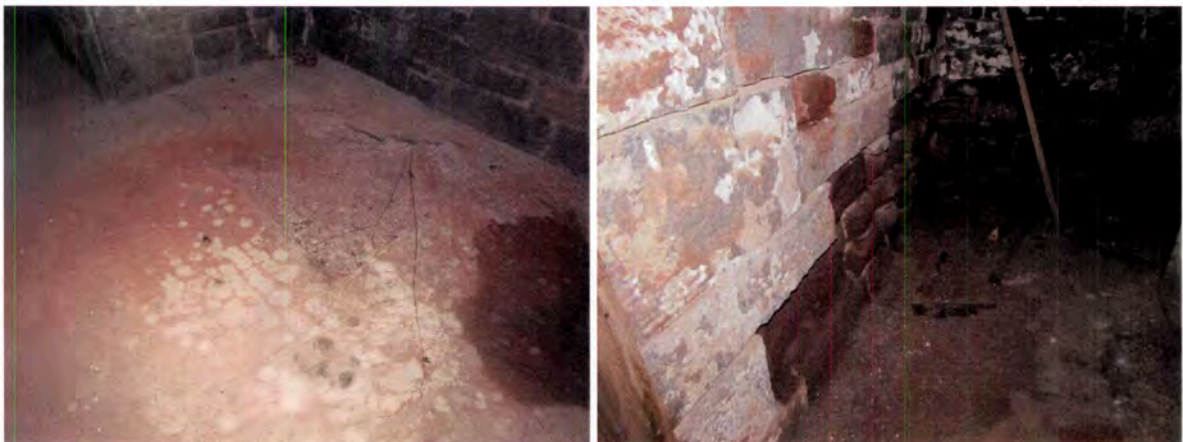
Figure 52: Typical floor conditions of corner sections with water damage and vegetation.
