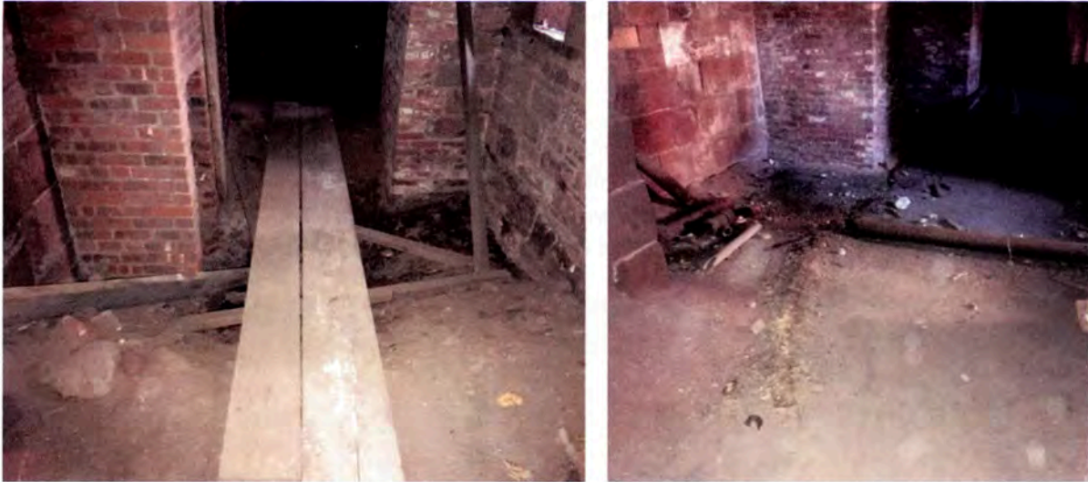
Figure 95: Wood planks traversing the depression in the floor at C146 (left) and exposed pivot rails (right).
