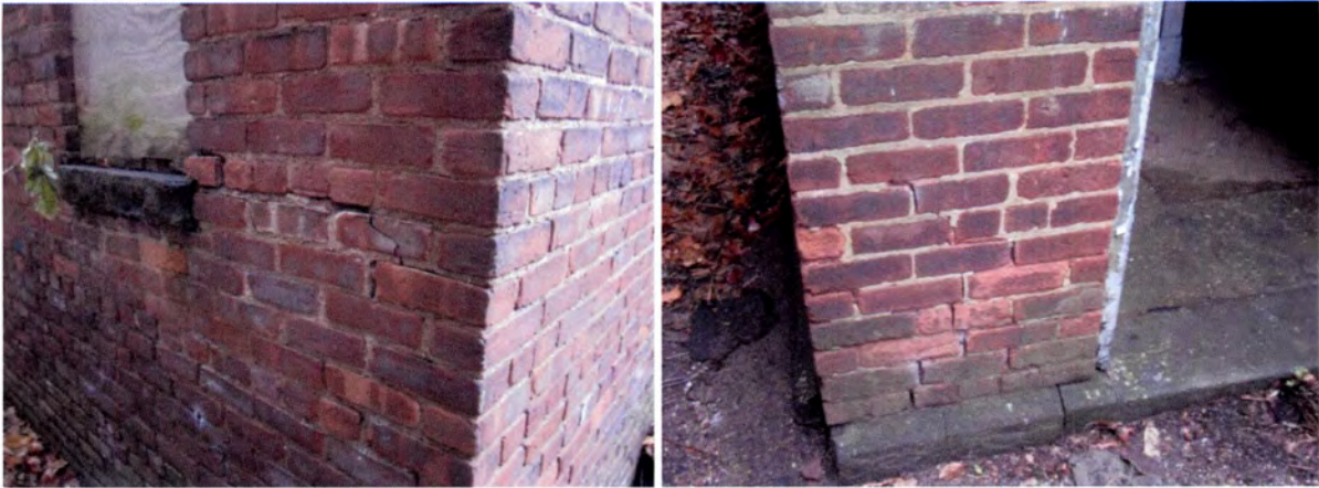
Figure 111: Cracks in masonry in northeast corner (left) and northwest corner (right) of Building 139.
