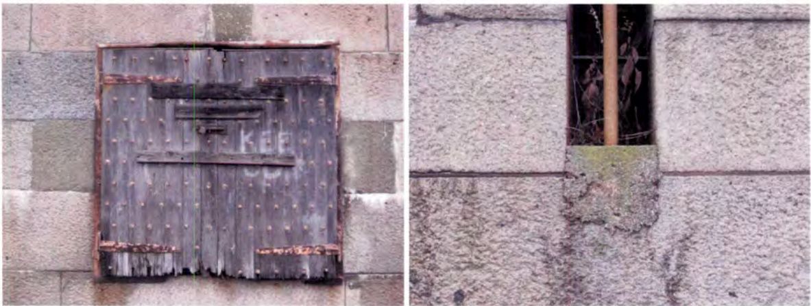
Figure 8: The masonry opening and wood panel on the east elevation is in poor condition (left). Many embrasures have been modified with concrete at the bottom to accommodate the metal bar.
