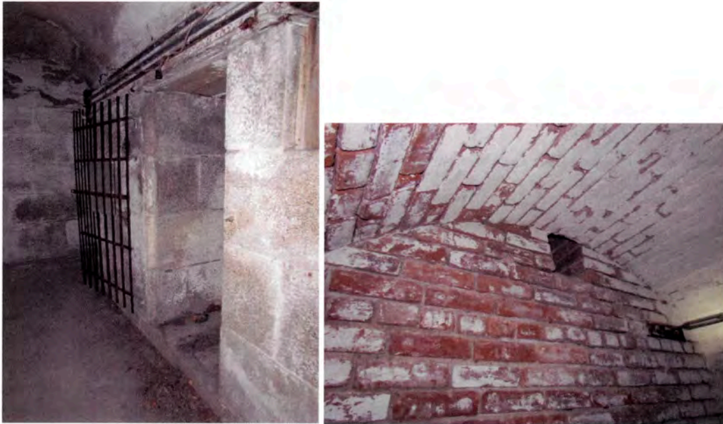
Figure 94: Rusted security door (left) and missing pointing in brick ceiling and walls (right).
