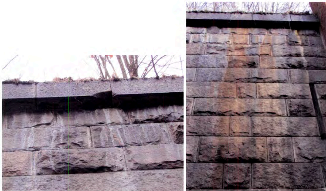
Figure 1: Piece of broken granite coping and water stains (left) and severe rust stains (right) on south section of west elevation.
