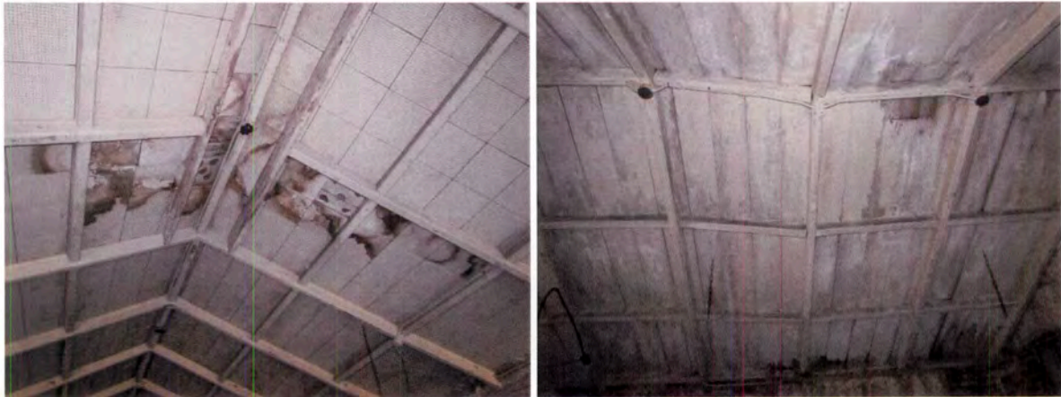
Figure 76: Water damage in acoustical ceiling tile (left) and sagging bead board and exposed wood rafters (right).
