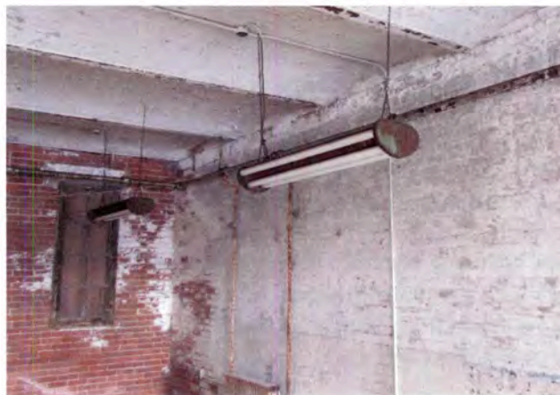
Figure 36: Typical suspended fluorescent lights.
