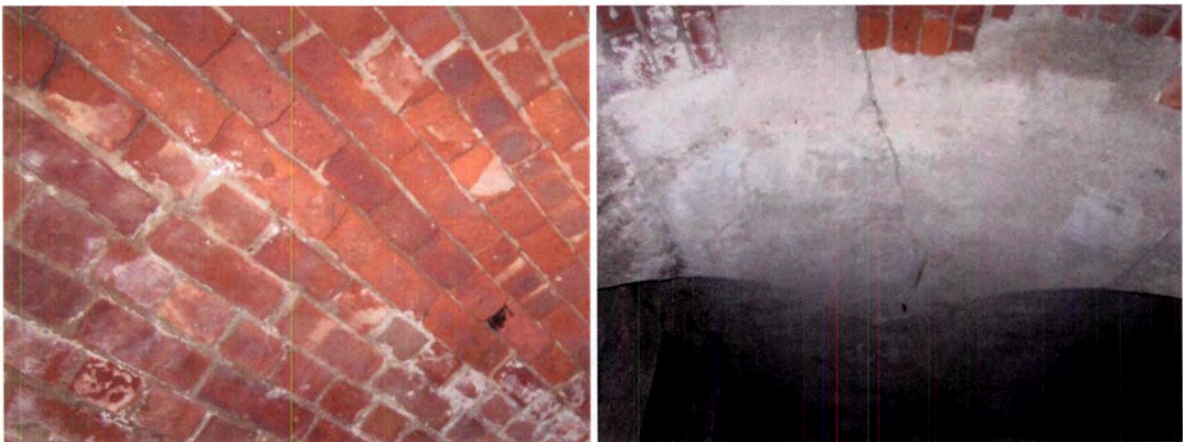
Figure 101: Erosion to brick / mortar (left) and crack in barrel (right).
