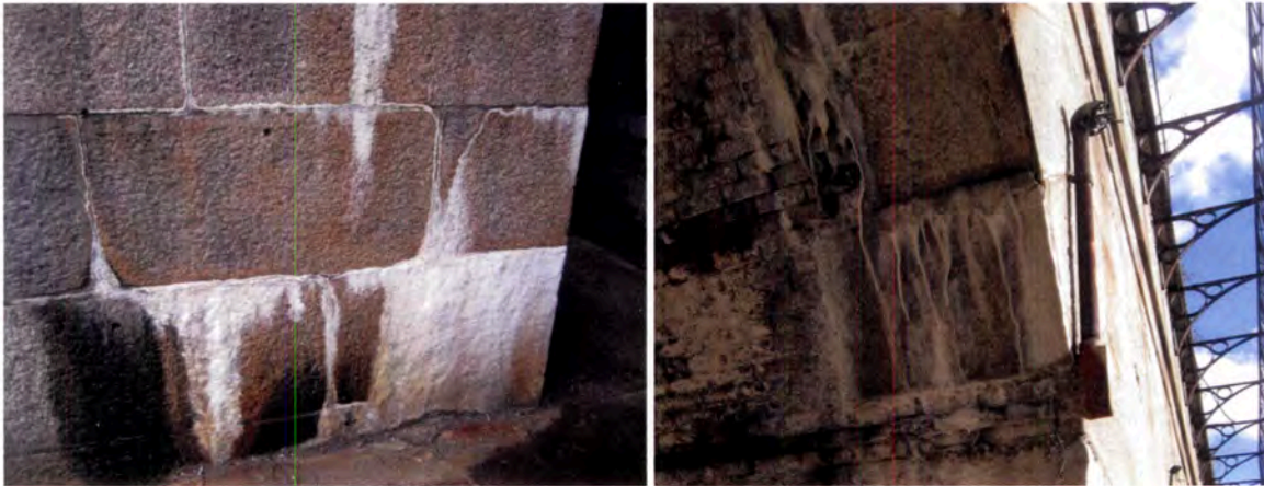
Figure 31: Efflorescence on wall (left) and on stone and brick arch (right).
