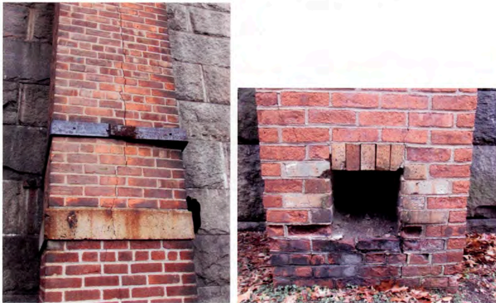
Figure 13: Cracks, spalling and missing bricks on chimneys.
