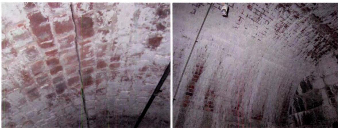
Figure 85: Crack in roof of Room 235 (left) and efflorescence in Room 233 (right).
