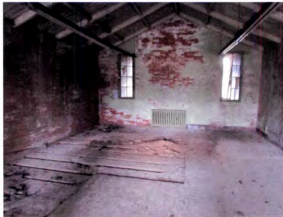
Figure 73: Deteriorating wood and plywood floor coverings on second floor.
