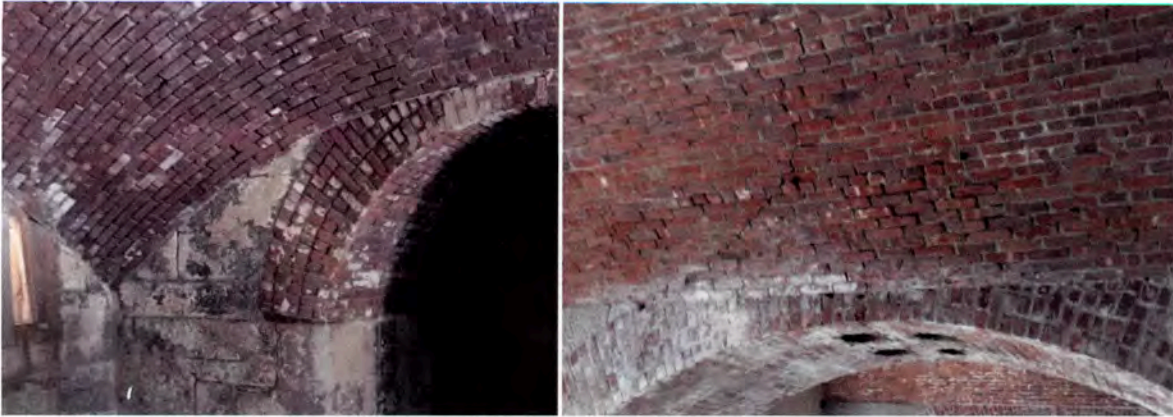
Figure 63: Brick and mortar deterioration at casemate ceilings.
