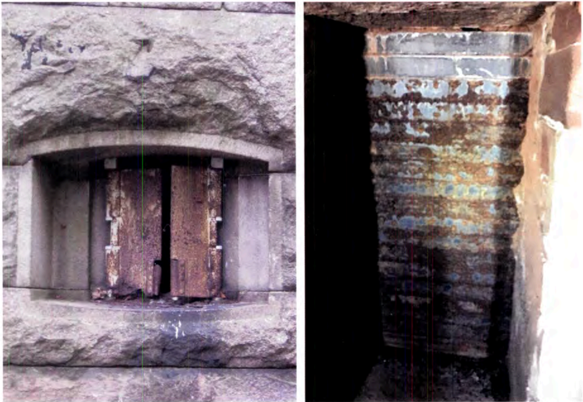
Figure 97: Badly deteriorated embrasure shutters (left) and significant rust and door blocked with steel (right).
