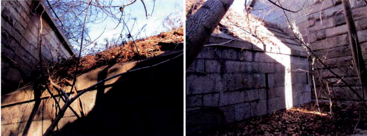
Figure 6: Vegetation on roof (left) and minor stains on small section between counterscarp and fort.
