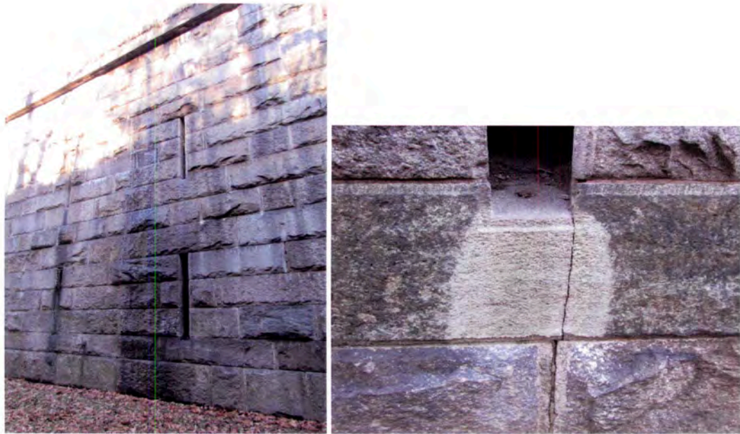
Figure 4: Active water (left) and minor crack under masonry opening (right) on the north section of the west elevation.
