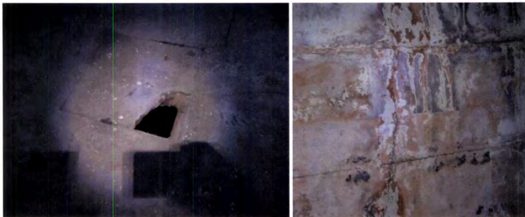
Figure 69: Hole in floor in Casemate N (left) and crack in east wall of M (right).
