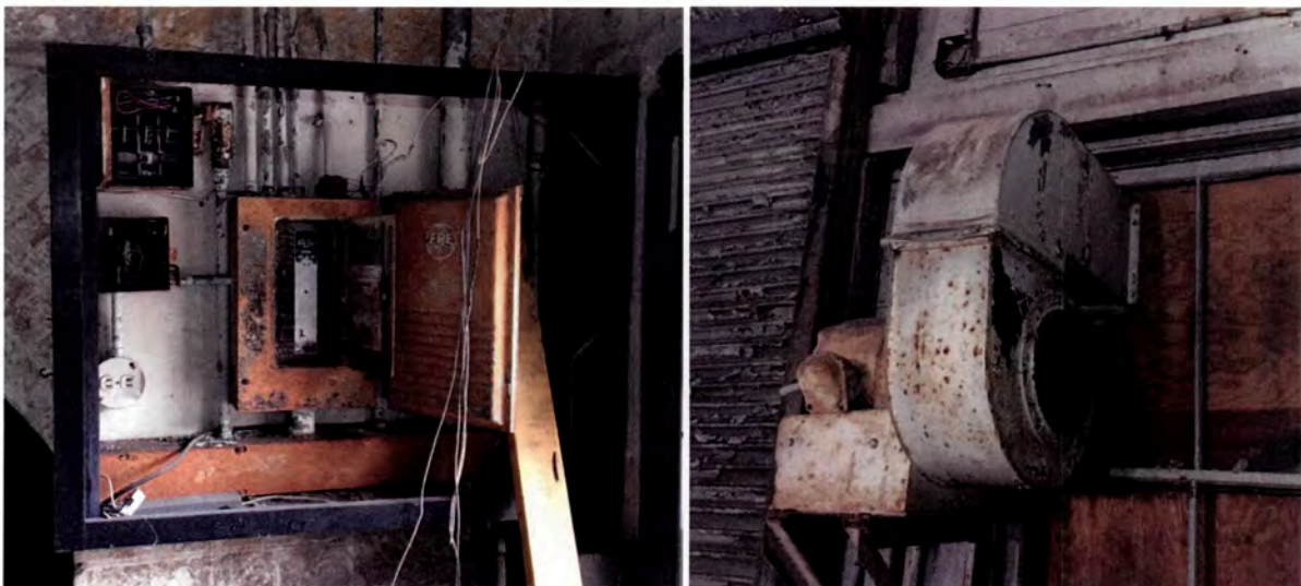
Figure 68: Damaged electrical panels (left) and rusted exhaust fan (right).
