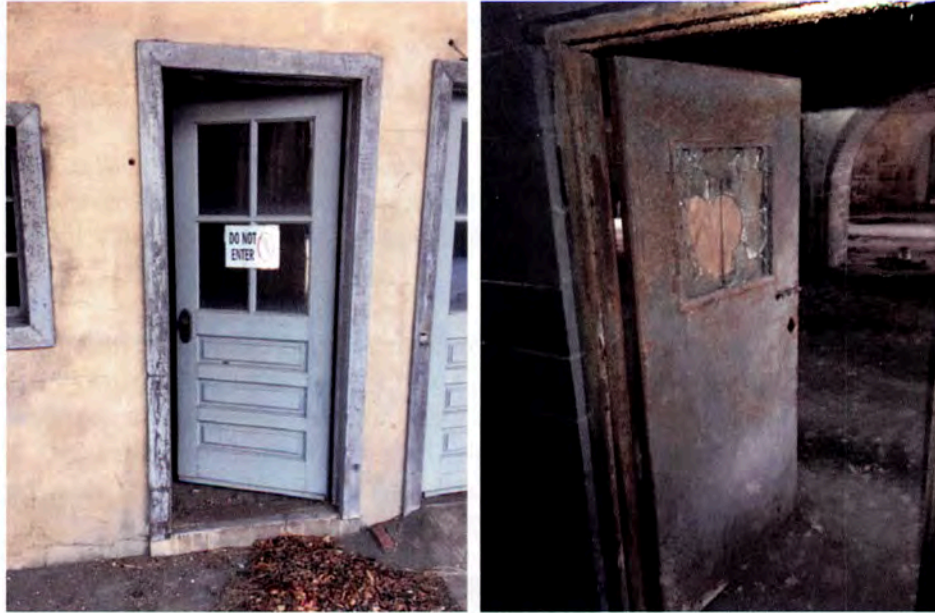
Figure 67: Modern wood replacement door (left) and significant rust and damage at hollow metal door (right).
