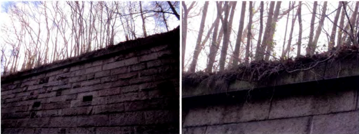
Figure 21: Large trees growing on counterscarp roof (left) and detail of coping and vegetation (right).
