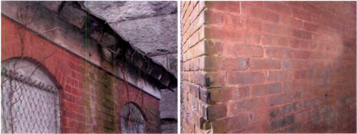
Figure 102: Stains on masonry below damaged roof and fascia (left) and stepped crack in masonry (right).
