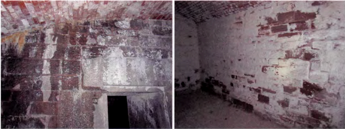
Figure 53: Deteriorating wall conditions of the corners including water damage (left) and fading whitewash (right).
