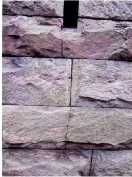
Figure 22: Crack in granite wall below masonry opening on west elevation.
