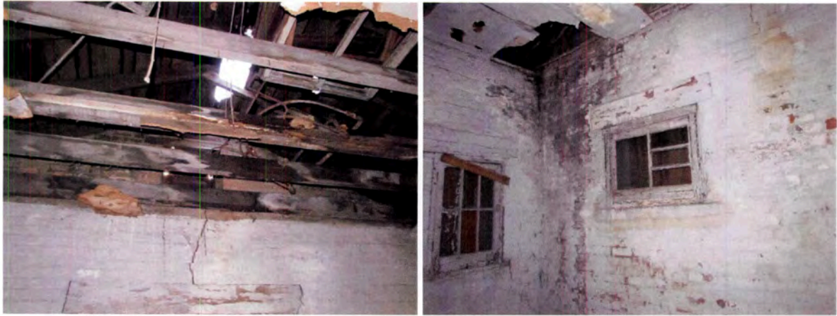
Figure 109: Hole in roof and deteriorating wood rafters (left) and overview of the interior of Building 139.
