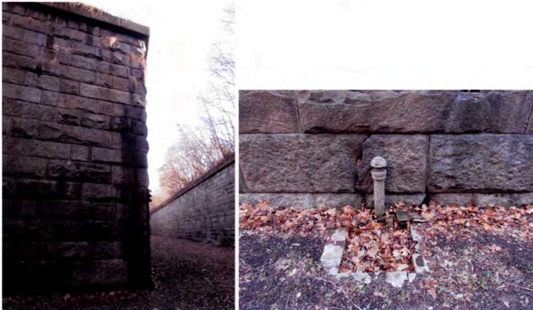
Figure 7: Active water on west end of north elevation (left) and minor crack in masonry (right).
