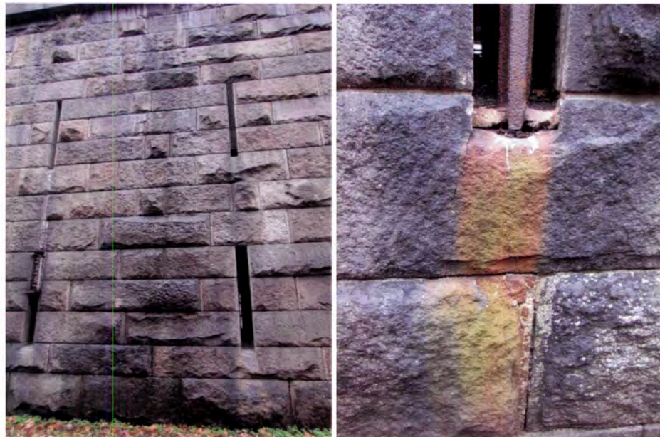
Figure 5: Active water (left) and rust stain from bar in masonry opening (right) on south section of west elevation.
