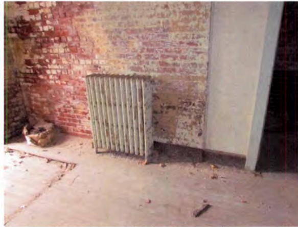
Figure 77: Typical radiator on second floor.
