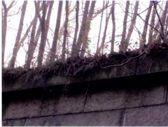
Figure 25: Vegetative roof and biological staining on coping of counterscarp.
