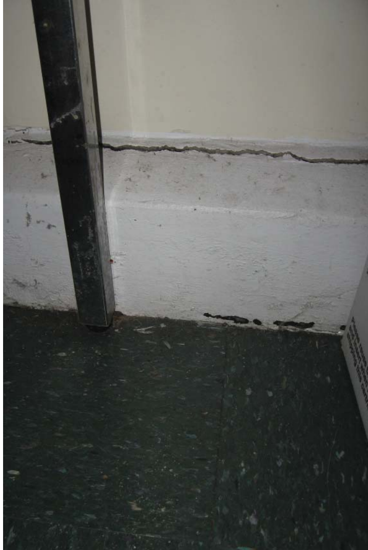
Photo 77. Detail of the masonry curb at the northeast corner of the historic kitchen area. Note the gap between the wall and the curb. (JMA, October 2009)
