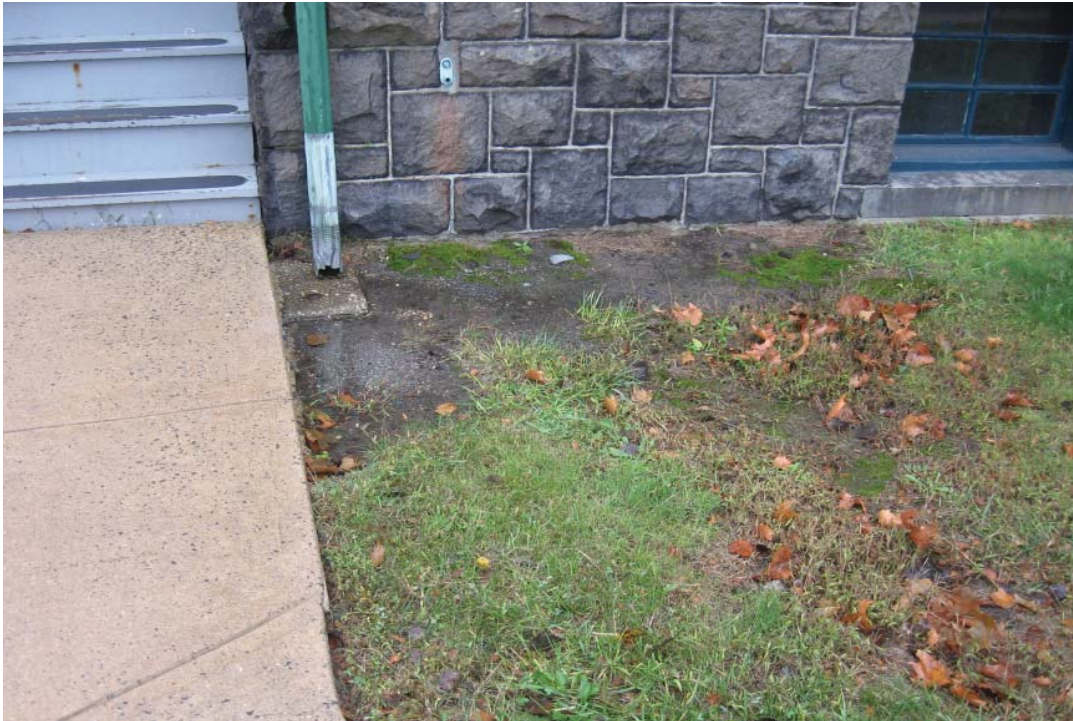
Photo 55. Detail of site drainage at the northeast corner. Note the eroded soil and moss growth that indicates poor site drainage. (JMA, October 2009)
