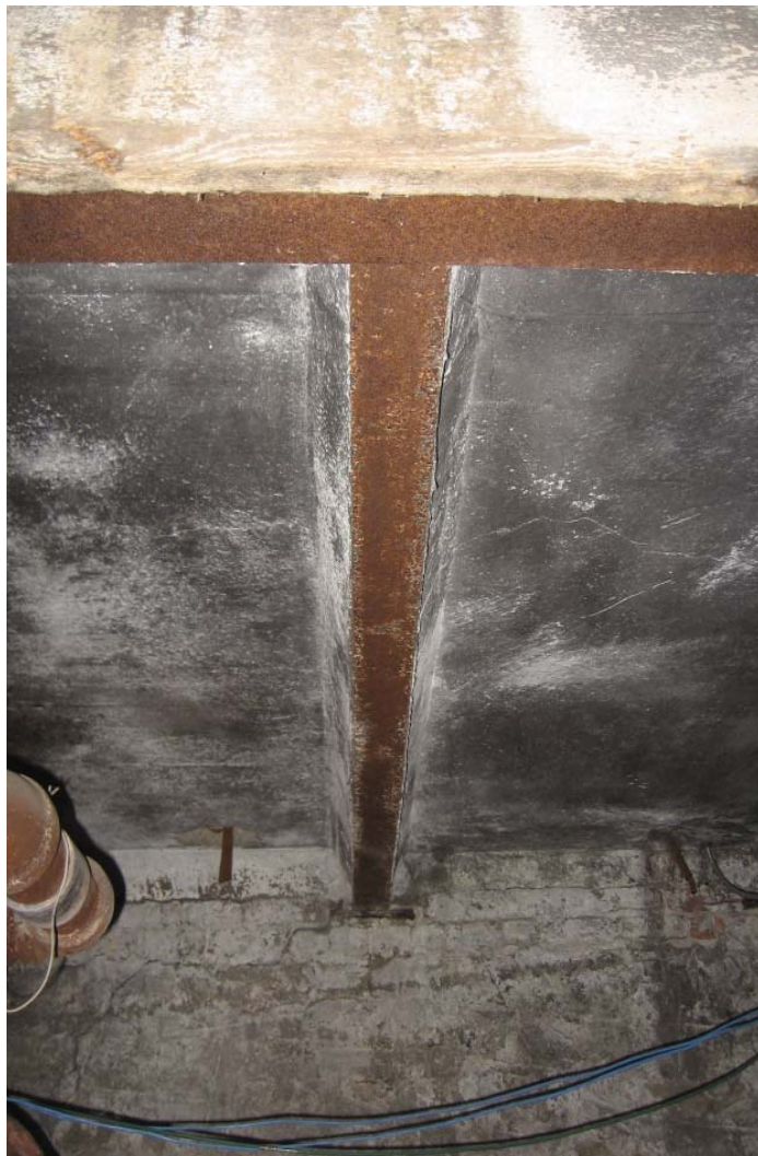
Photo 82. Detail of the steel framing and cement parged panels at the north end of the Boiler Room. Note the corrosion of the steel beams. (JMA, October 2009)
