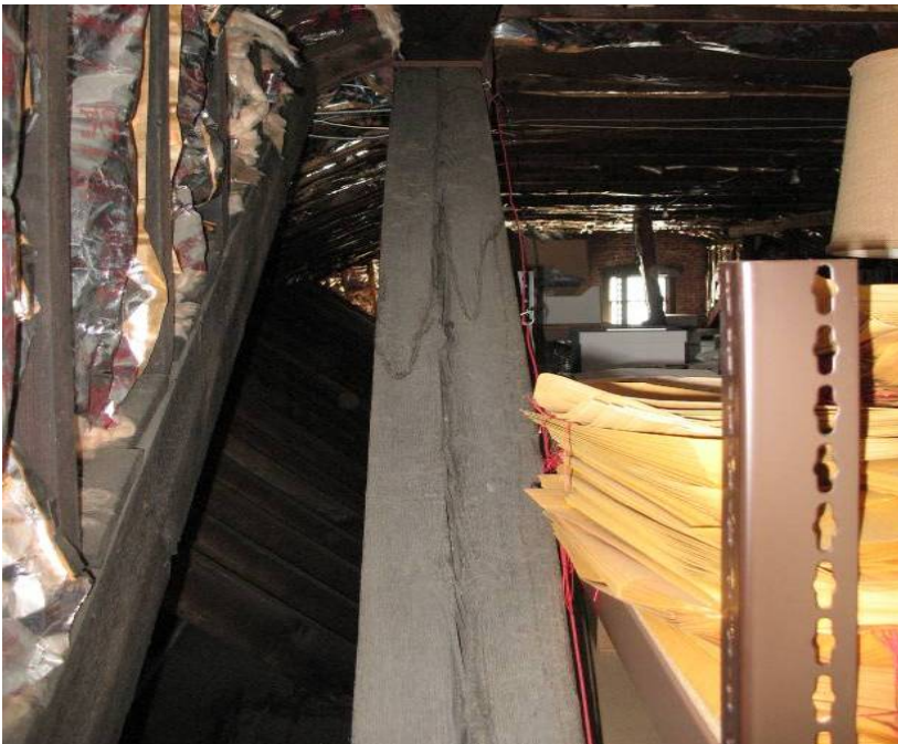
Photo 6: Check in sloping timber top chord of east truss – north end.
