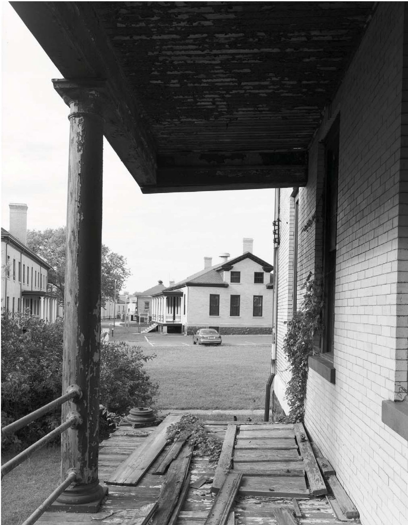
Photo B-12. Building #58, looking north from deteriorated porch of Mess Hall Building #57. Fort Hancock, Sandy Hook Unit, Gateway National Recreation Area. Sandy Hook, New Jersey. Photographer: Doug Harnsberger. September 2010.
