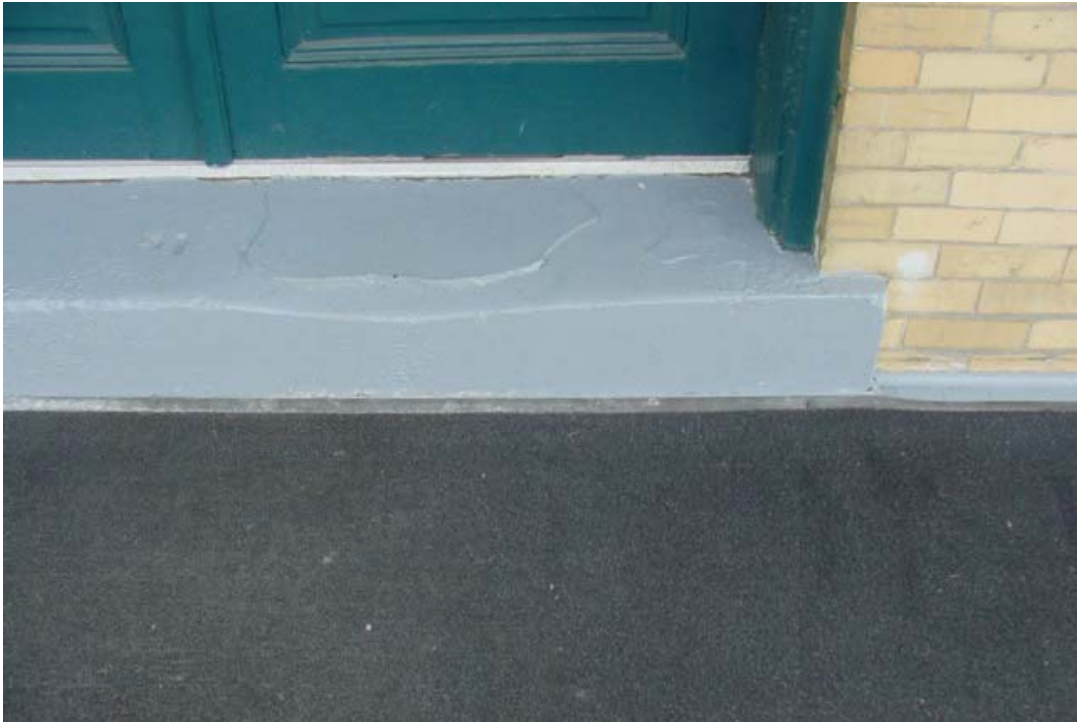
Photo 62. Detail of the main west entrance door sill. Note the cement patch at center and recent gray paint. (JMA, August 2010)
