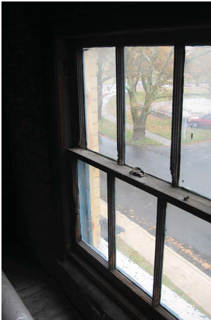
Photo 67. Interior detail of the northwest attic window (201D). Note the damage at the interior muntins. (JMA, October 2009)
