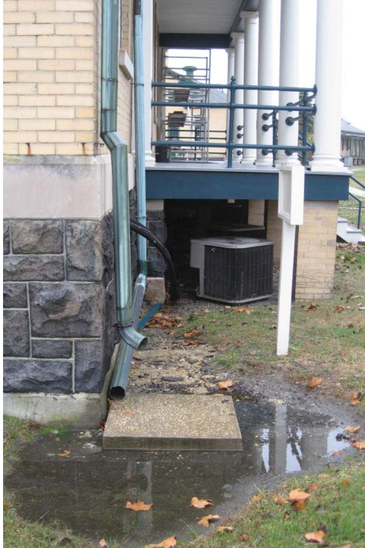
Photo 56. Condition of site drainage at the northwest corner. Note the discharge of two downspouts and ponding water. (JMA, October 2009)
