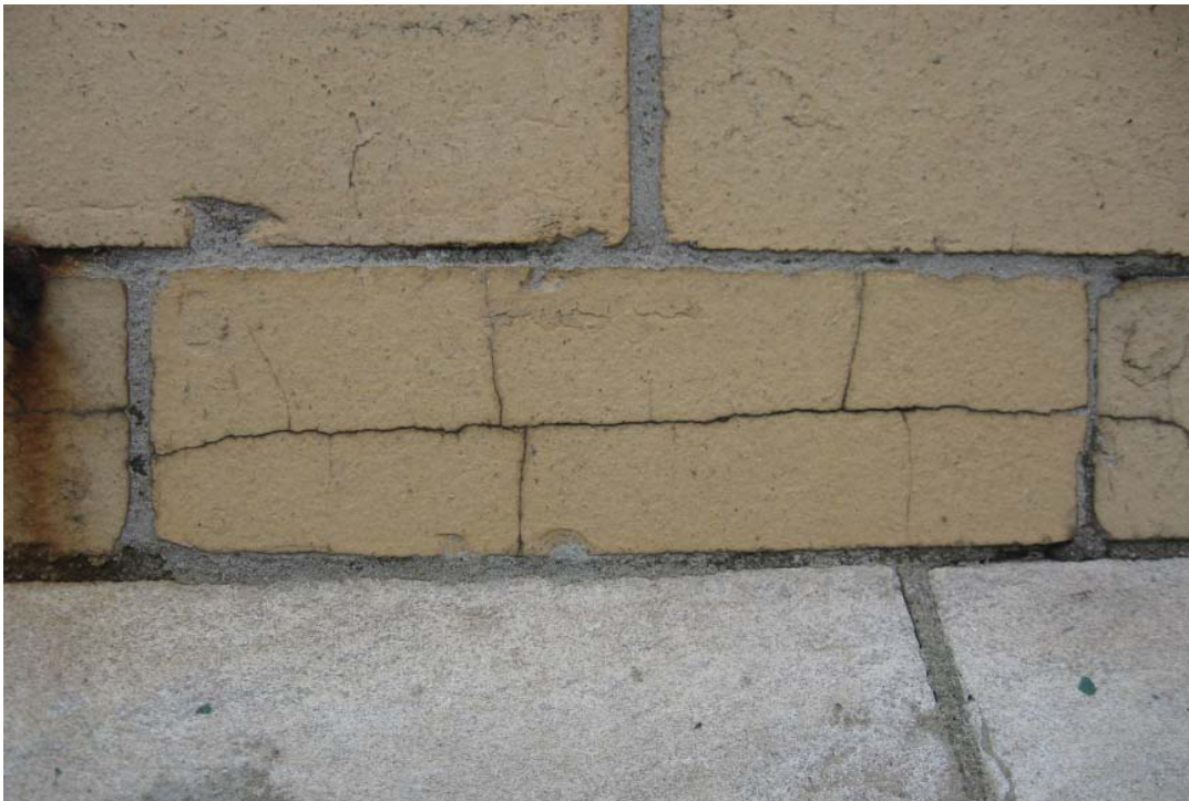
Photo 60. Detail of typical cracked brick unit with a crack through the long axis of the face and smaller cracks radiating up and down. (JMA, October 2009)
