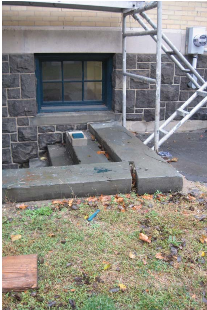
Photo 66. West basement entry stair. Note the gap between the slate curb and the rectangular slot where a cramp once held the stones together. (JMA, October 2009)
