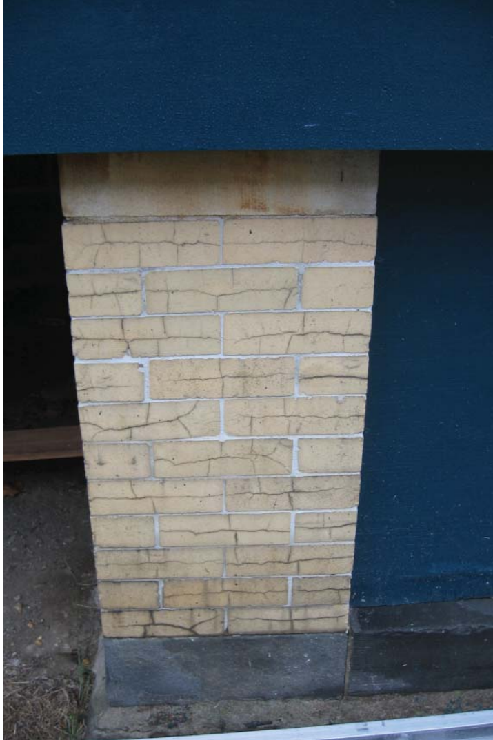
Photo 59. Detail of hairline cracks at the brick masonry at the west porch piers. The cracking is typical of almost all brick units regardless of location. (JMA, October 2009)
