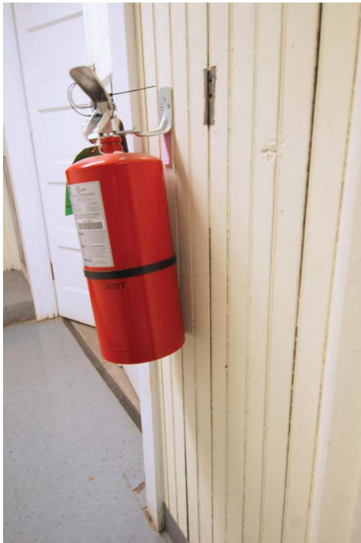
Photo 96. Typical hand held dry chemical fire extinguisher shown here at the basement level (JMA, October 2009).
