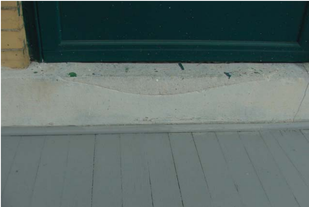
Photo 63. Detail of the door sill at the southern entry at the west façade. Note the large concrete patch and evidence of a past gray coating. (JMA, August 2010)
