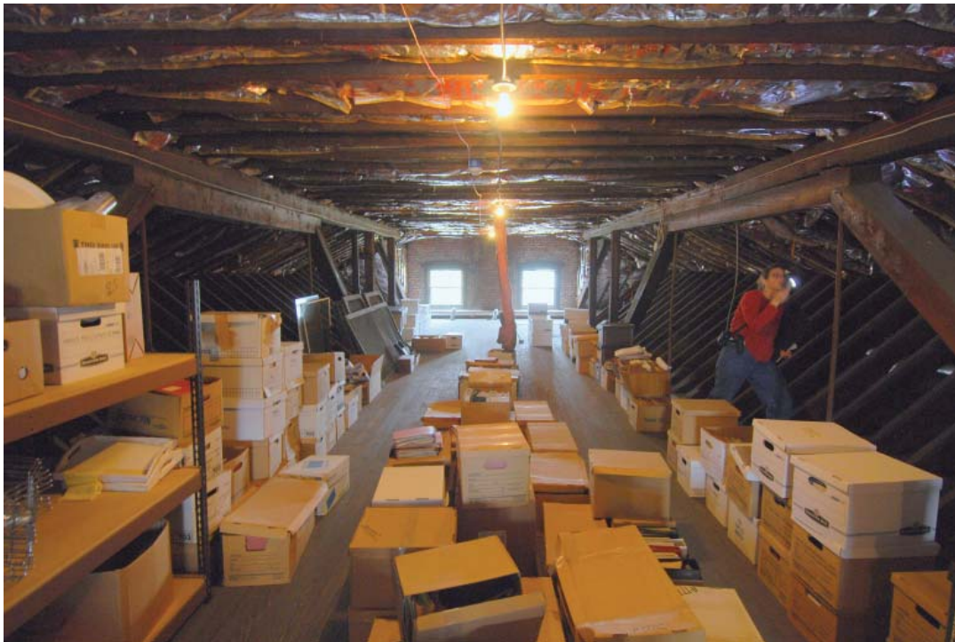
Photo 97. Overview of the attic looking north. The debris and miscellaneous items in the attic are a fire hazard (JMA, October 2009).
