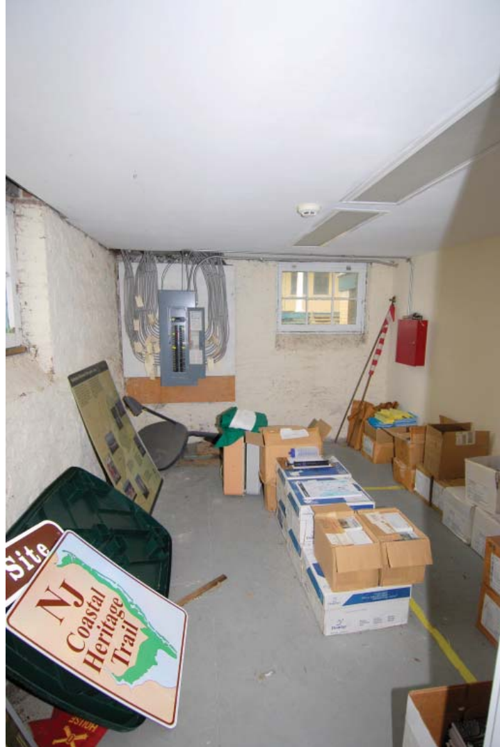
Photo 99. Overview of the electrical room looking west. The debris and miscellaneous items in the Electrical Room are a fire hazard (JMA, October 2009).
