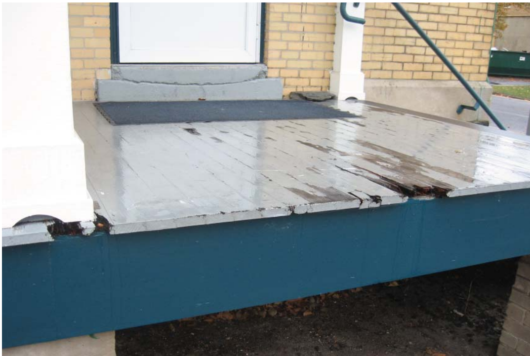
Photo 65. East porch floor. Note the deterioration at the exposed ends of the floor boards. (JMA, October 2009)
