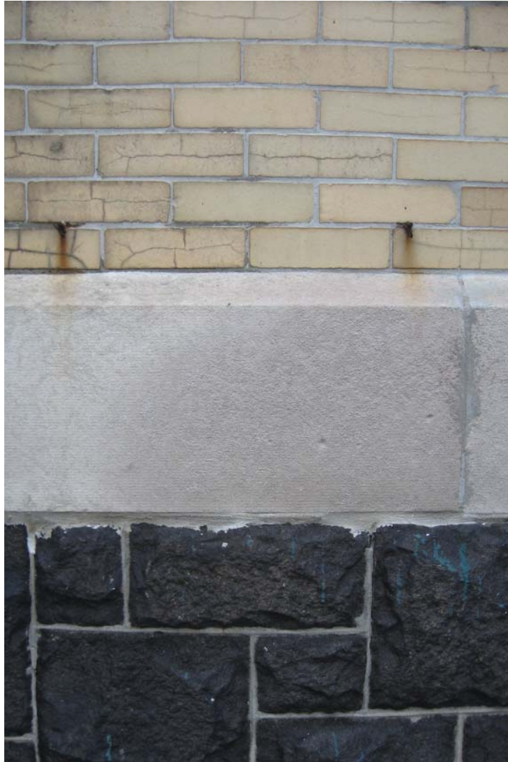
Photo 58. Detail of the masonry at Building #58. Buff colored brick at the top with characteristic hairline cracks. Light limestone trim at center. Dark diabase ashlar masonry at the foundation. (JMA, October 2009)
