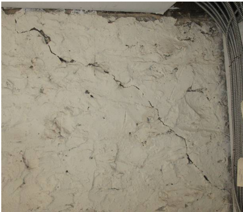
Photo 2: Crack in south wall at west corner from inside.
