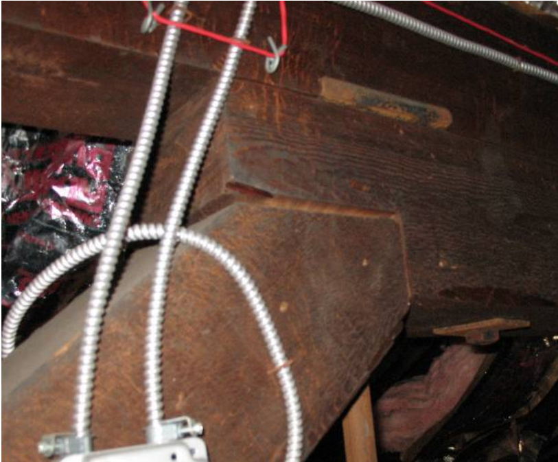
Photo 5: Truss diagonal to top chord connection. Notice gap in top chord caused by warping of the diagonal member.
