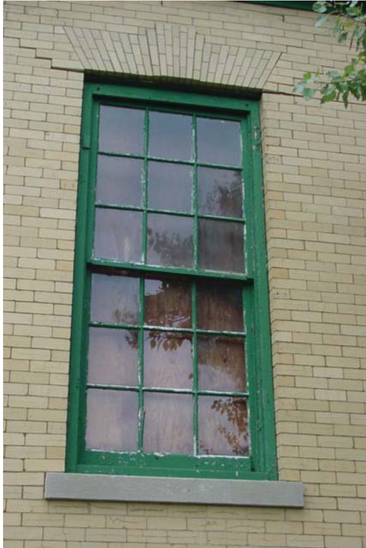
Photo 68. Original nine-over-nine window at Building #57 with a thinner casing and wider sash. Note the disruption of the masonry caused by the corroding lintel. (JMA, August 2010)
