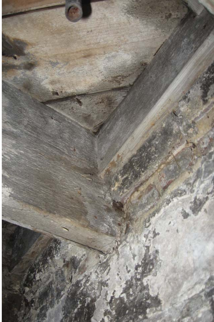
Photo 81. Detail of the floor joists supporting the northeast corner of the former kitchen floor. Note the damage where the wood sits in the masonry wall. (JMA, October 2009)
