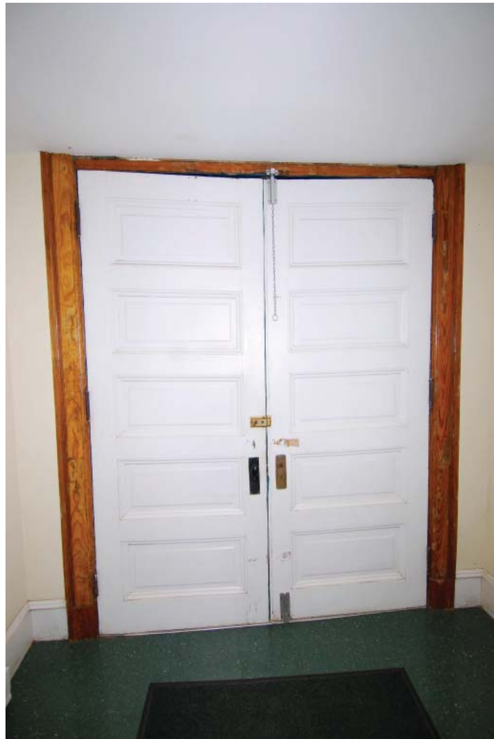
Photo 89. Existing historic double in swing doors with original hardware at main west entrance (114-2). In order to make these accessible, the doors will need to be activated by a push button mounted to the side (JMA, October 2009).
