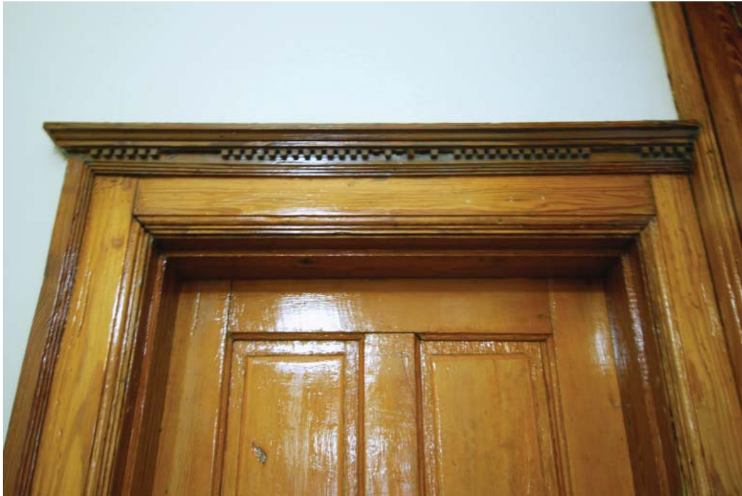
Photo 79. Detail of the wood trim at the door to Office 108. Note the missing dentils, the lack of paint, and the shiny polyurethane coating. (JMA, October 2009)
