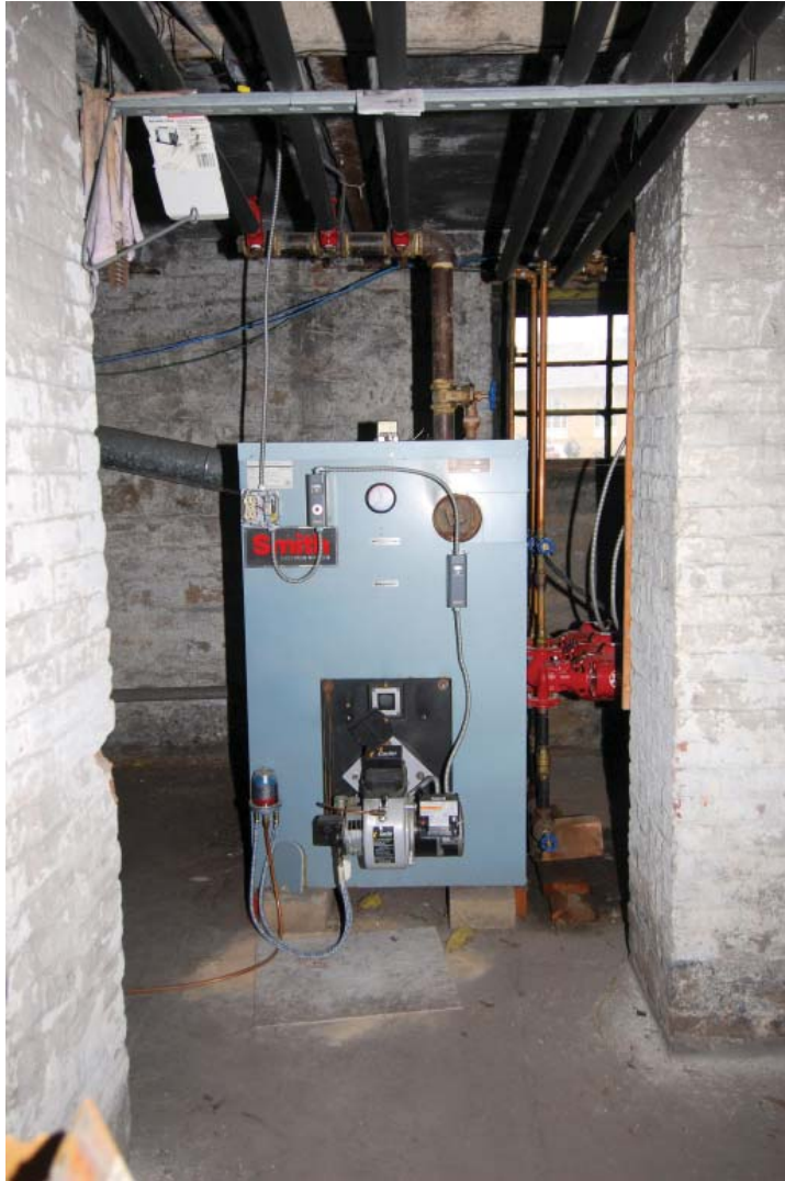
Photo 100. Detail of heating equipment in the boiler room. Heating equipment residing in the main portion of the boiler room should be enclosed by fire rated partitions as an additional safety precaution (JMA, October 2009).
