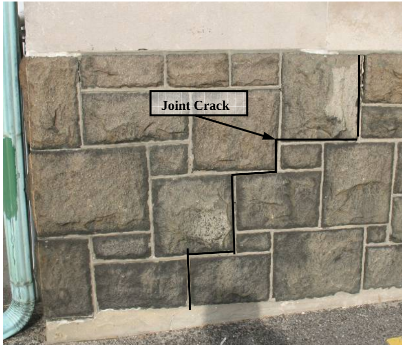
Photo 1: Crack in south wall at west corner. Crack extends through wall.
