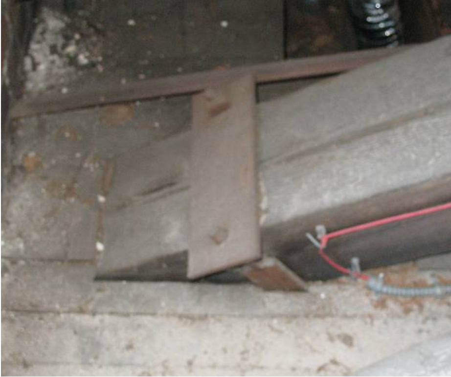
Photo 7: Strap at heel joint where top and bottom chords connect. Nut is missing from strap as noted in text above.
