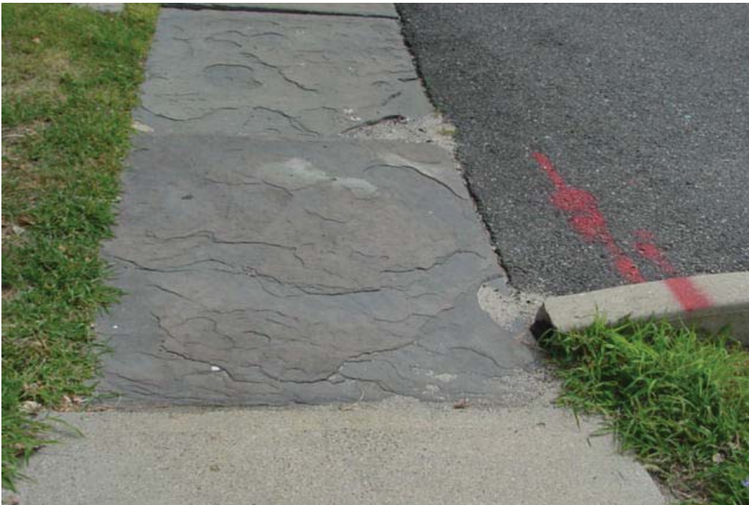
Photo 57. Detail of historic slate paving at southwest portion of the site. Note delamination and lipping between slabs. (JMA, August 2010)
