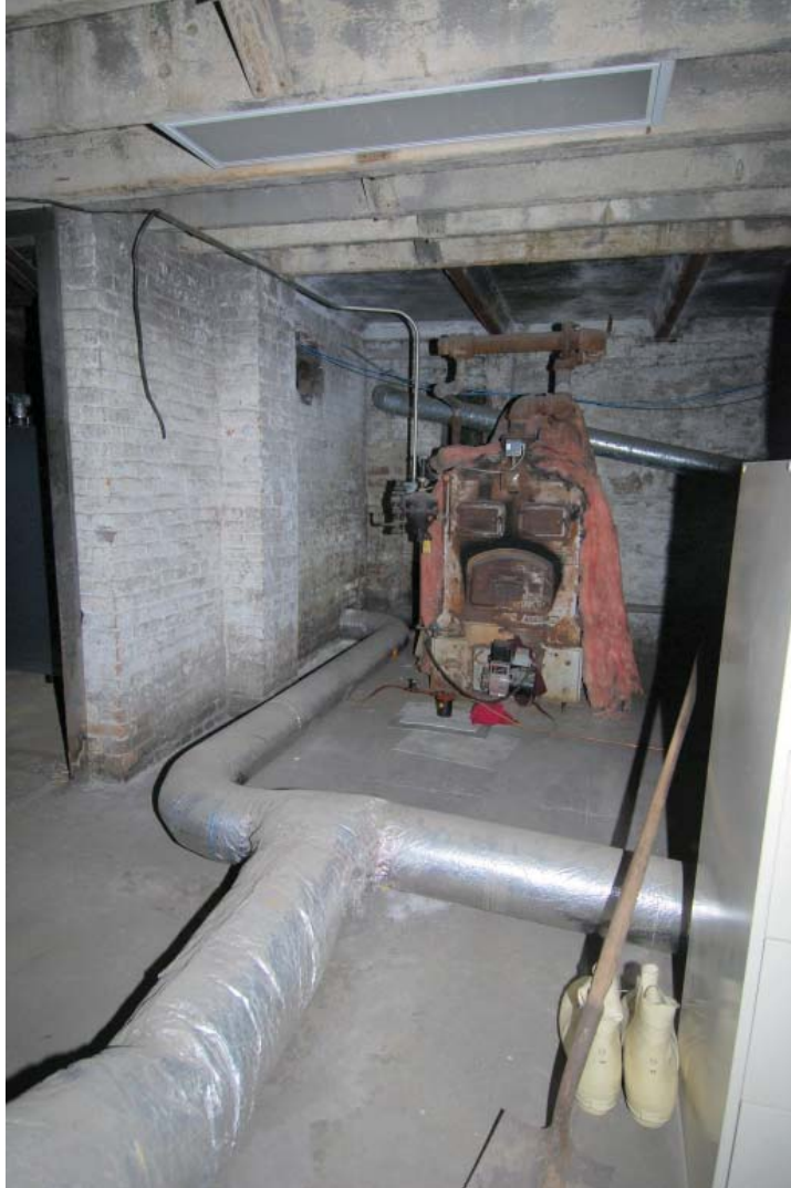
Photo 50. Boiler Room looking northwest. Note old boiler no longer in use (JMA, October 2009).
