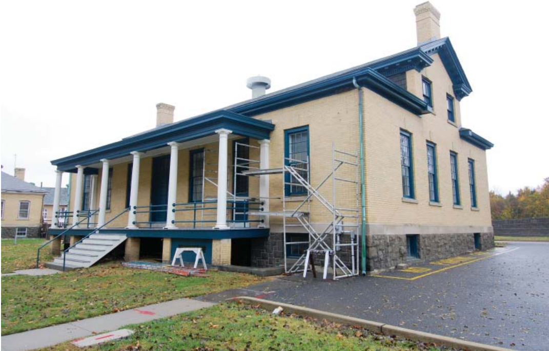
Photo 84. Overall view of Mess Hall Building #58 from the southwest. Note the lack of a continuous path and accessible entrance (JMA, October 2009).
