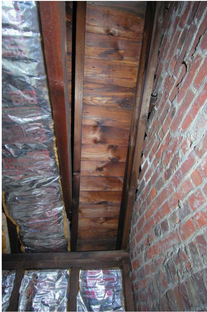
Photo 83. Detail of the underside of the roof at the north dormer end. Note the lack of insulation at the dormer roof. (JMA, October 2009)
