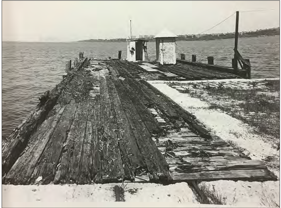
Figure 2.80. Photograph of the dock in disrepair, 1970s (Gateway National Recreation Area Collections).
