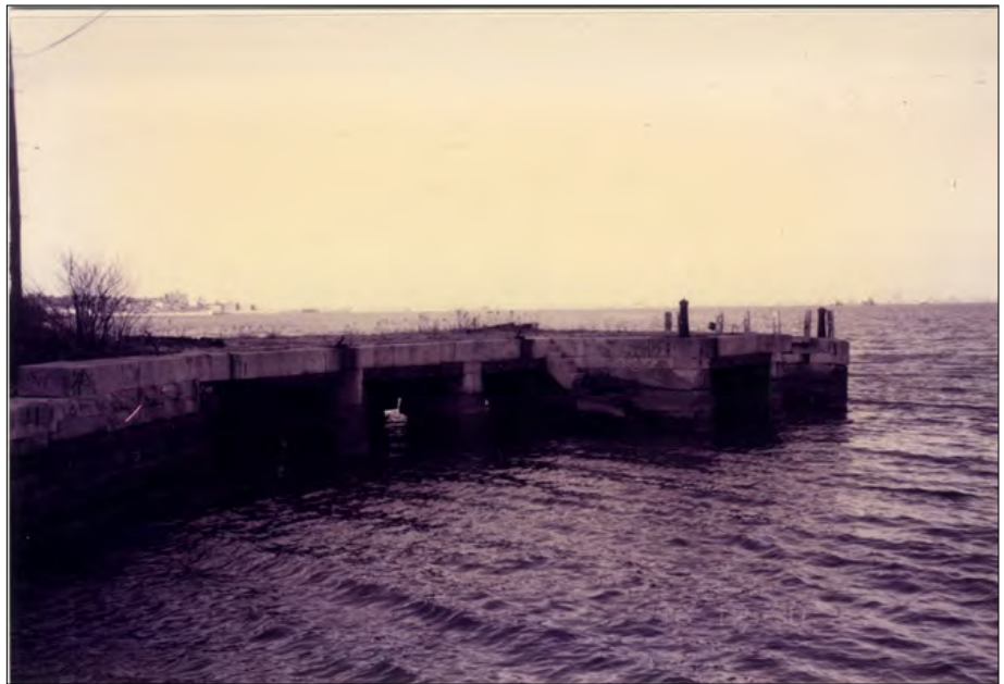
Figure 2.92. Photograph of the dock north of Battery Weed looking north, circa 1995. Note the general state of disrepair with vegetation on the decking, damaged piers, and deteriorating stonework (Gateway National Recreation Area Collections, Image 31082).
