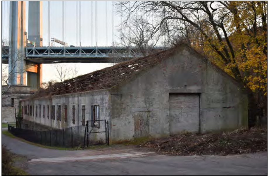
Figure 3.7. Photograph of the Torpedo Storage building, facing southeast from Weed Road. Note the missing roof (PaleoWest 2021).
