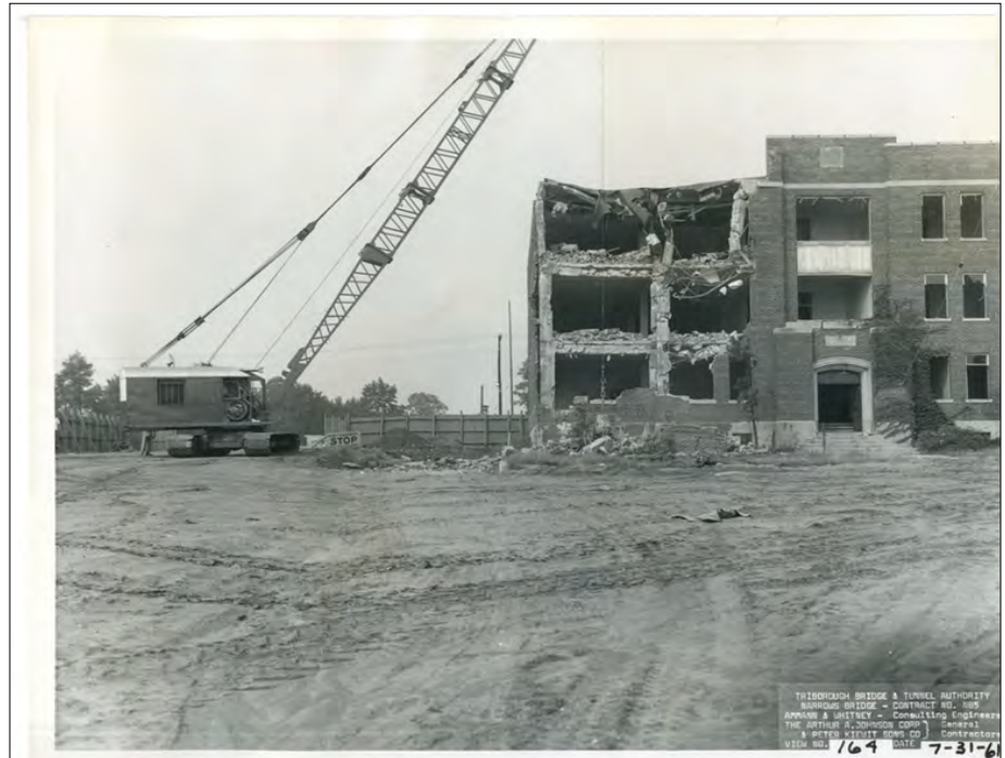
Figure 2.71. Photograph of the demolition of the 1931 Infantry Barracks at the southern end of Building 210, June 1961 (Courtesy of MTA Bridges and Tunnels Special Archive, Photo NB-5-164).
