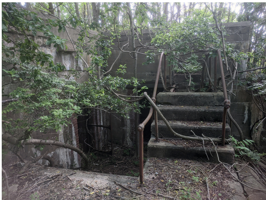
Figure 20. View looking east at overgrown steps, missing catwalk (center right), and damaged railings at Battery Urmston. (OCLP 2020, IMG-093812)
