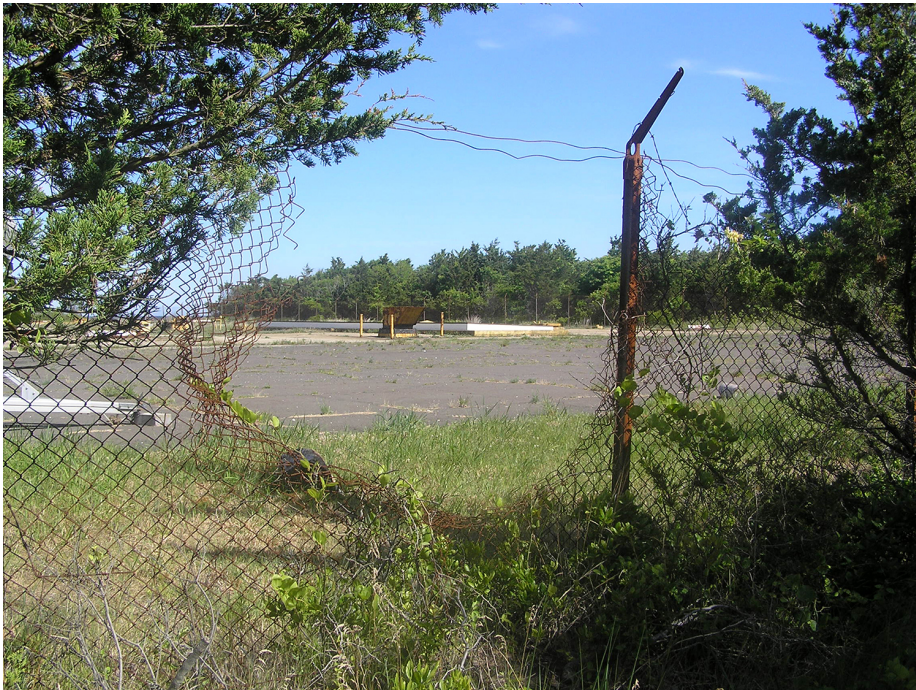
Figure 25. Section of inner fence in poor condition at the missile magazine area, NIKE Launch Site. (OCLP 2020, P1010019)
