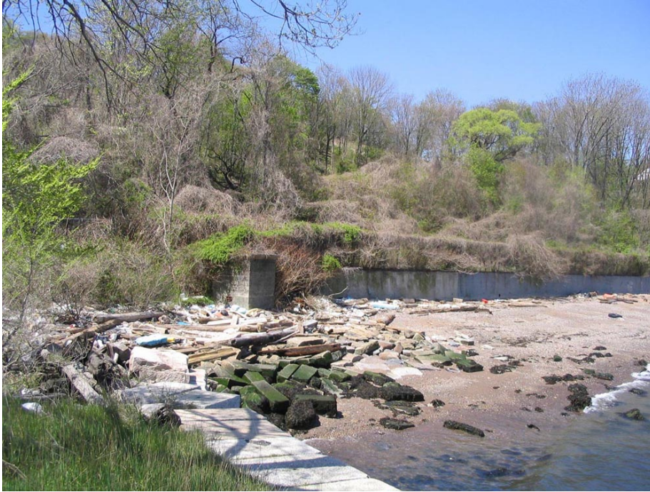
Figure 28. The partially vine-covered concrete seawall (BS-13) built in c.1938, view looking northwest with Battery Catlin in the background. In the foreground is a collapsed section of the granite seawall. (SUNY ESF, 2007)
