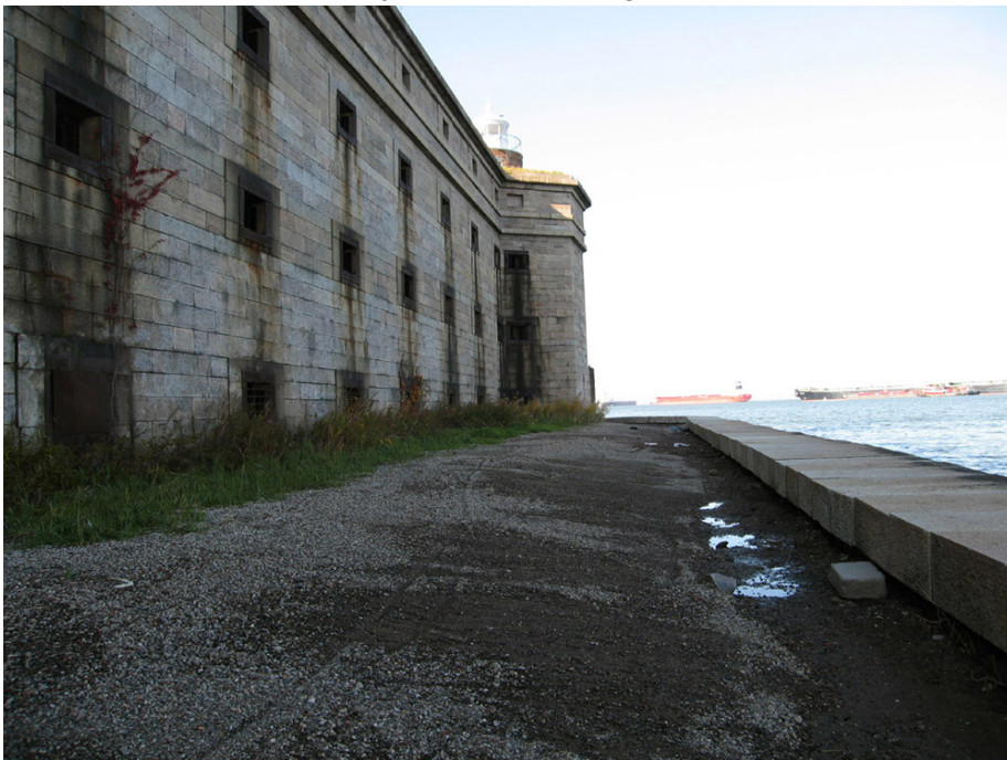
Figure 15. The moat space (SO-2) and waterfront promenade (C-5), looking north, is filled with earth and rubble and top-dressed with gravel between the granite seawall (BS-2) and the fort walls. (SUNY ESF, 2006)
